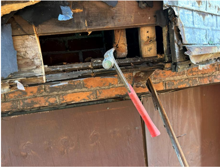
Dry rot condition at end of joist at Altadena Building
