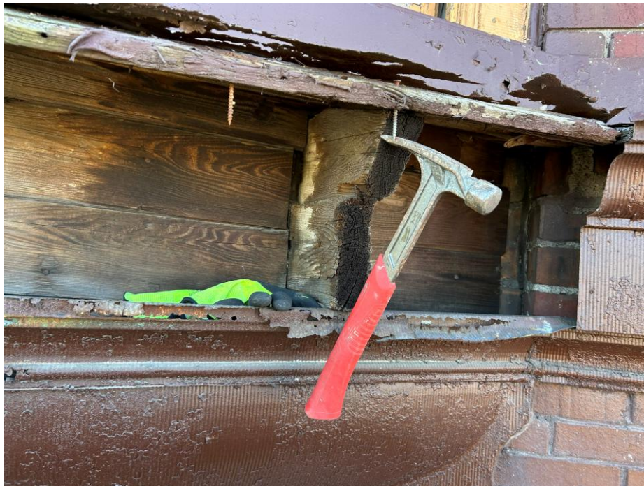
Dry rot condition at end of joist at Manhattan Building
