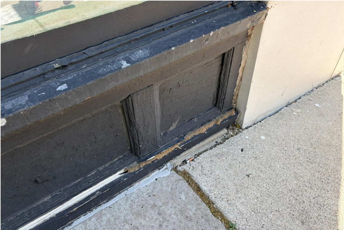
17. Storefront F sill deterioration, North Façade, Looking South.
