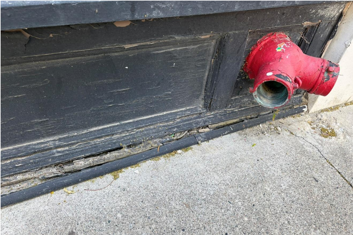
13. Storefront C sill deterioration, North Façade, Looking South.
