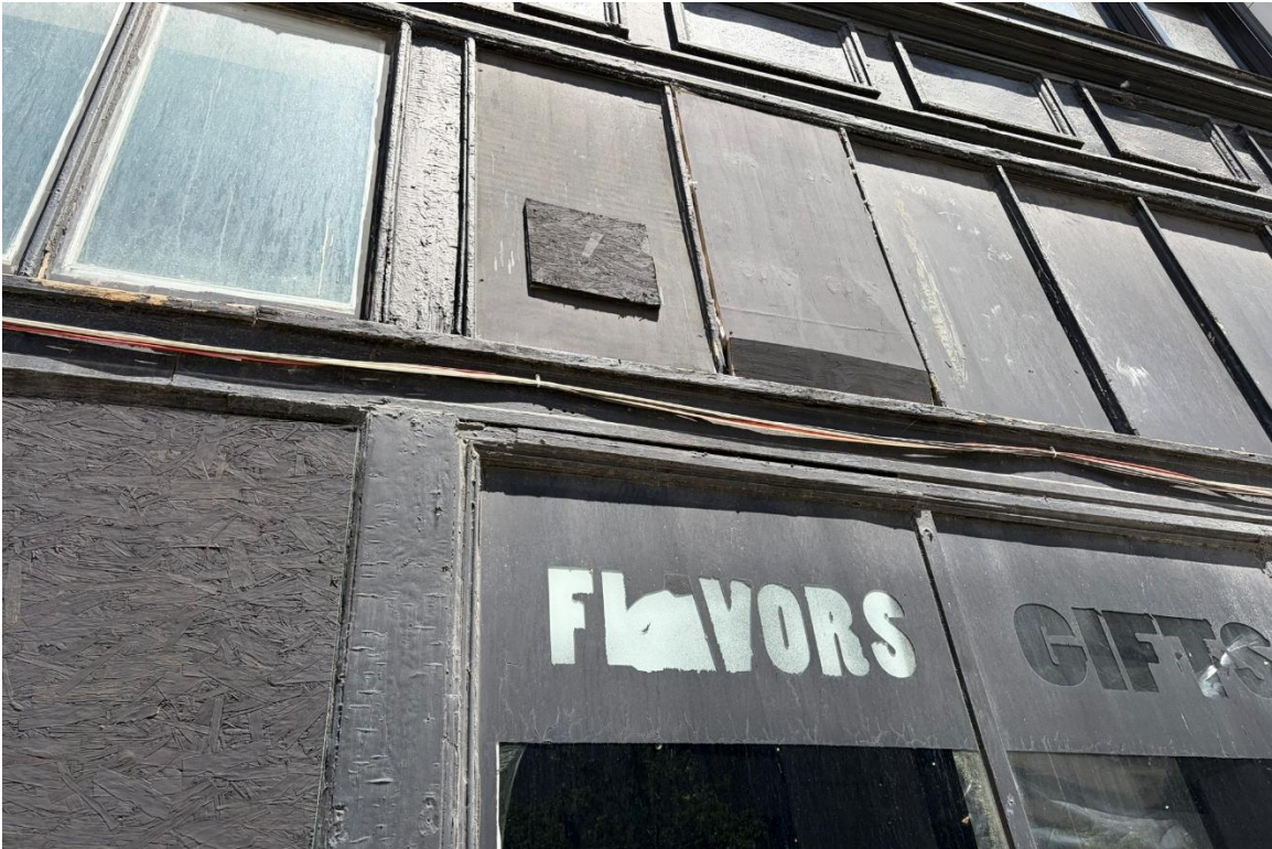
25. Storefront G missing transom panels, West Façade, Looking East.
