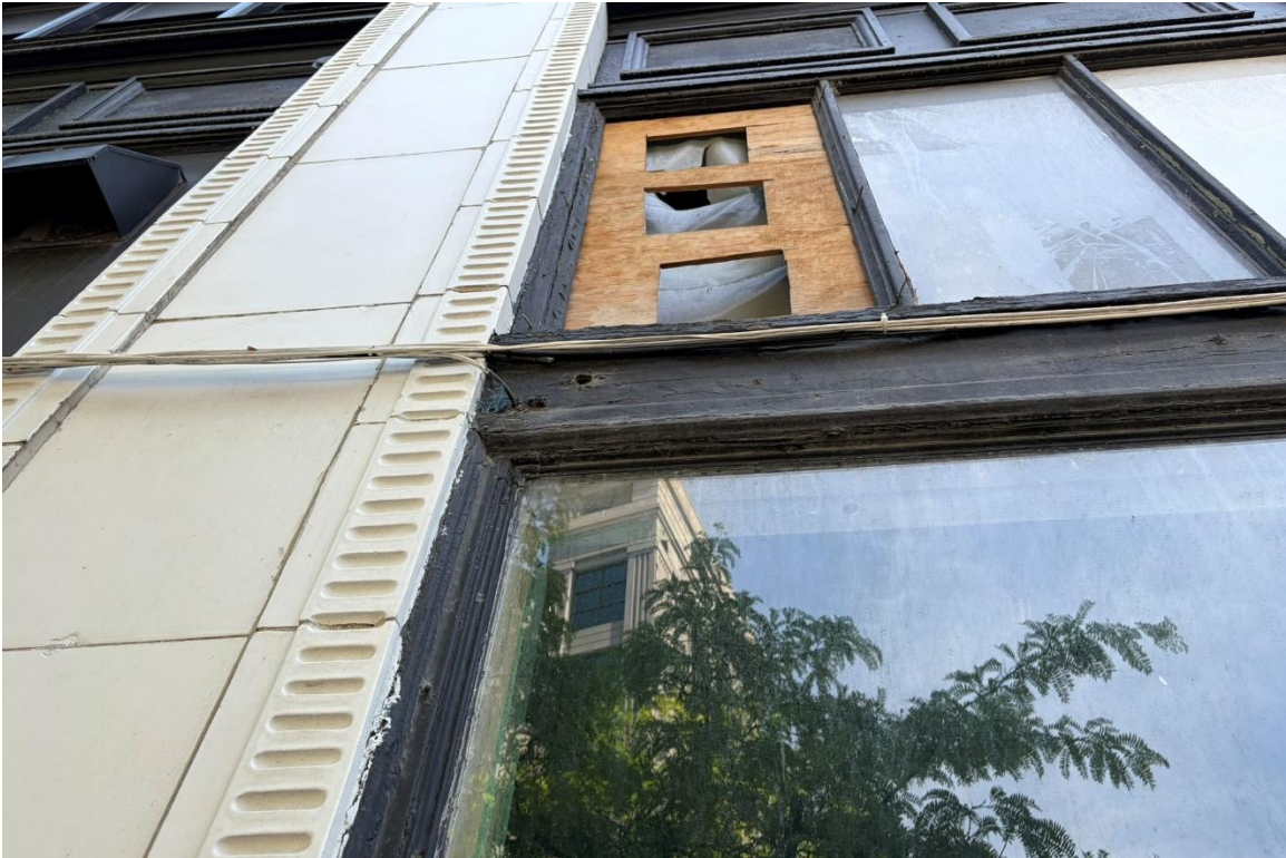
19. Storefront C missing transom panels, North Façade, Looking South. .
