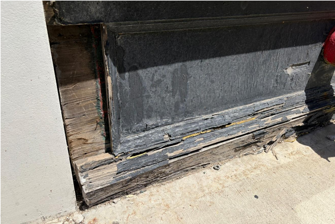
23. Storefront H damaged sill, West Façade, Looking East.
