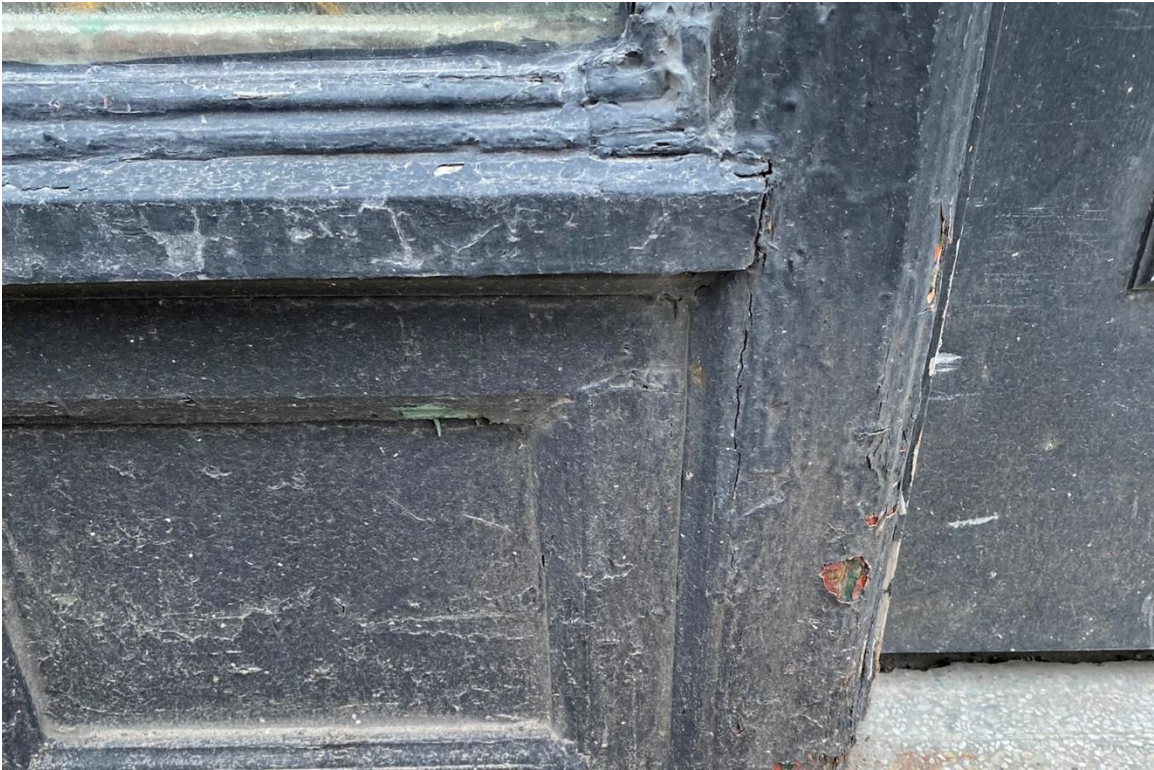
11. Storefront B deteriorated sill, North Façade, Looking South.
