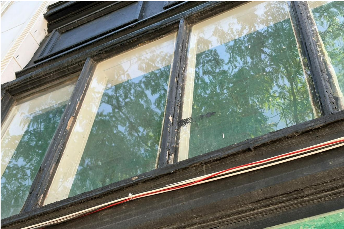
22. Storefront F deteriorated transom, North Façade, Looking South.
