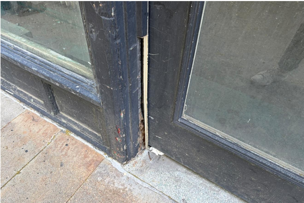
20. Storefront B damaged door trim, North Façade, Looking South.
