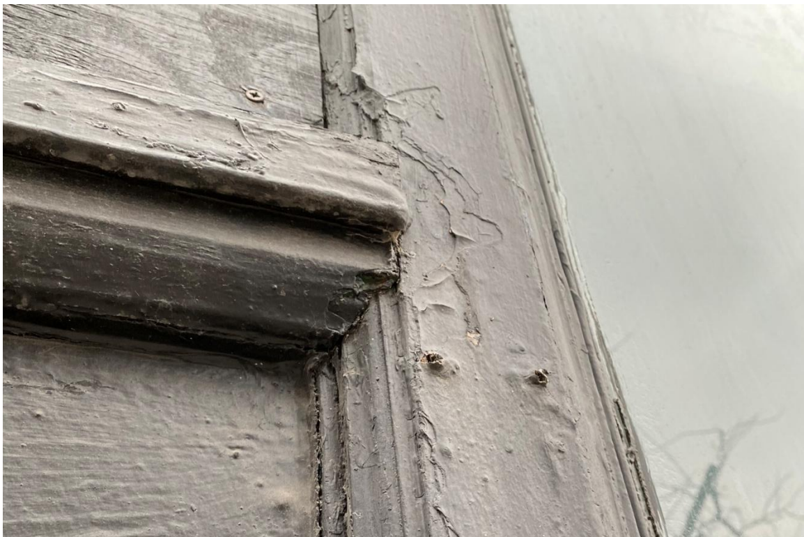
12. Storefront B deterioration, North Façade, Looking South.
