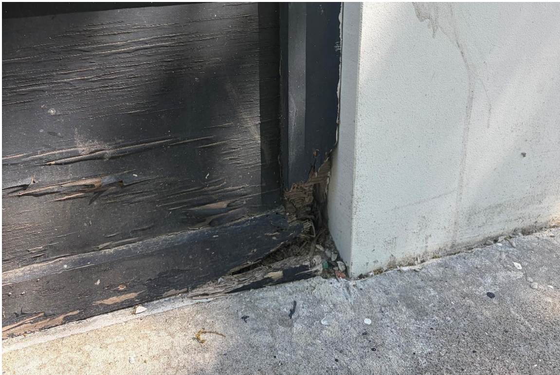
18. Storefront E sill damage, North Façade, Looking South.
