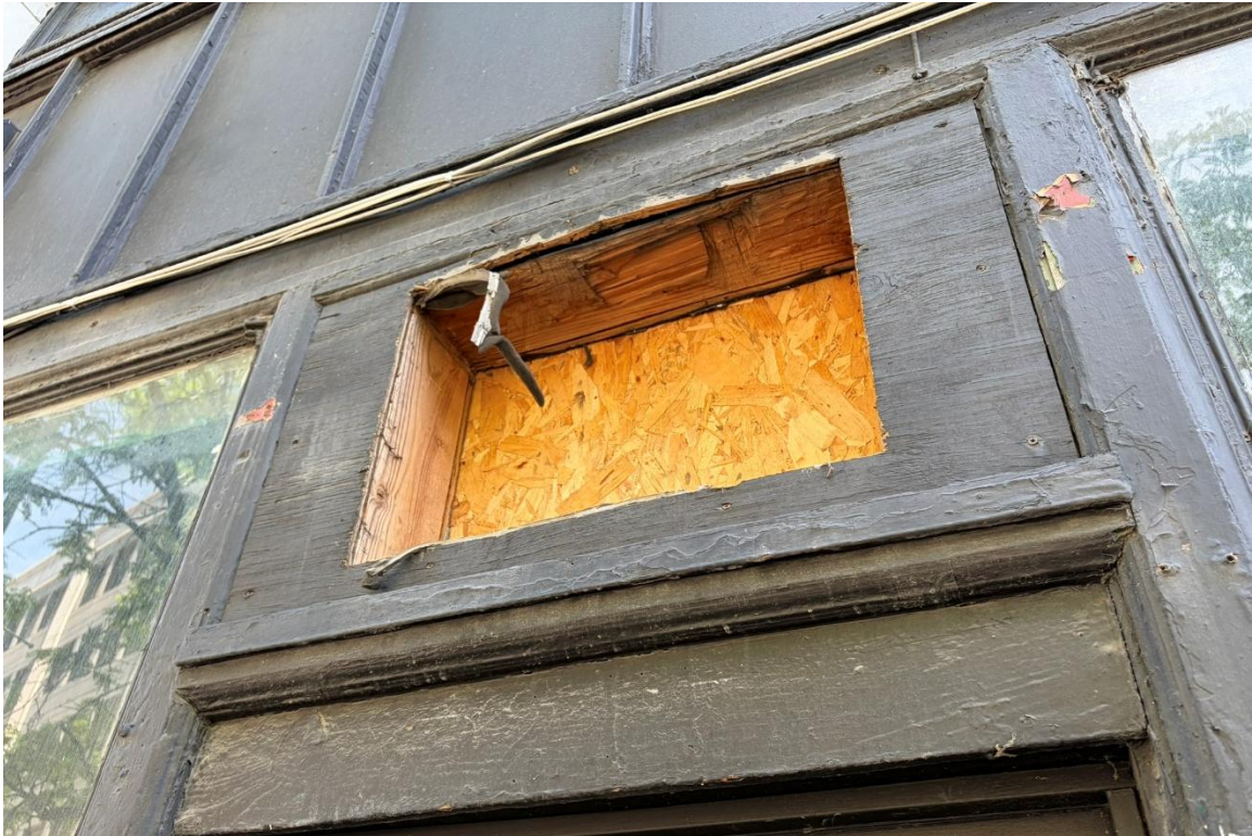
9. Storefront B missing transom, North Façade, Looking South.
