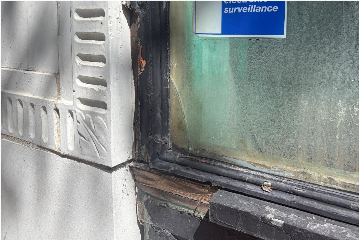
15. Storefront B damaged wood sill, North Façade, Looking South.
