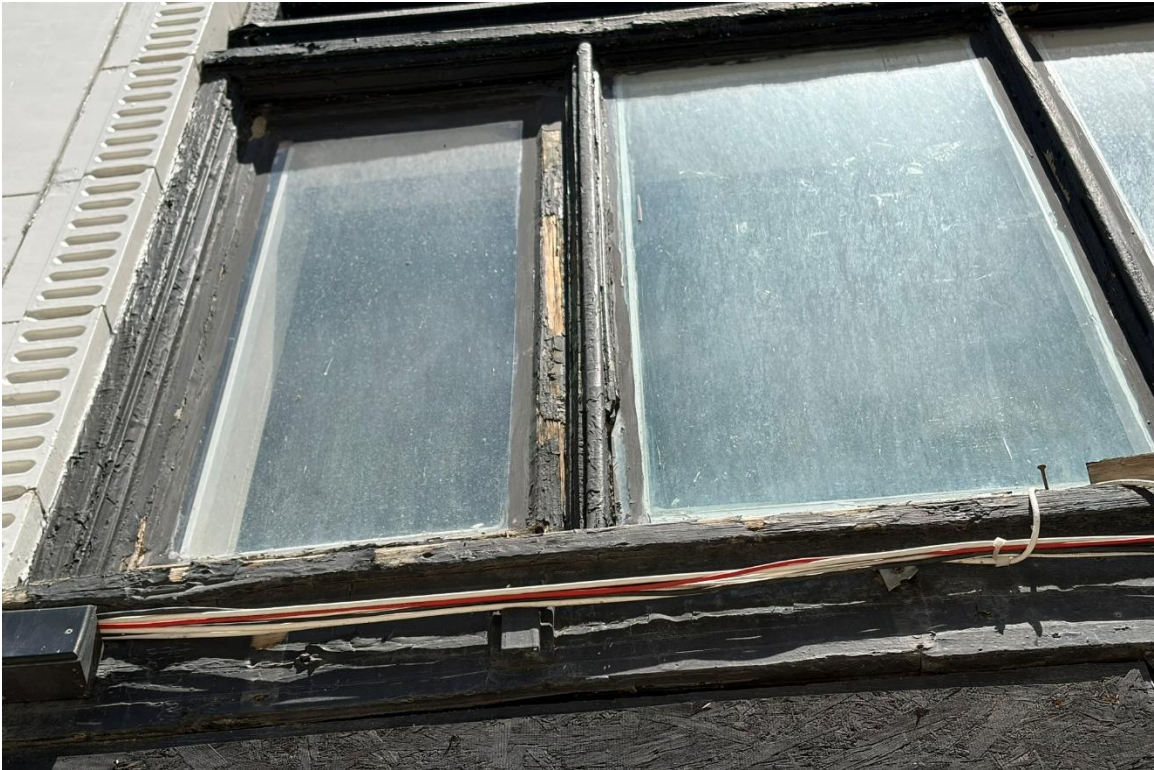
21. Storefront G deteriorated transom, West Façade, Looking East.
