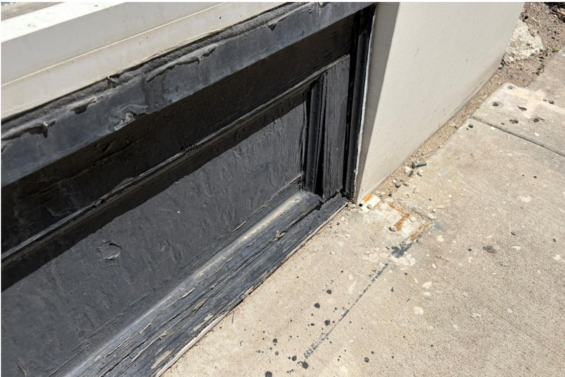
26. Storefront H sill deterioration, West Façade, Looking East.
