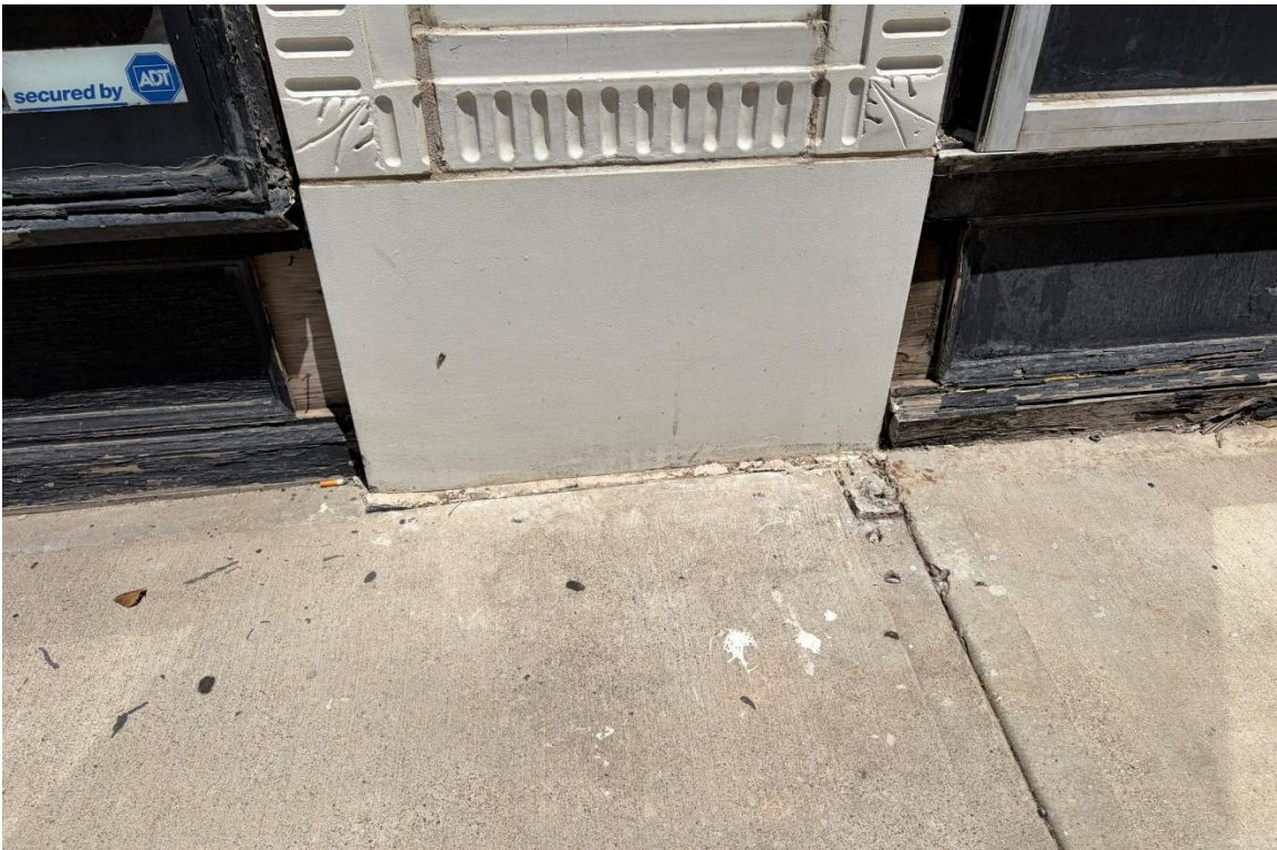
24. Storefront G and H sill damage at column, West Façade, Looking East.
