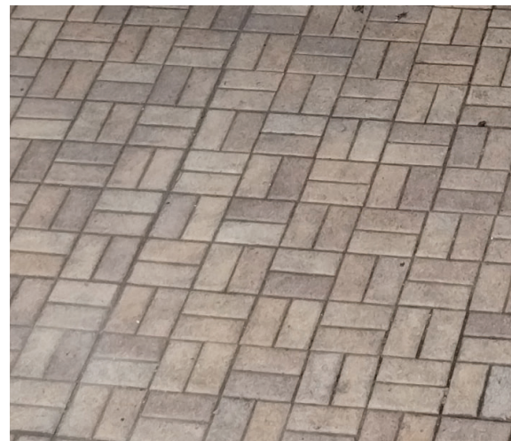
ENTRY FLOOR TILES: The existing historic tiles at the recessed entrances will remain with repairs with matching tiles, infill grouting and gentle cleaning.
