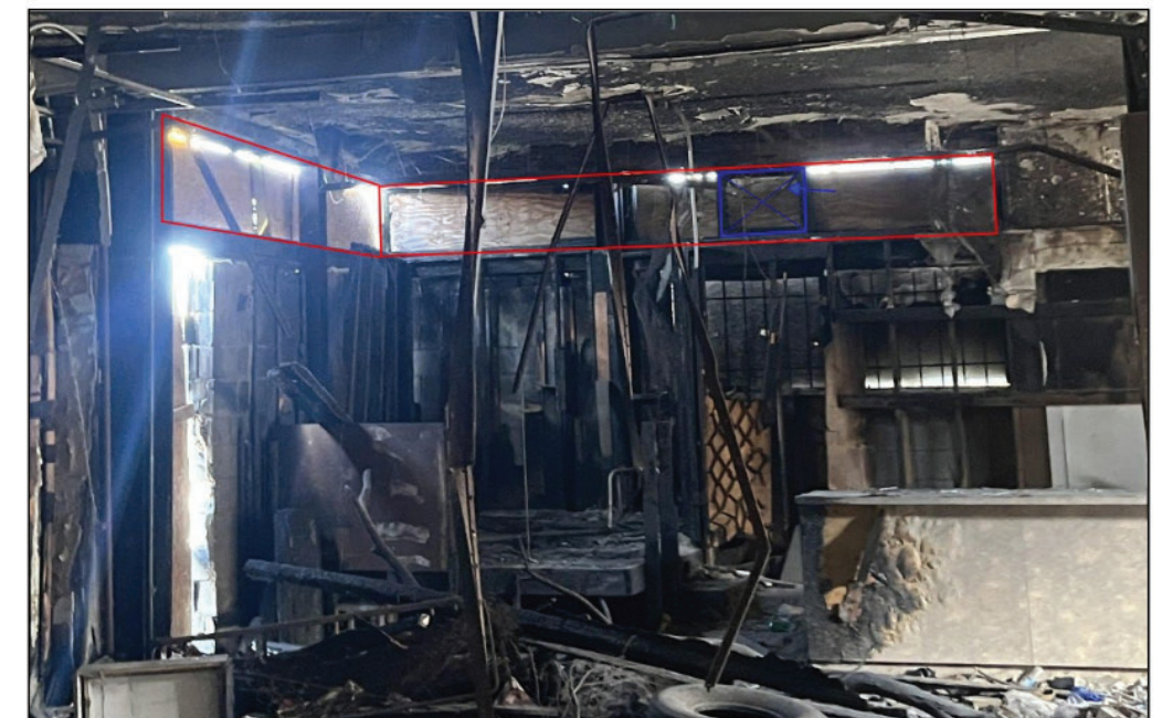
Figure 23. Transom window framing and a fragment of the X mullion that remain at the corner storefront.
