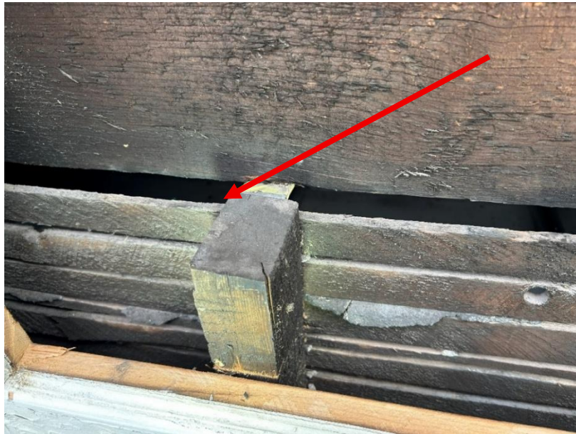
Photo 3: Interior condition at second northern bay window assembly. Metal support clip indicated with red arrow.
