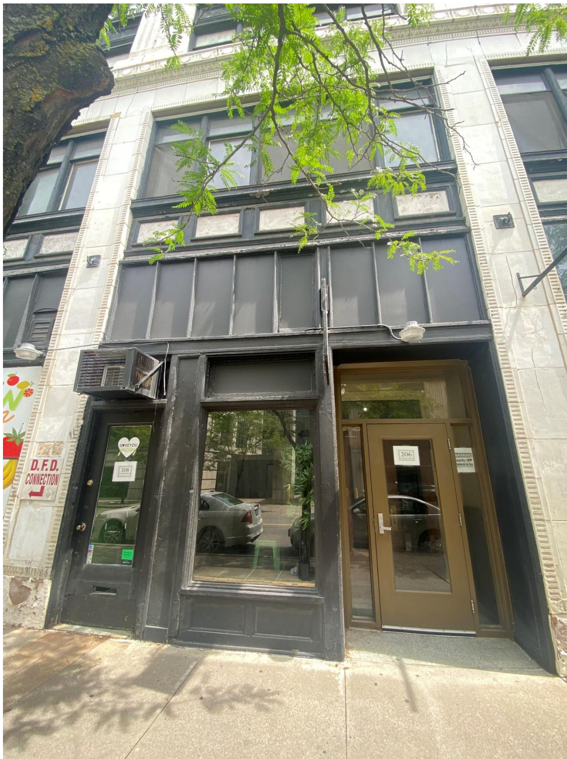
5. Exterior, North Elevation, Looking South. c. 2022. Location of historic canopy, tieback connections still on façade.
