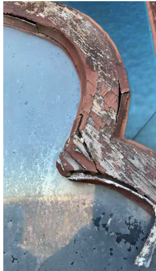
Detail view of existing historic wood tracery, typical condition.
