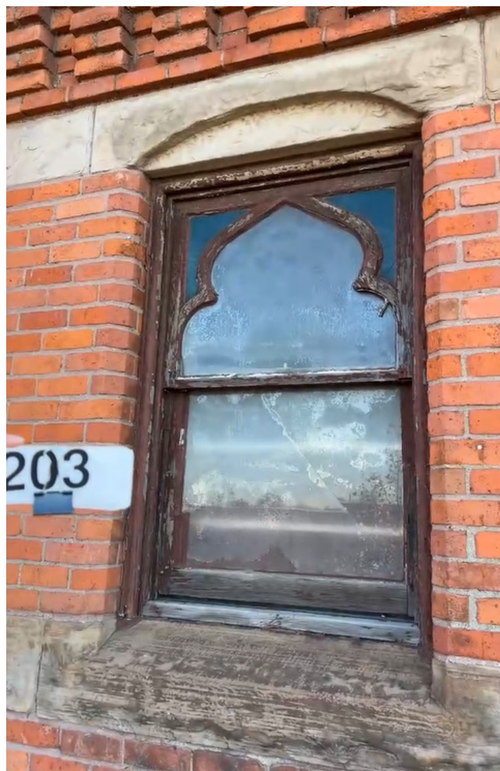
View of existing historic wood window #203 at Basilica (sacristy), 2nd floor, west elevation.
