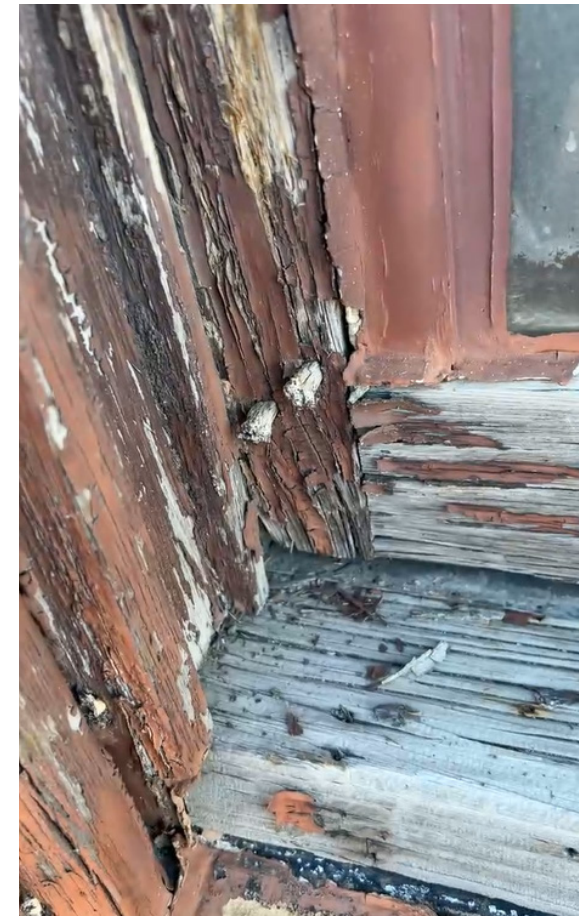
Detail view of existing historic wood sill, frame, and lower sash components, typical condition.
