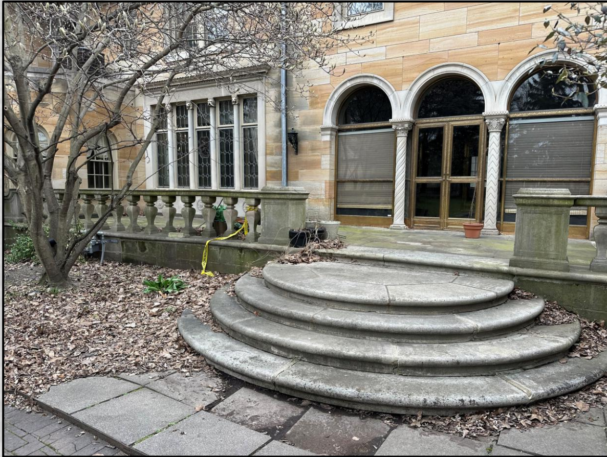
Upper terrace and staircase is original. There are some pieces that broke and replaced with concrete in flatwork areas.
