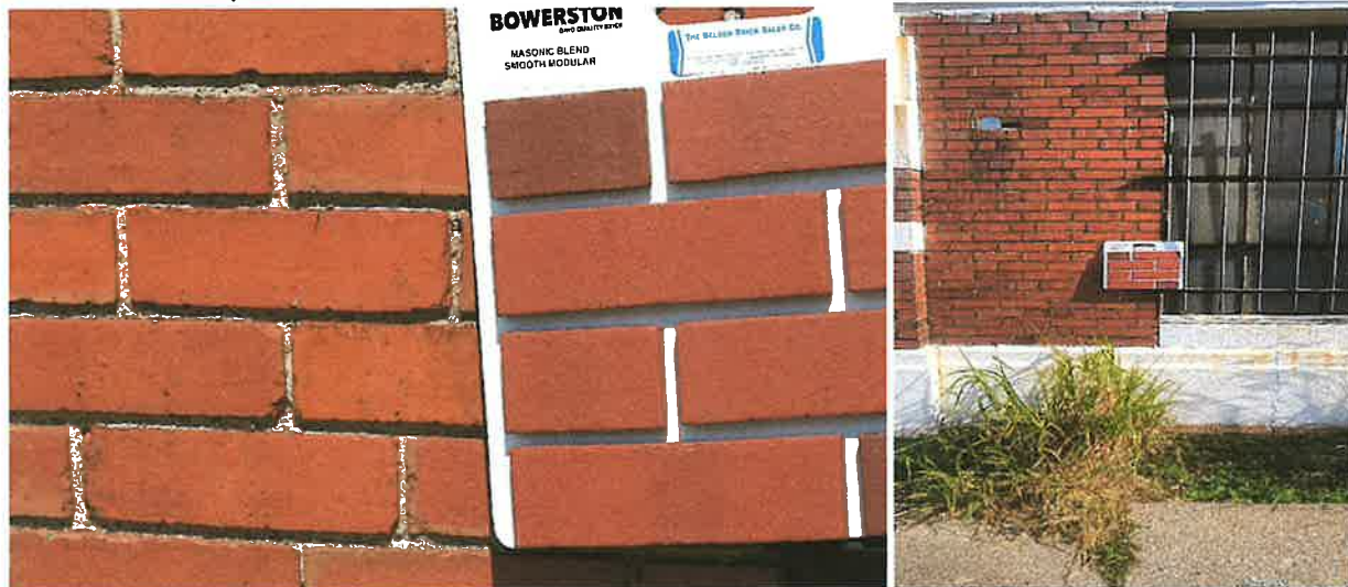
Photo 1 above approx. 2ft away with existing brick being cleaned using One Restore cleaner on 4/23/26 Photo 2 above approximately 12ft away brick hasn't been cleaned. (Earlier Photo)
