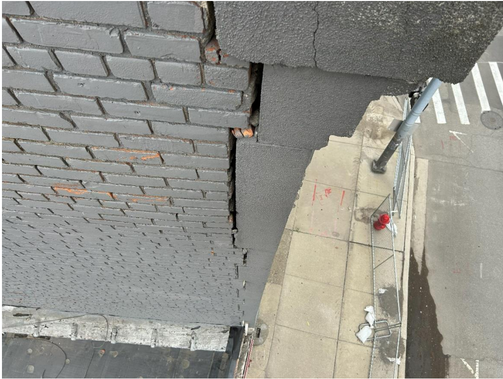
Photo 6: Unbonded brick façade at building corner
