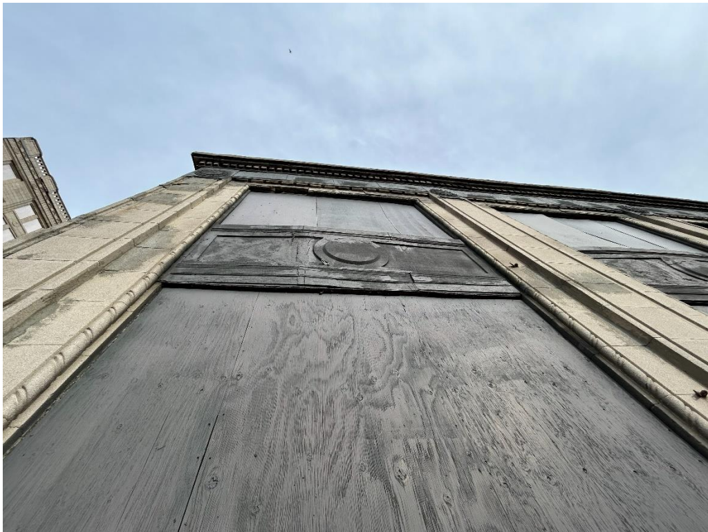
Photo 3: Debonded decorative spandrel component
