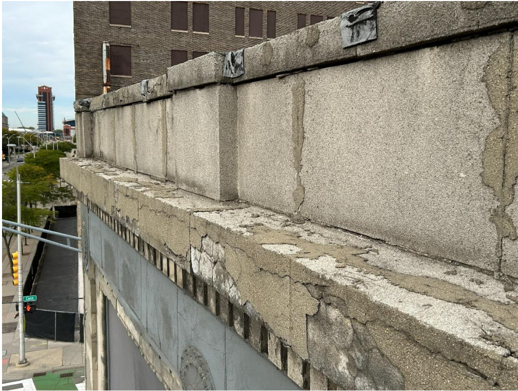
Photo 2: Damaged Cornice component
