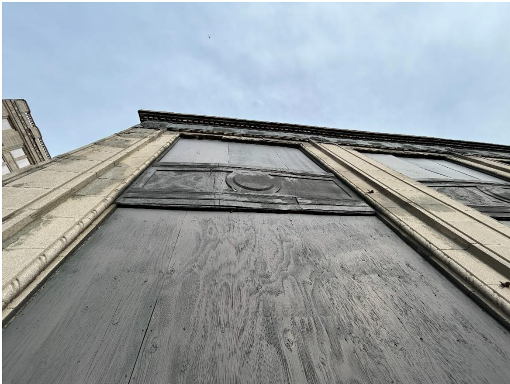
Photo 3: Debonded decorative spandrel component
