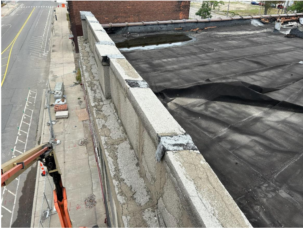
Photo 4: Out of plumb parapet wall
