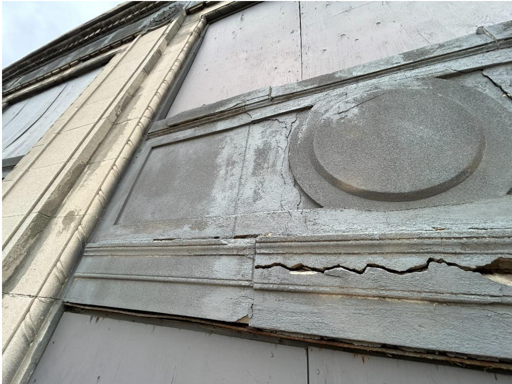
Photo 7: Damaged spandrel and header components
