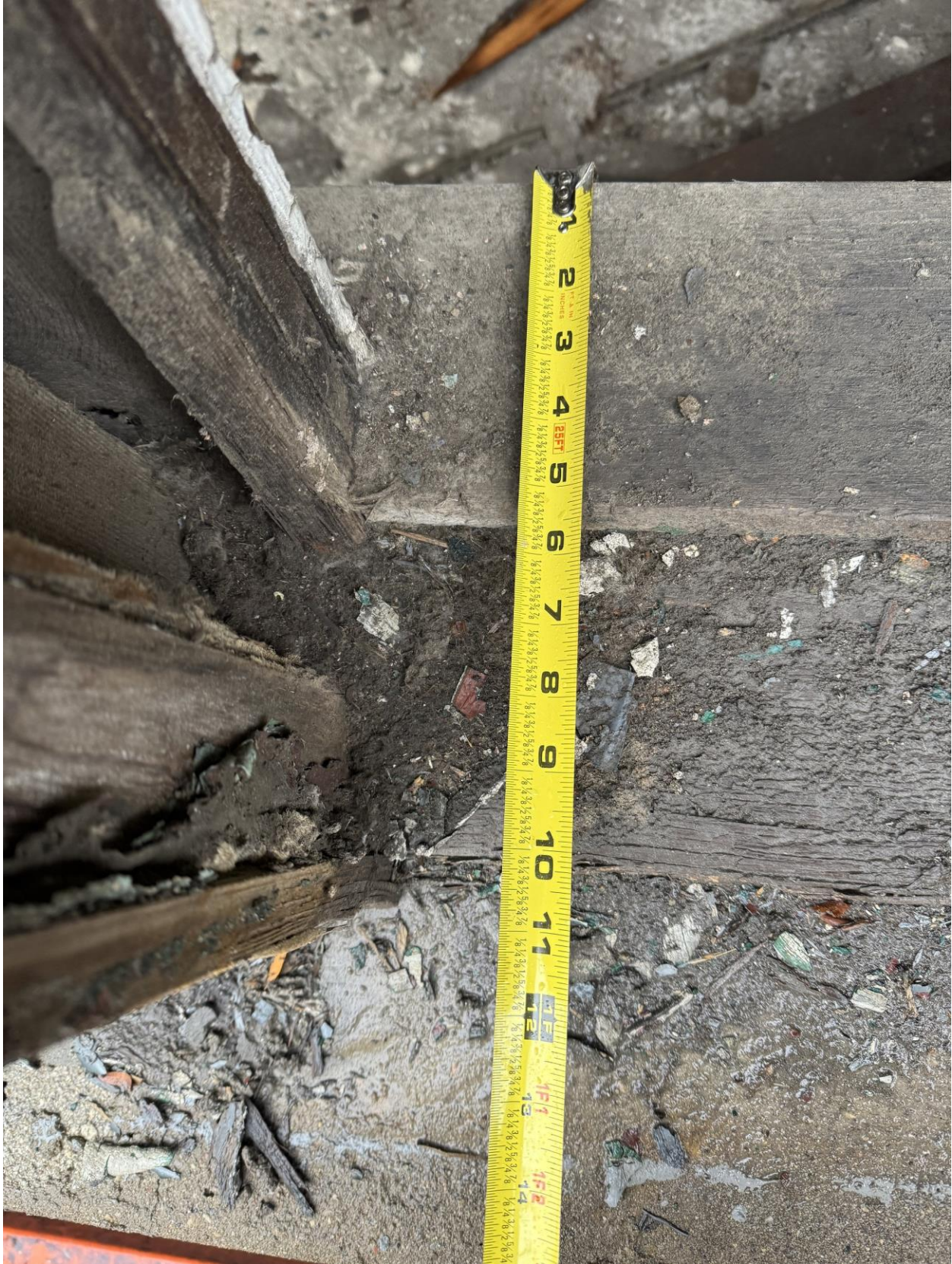
Photo W16 (Sill)
