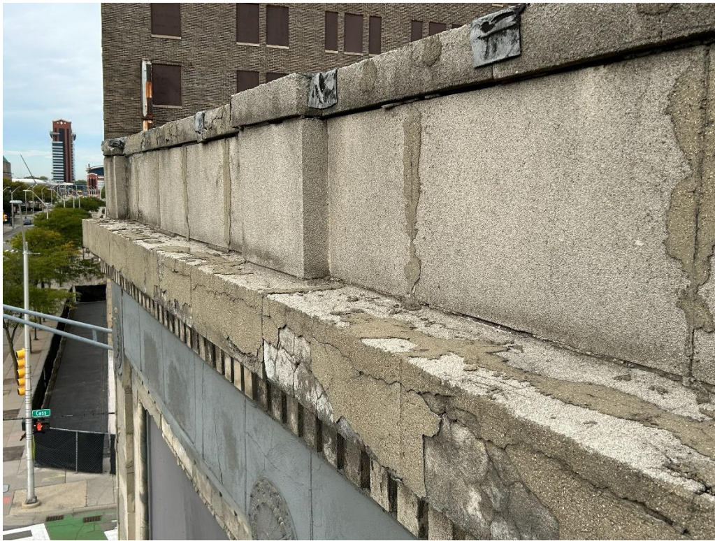
Photo 2: Damaged Cornice component
