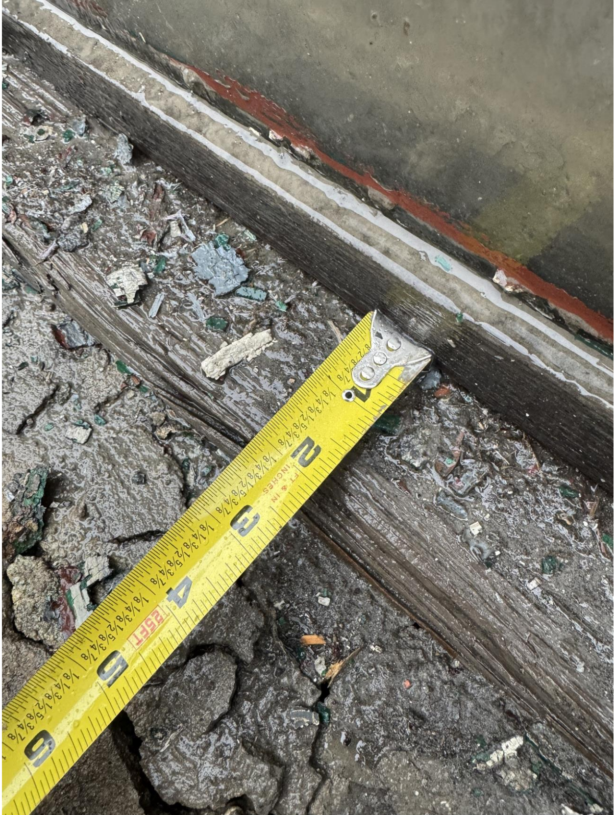
Photo W15 (Sill)
