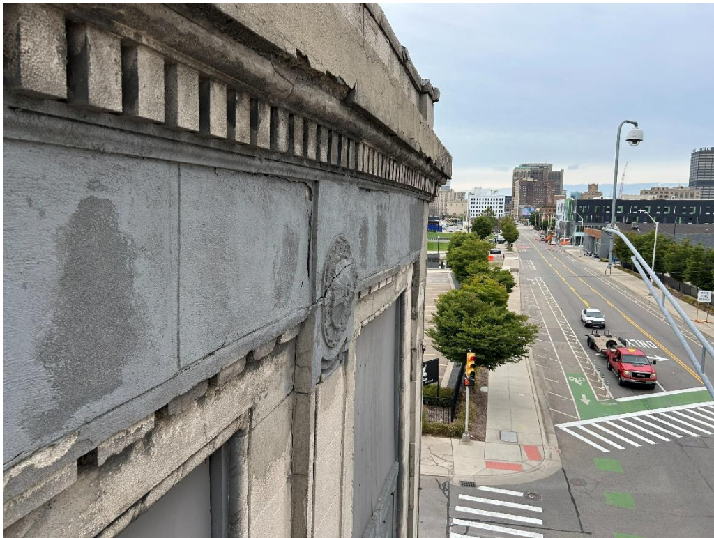
Photo 5: Damaged concrete panels and cornice components
