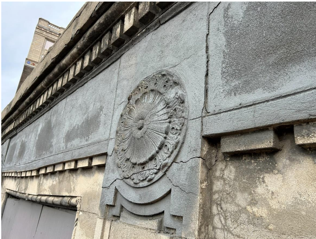
Photo 1: Unbonded/damaged decorative panel
