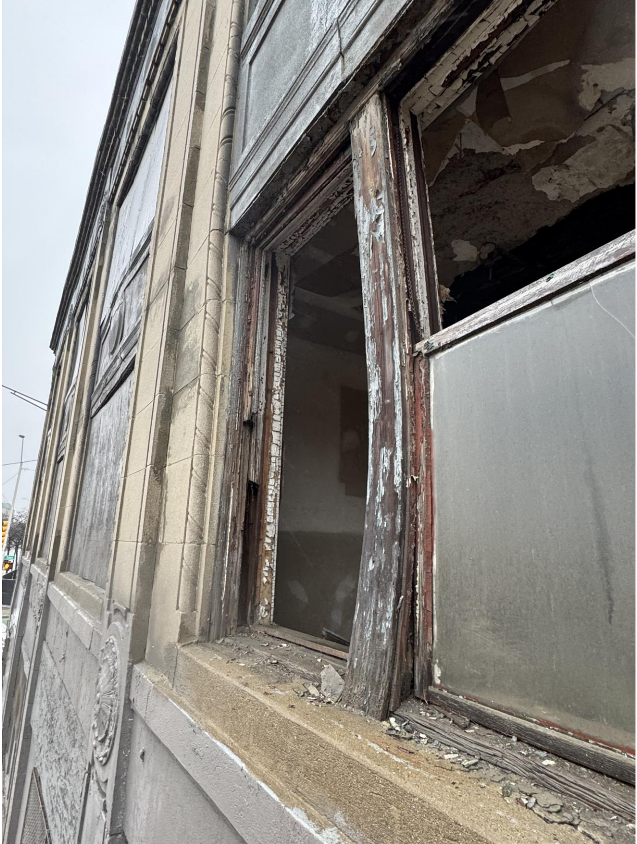
Photo W1 (Left & Center Windows)
