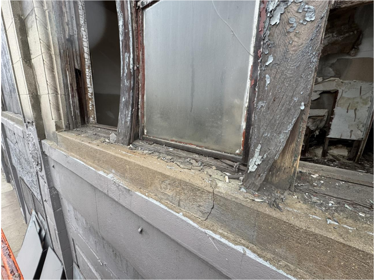
Photo W4 (Left & Center Windows – Sill & Lower Sash Opening)
