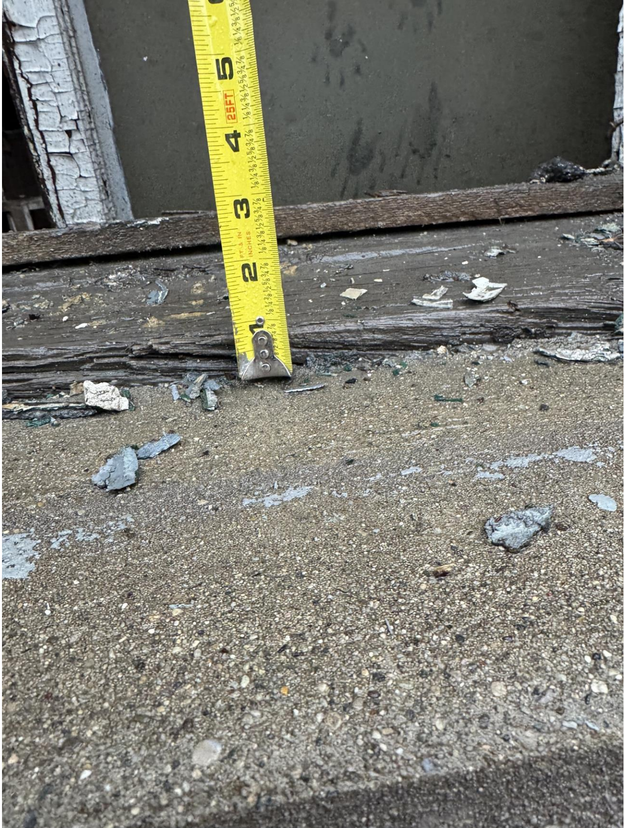
Photo W17 (Sill)
