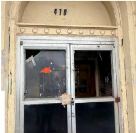
Existing damaged double entry door
