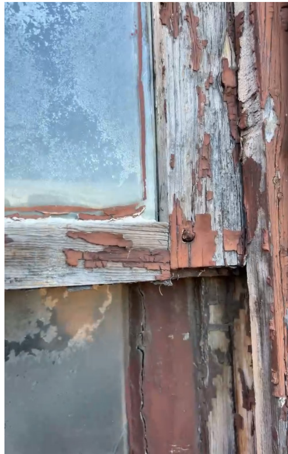
Detail view of existing historic wood upper sash components and frame, typical condition.
