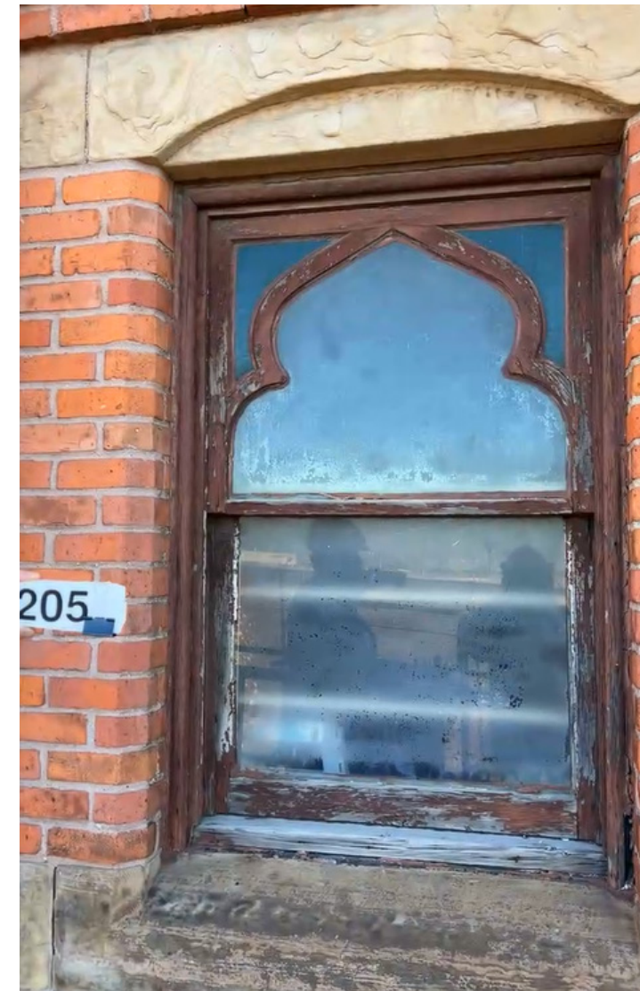
View of existing historic wood window #205 at Basilica (sacristy), 2nd floor, west elevation.
