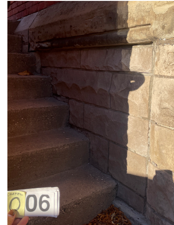
FOR REFERENCE: View of existing historic masonry opening #006 at Basilica/chapel. Previously infilled with stone; north of #005 at west elevation.
