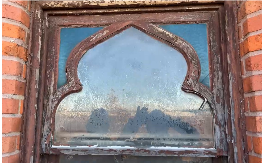
Detail view of existing historic wood upper sash and frame, typical condition.
