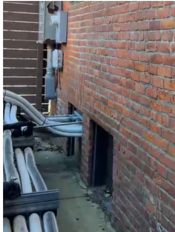
FOR REFERENCE: View of masonry openings #006 and #007 at Wellness Center/Convent, north elevation. Concealed from view by existing screen/fence.
