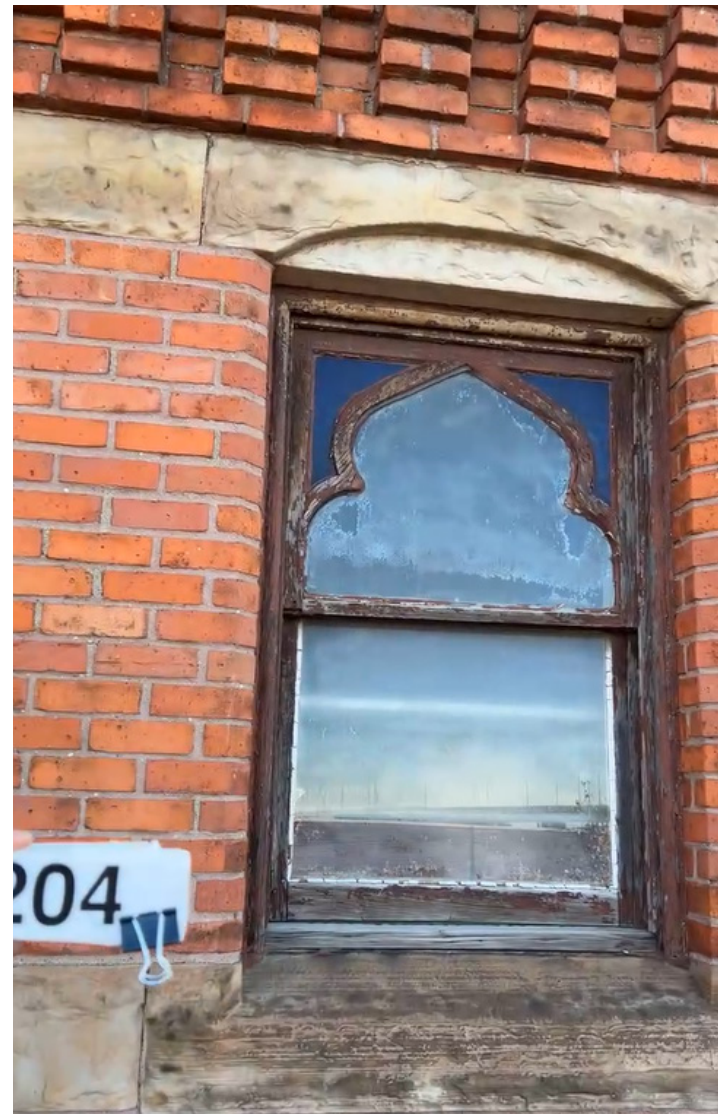
View of existing historic wood window #204 at Basilica (sacristy), 2nd floor, west elevation.
