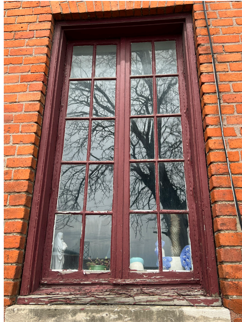
View of existing historic wood window #104 at Rectory, 1st floor, south elevation.
