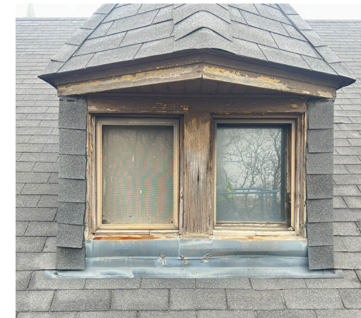
View of existing historic wood window #400A/B at Rectory, roof dormer, south elevation.
