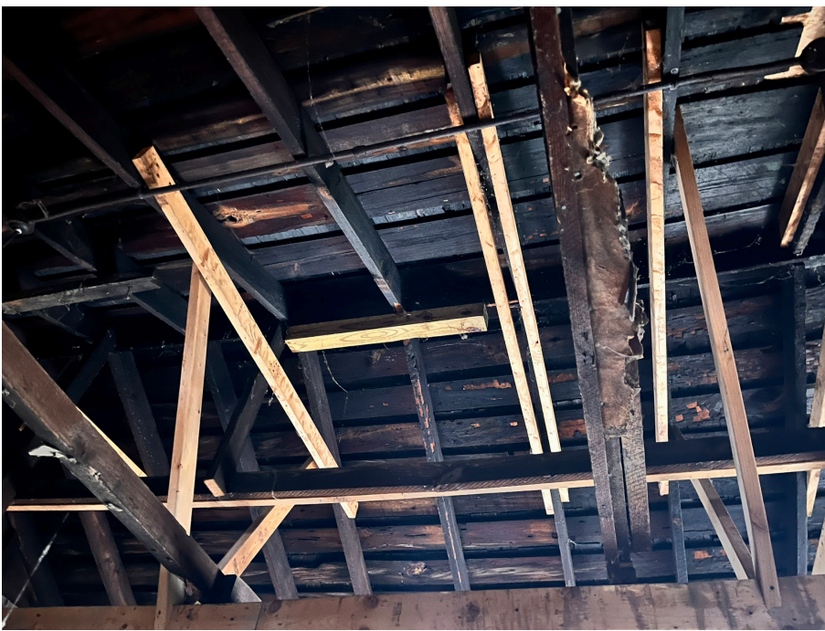
IMAGE 18: TEMPORARY SISTER SUPPORTS FOR EXISTING RAFTERS - UNKNOWN WOOD CONDITION DUE TO LONGTERM WEATHER EXPOSURE
