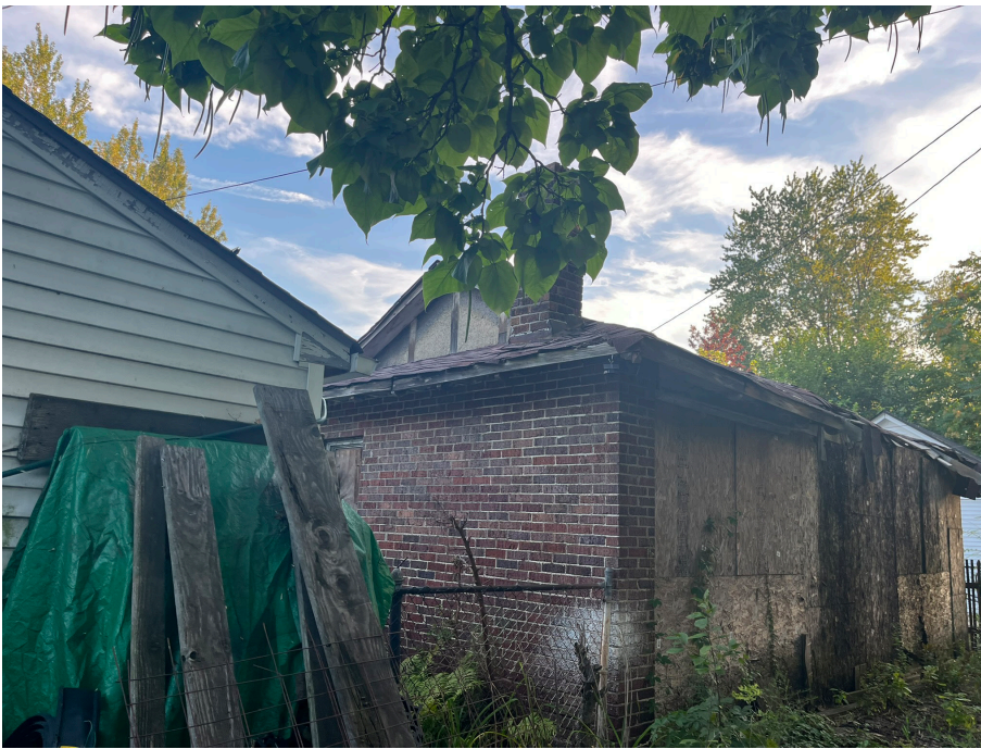
IMAGE 09: EAST ELEVATION SMALL GABLE AT BOTH SIDES WITH STUCCO AND BEAM DETAILING
