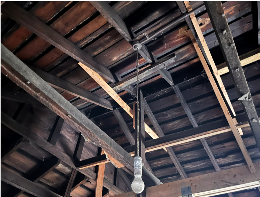
IMAGE 17: RAFTER SHORING IN MULTIPLE LOCATIONS - LIGHT AND CONDUIT ARE NON-FUNCTIONAL
