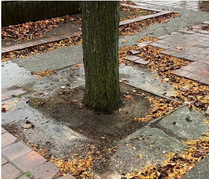
DEGRADED TREE PIT
