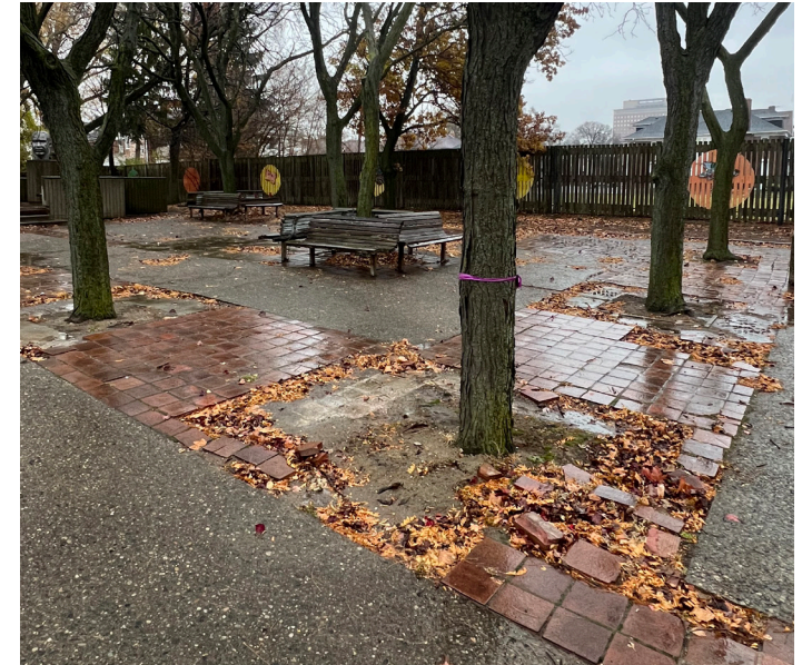
DEGRADED TREE PIT
