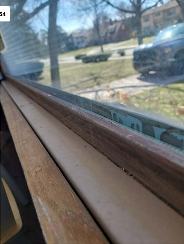
1100-Mold, water damage, broken seals, condensation inside of glass
