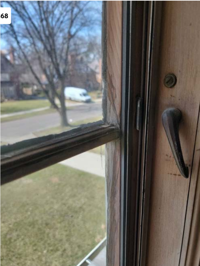
3200- water damage, mold, broken seals, hardware is non functioning, window does not open, condensation between glass, decayed wood between glass
