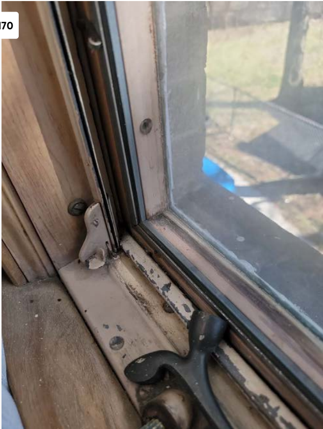
1700- water damage, mold, broken seals, hardware is non functioning, window does not open, condensation between glass, decayed wood between glass
