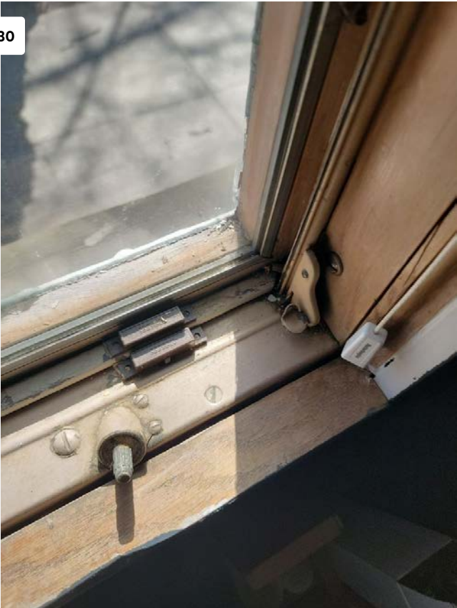
1400-Mold and water damage, broken seals, hardware in nonfunctional, window does not open
