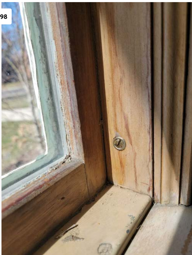
600-Mold, water damage, broken seals, decayed wood inside of glass, condensation inside of glass
