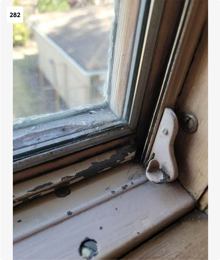
2300- water damage, mold, broken seals, hardware is non functioning, window does not open, condensation between glass, decayed wood between glass
