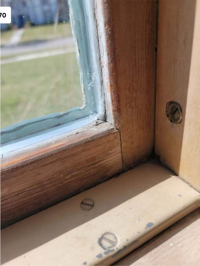
800-Mold, water damage, broken seals, decayed wood inside of glass, condensation inside of glass
