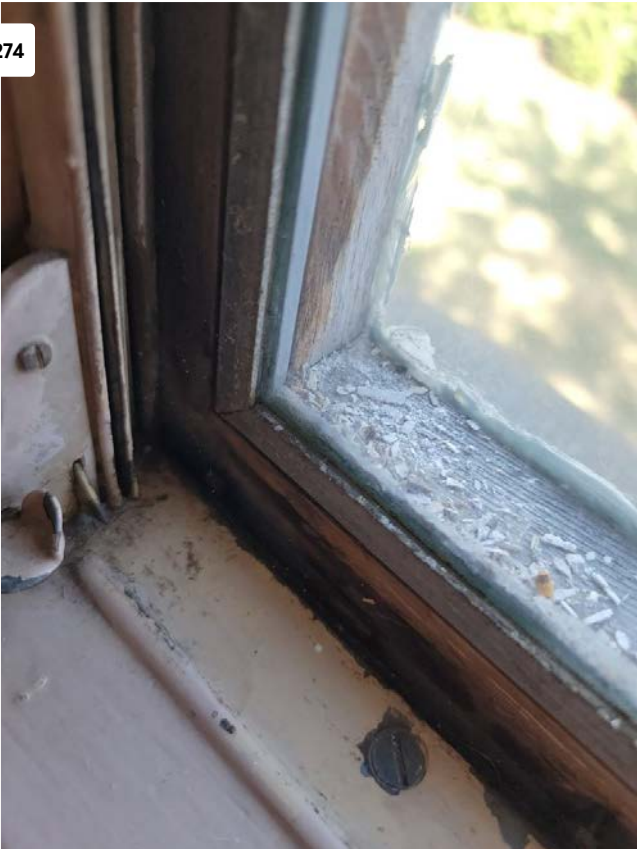
2200- water damage, mold, broken seals, hardware is non functioning, window does not open, condensation between glass, decayed wood between glass, bugs between glass
