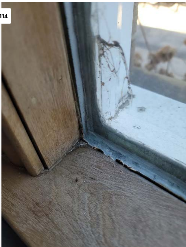
400-Mold, water damage, broken seals, decayed wood inside of glass, condensation inside of glass
