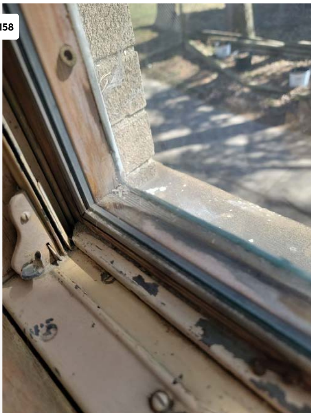
1600- water damage, mold, broken seals, hardware is non functioning, window does not open, condensation between glass, decayed wood between glass
