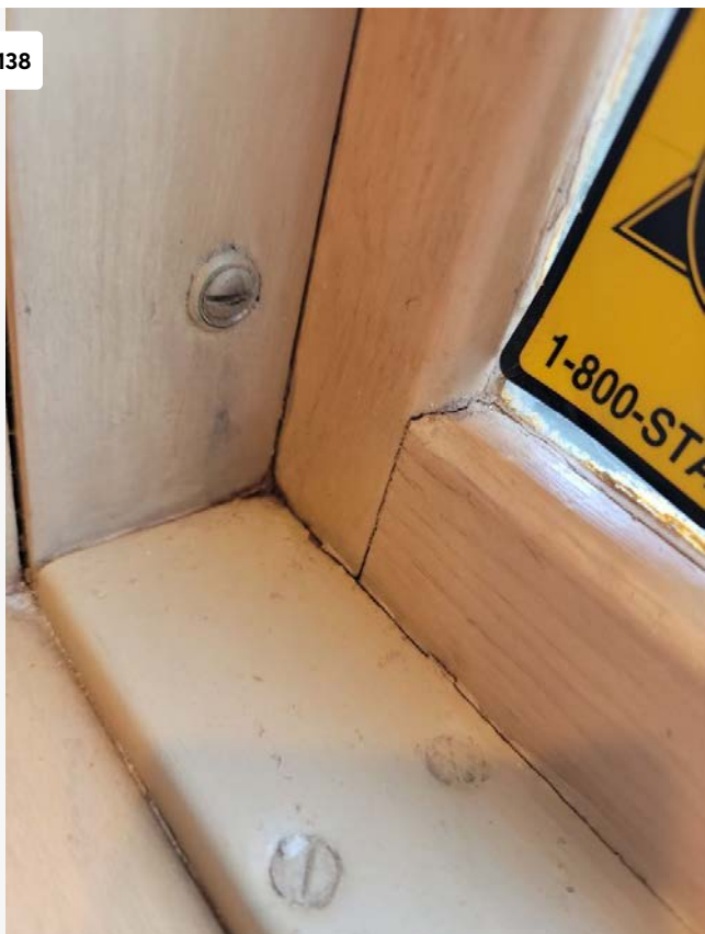
200- Broken frame, cracked seals, water damage, mold, decayed wood inside of glass, condensation in between glass
