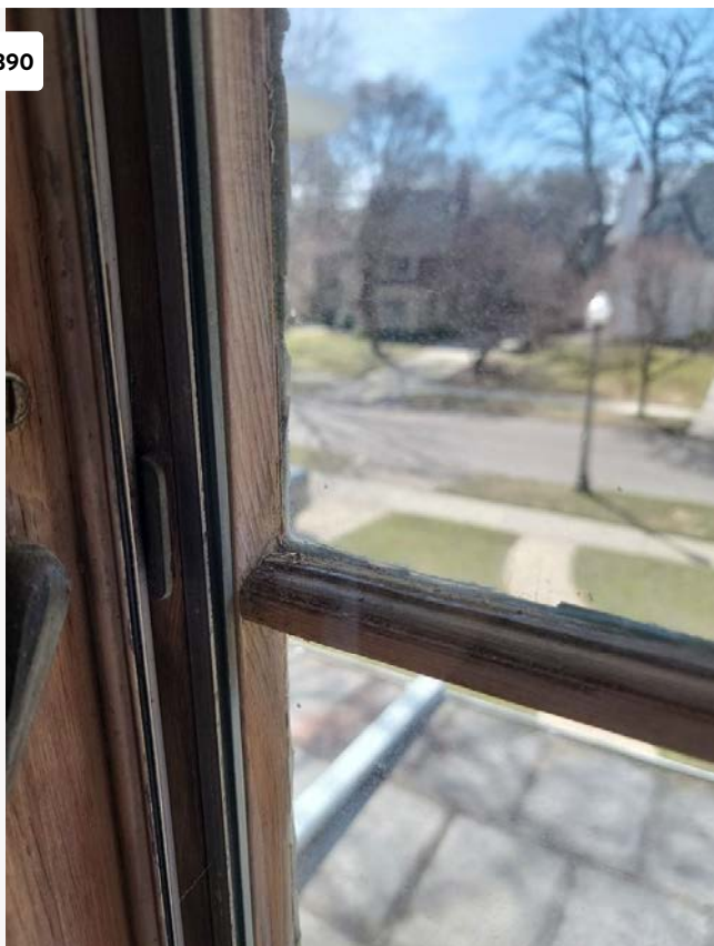
3300- water damage, mold, broken seals, hardware is non functioning, window does not open, condensation between glass, decayed wood between glass
