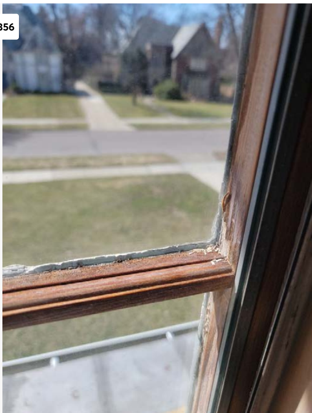
3000- water damage, mold, broken seals, hardware is non functioning, window does not open, condensation between glass, decayed wood between glass
