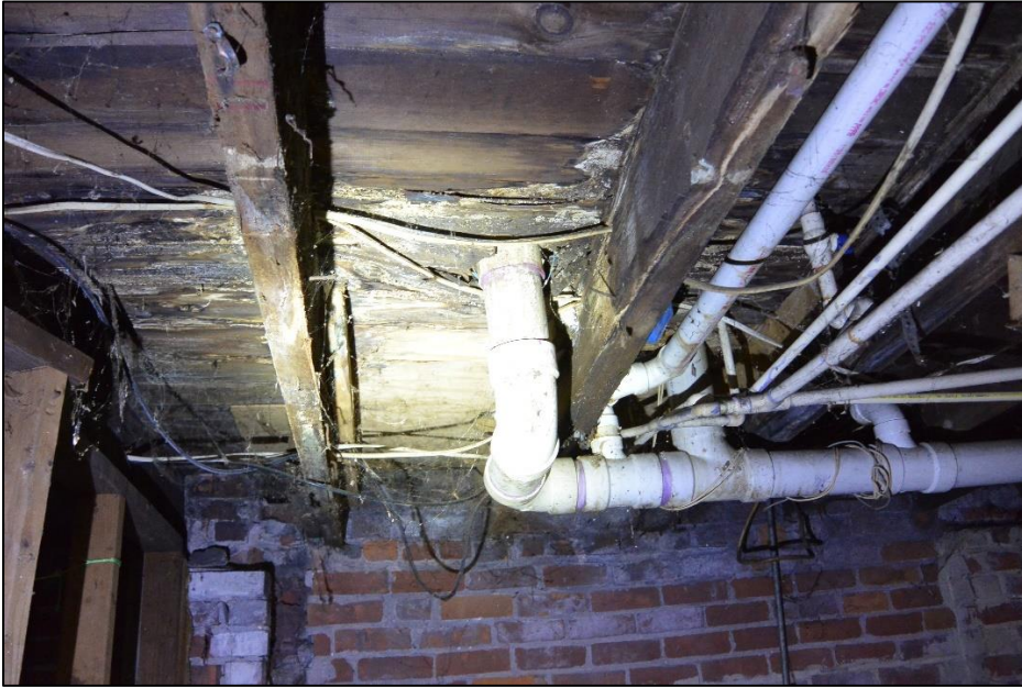
PHOTO NO. 3: Wood decay damage at plumbing penetrations.
