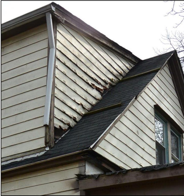
PHOTO NO. 5: Decayed wood siding, back-up framing, and poor flashing and drainage features.
