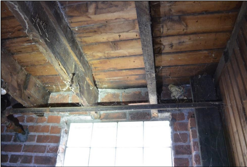
PHOTO NO. 4: Floor joists bearing on brick masonry resulting in structural concern due to likelihood for decay of wood encased in masonry exposed to the elements.
