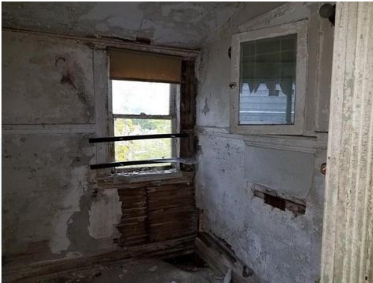
PHOTO NO. 10: Extensive deterioration and damage to interior finishes and signs of wood decay on some exposed interior lath and framing elements.
