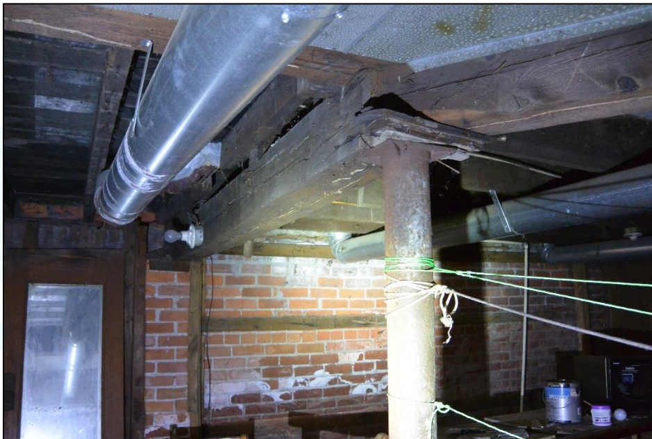
PHOTO NO. 2: Cracked wood girders supporting first floor faming with insufficient and nonconcentric bearing area with unorthodox shimming on steel post.
