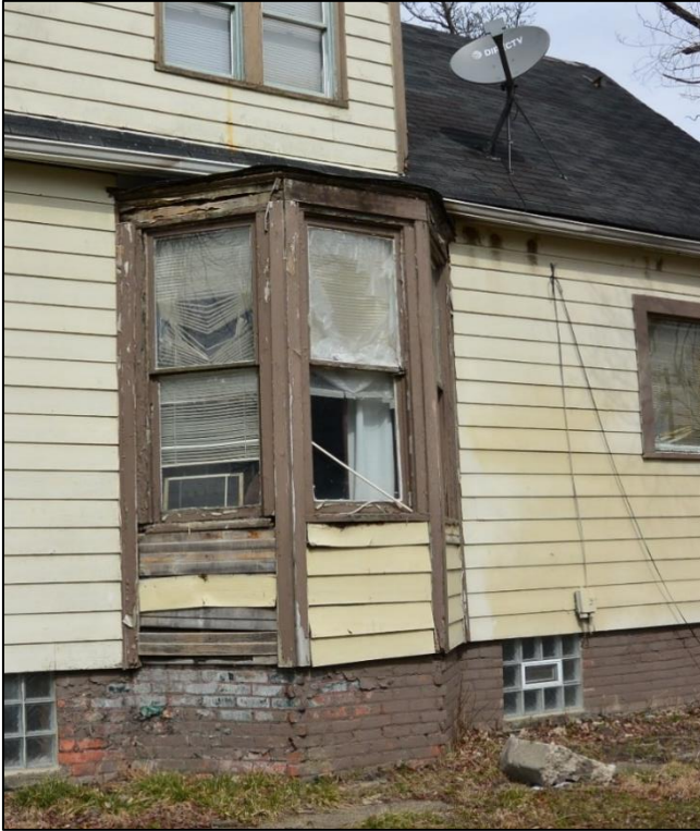
PHOTO NO. 7: Decay damaged wood at south elevation bay
