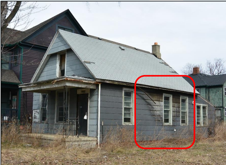
PHOTO NO. 8: Exterior fire damage to siding on exterior wall of south elevation (within red rectangle).
