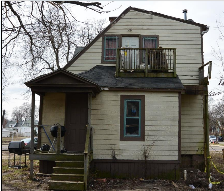
PHOTO NO. 6: Shed roof displacement beneath deck, may indicate over loaded shed roof joists.
