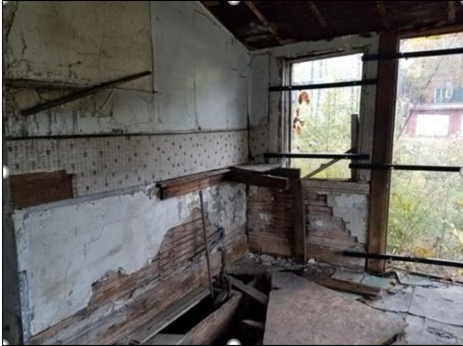
PHOTO NO. 11: Extensive deterioration and damage to interior finishes and signs of wood decay on some exposed interior lath and framing elements.
