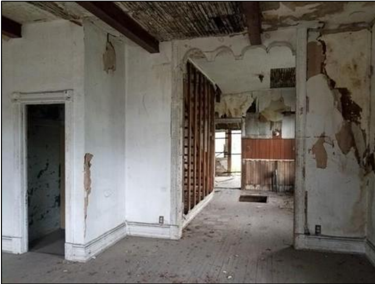
PHOTO NO. 9: Extensive deterioration and damage to interior finishes and signs of wood decay on some exposed interior lath and framing elements.
