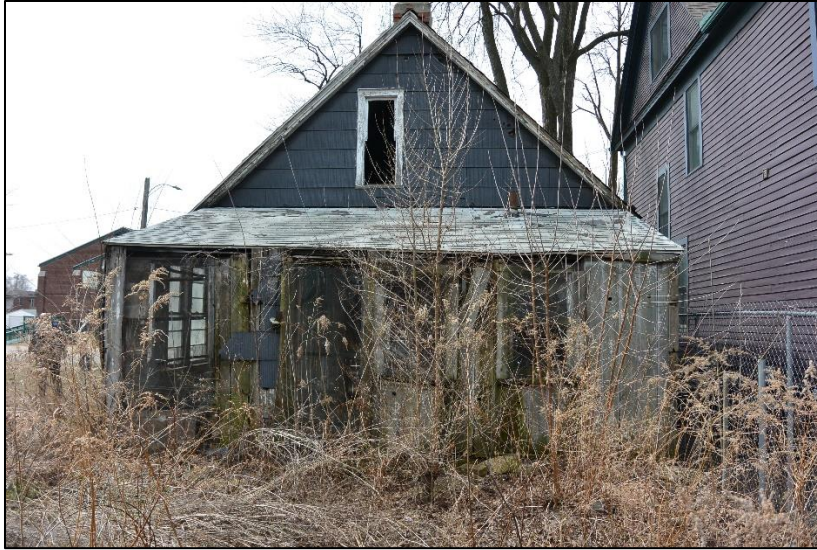
PHOTO NO. 13: Upper window were fully open to the elements on both north (shown) and south elevations.
