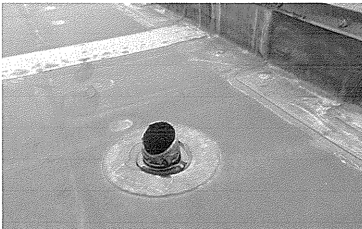
BROKEN PIPE NEEDS ATTENTION BY OTEHRS
