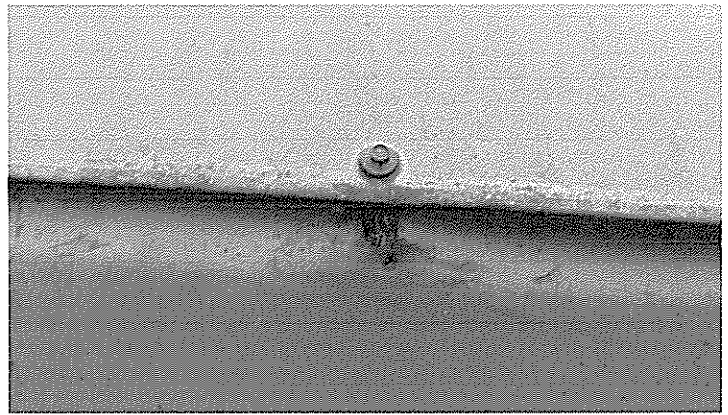
MEMBRANE STARTING TO PULL OUT FROM METAL
