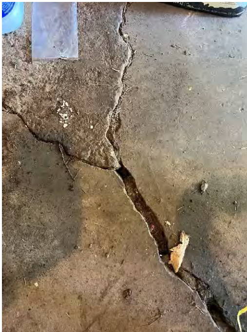
Deterioration of slab
