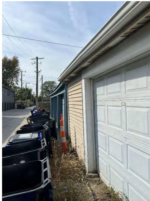
Exterior wall out of plumb
