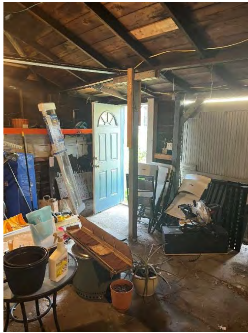
Excessive deflection in supporting member
