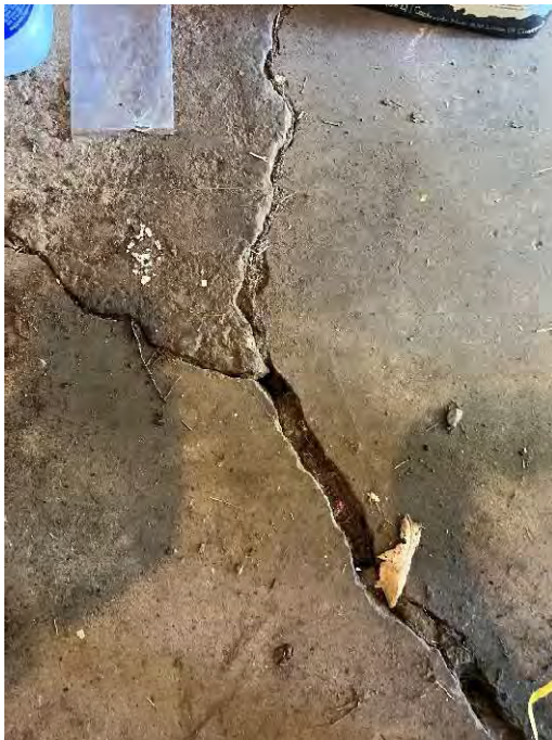
Deterioration of slab
