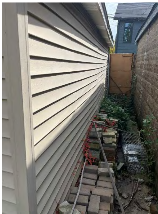
Buckling evident in exterior wall – west side
