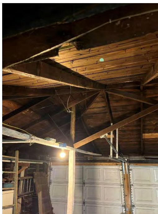
Example of framing member deflection
