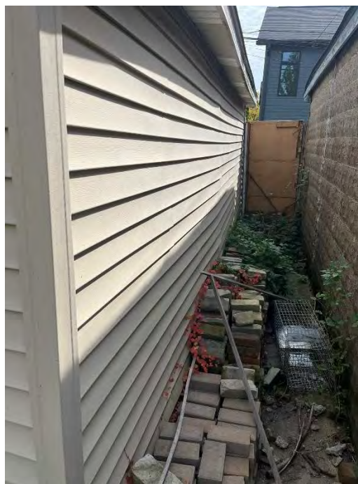
Buckling evident in exterior wall – west side
