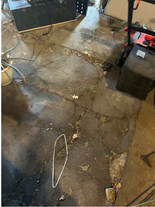
Interior concrete slab deterioration
