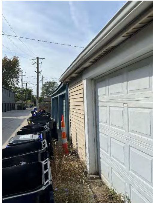
Exterior wall out of plumb
