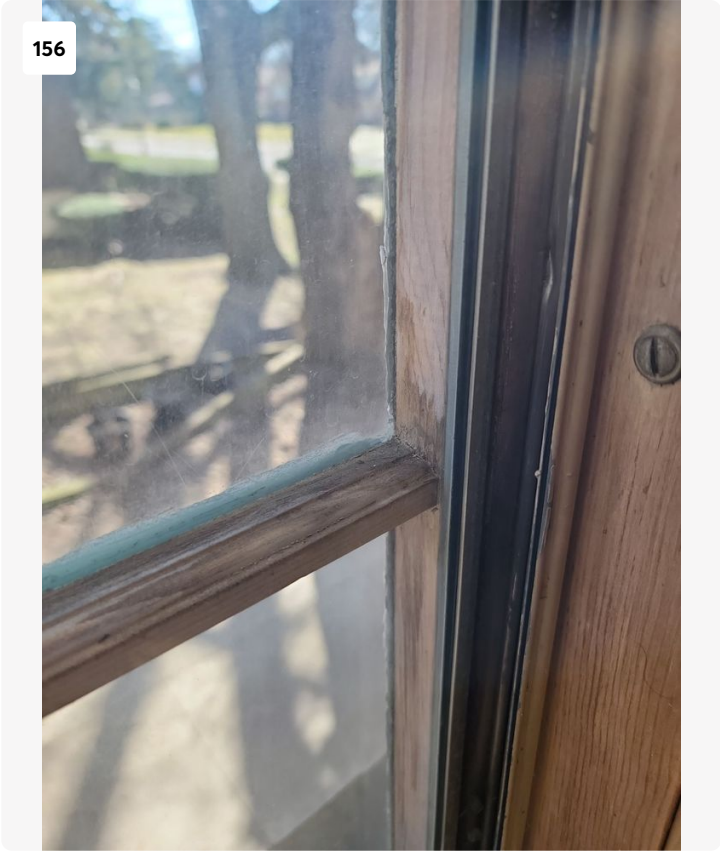
1600- water damage, mold, broken seals, hardware is non functioning, window does not open, condensation between glass, decayed wood between glass
