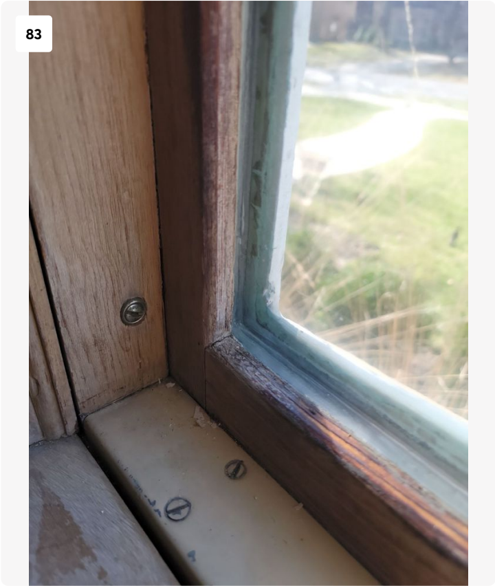
700-Mold, water damage, broken seals, decayed wood inside of glass, condensation inside of glass
