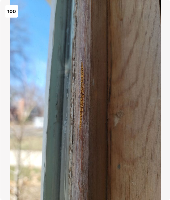
600-Mold, water damage, broken seals, decayed wood inside of glass, condensation inside of glass
