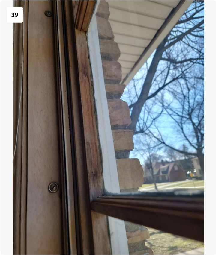
1000-Mold, water damage, broken seals, hardware in non-functional, window does not open
