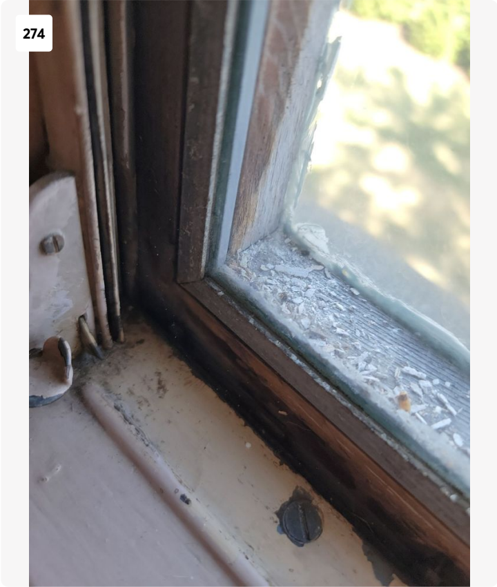
2200- water damage, mold, broken seals, hardware is non functioning, window does not open, condensation between glass, decayed wood between glass, bugs between glass
