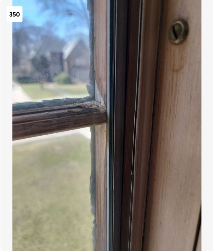
3000- water damage, mold, broken seals, hardware is non functioning, window does not open, condensation between glass, decayed wood between glass
