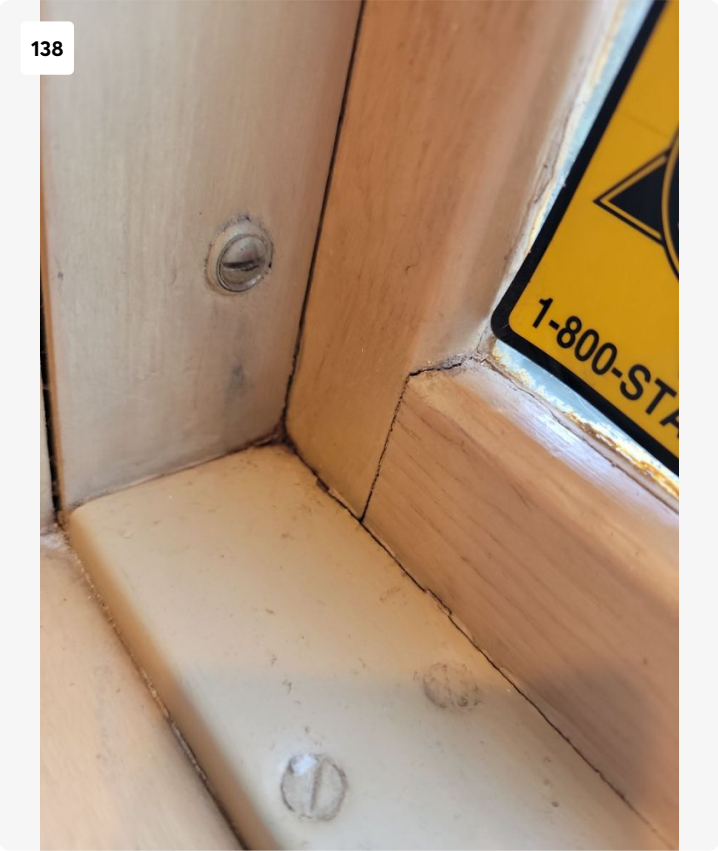
200- Broken frame, cracked seals, water damage, mold, decayed wood inside of glass, condensation in between glass
