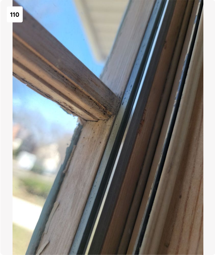
500-Mold, water damage, broken seals, decayed wood inside of glass, non functioning hardware, window does not open, condensation inside of glass
