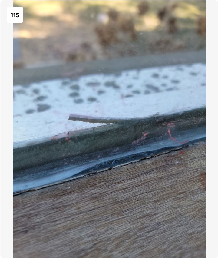
400-Mold, water damage, broken seals, decayed wood inside of glass, condensation inside of glass
