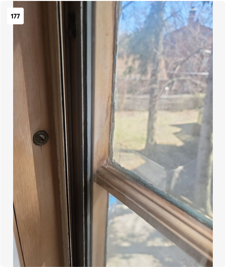
1700- water damage, mold, broken seals, hardware is non functioning, window does not open, condensation between glass, decayed wood between glass
