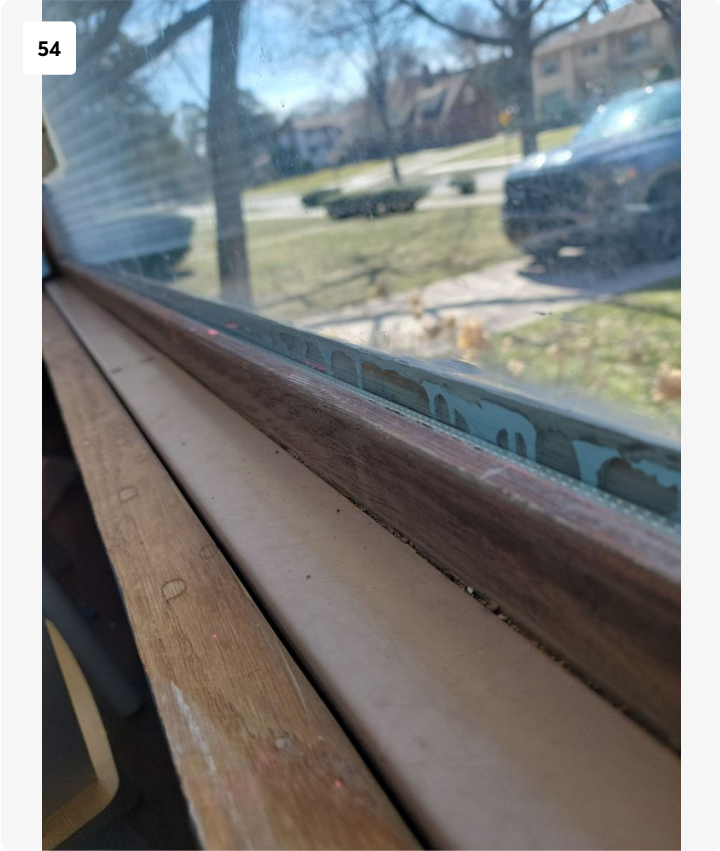
1100-Mold, water damage, broken seals, condensation inside of glass
