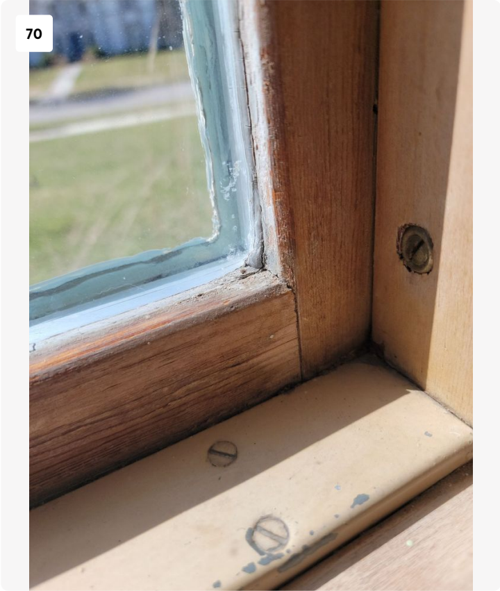
800-Mold, water damage, broken seals, decayed wood inside of glass, condensation inside of glass
