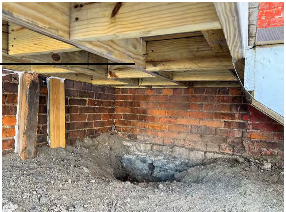
The porch structure is modern, exterior grade 2x members. No joist hangers were used as required. It is unclear how the "rim board" is attached to the brick masonry.
