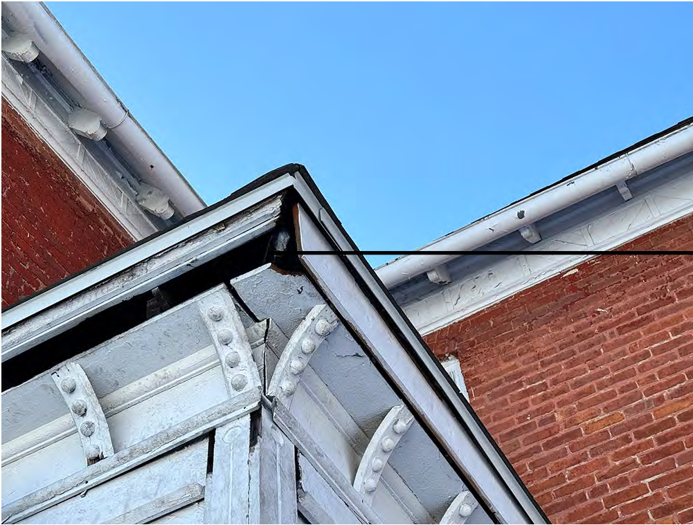
Separation and deterioration of the fascia boards remaining, some parts of the fascia are missing. Improper drip edge for the roof causing moisture to destroy the fascia board
