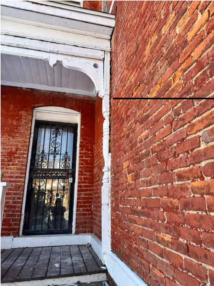
The pilaster is separating from the wall and is not attached properly to support the roof above
