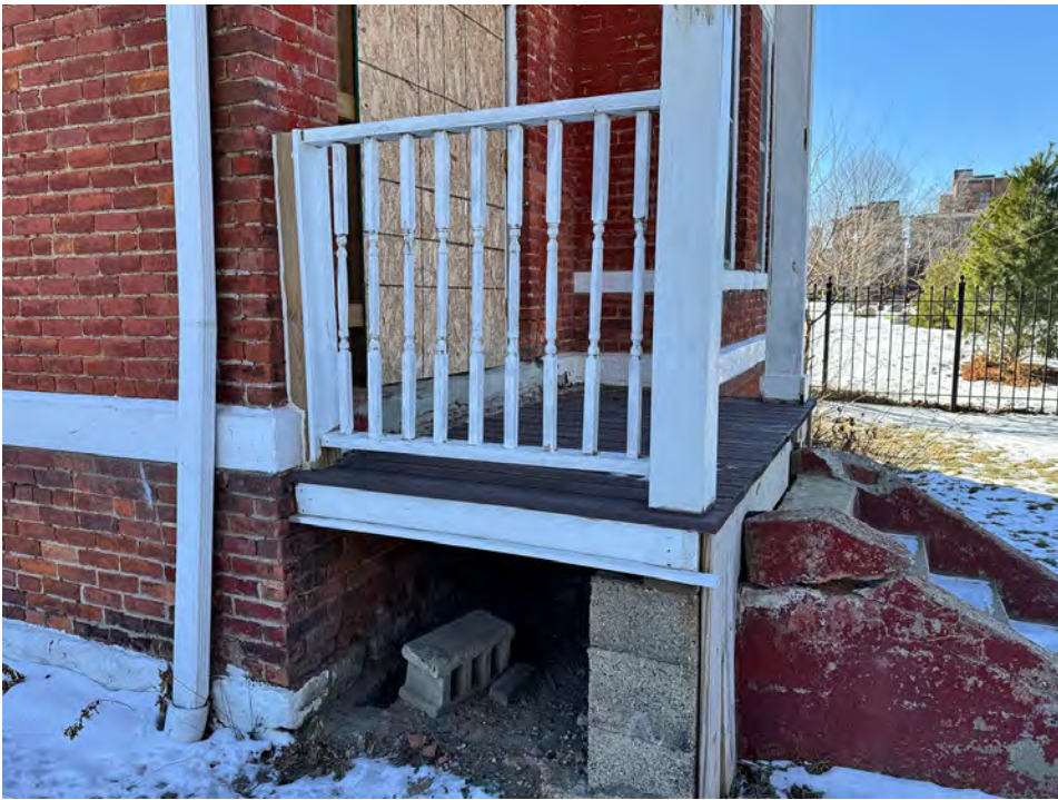
This is the front porch for reference, showing the same techniques used on the rebuilt side porch which is now in place, 2x structural members, 5/4 deck boards, 2x top cap rail
