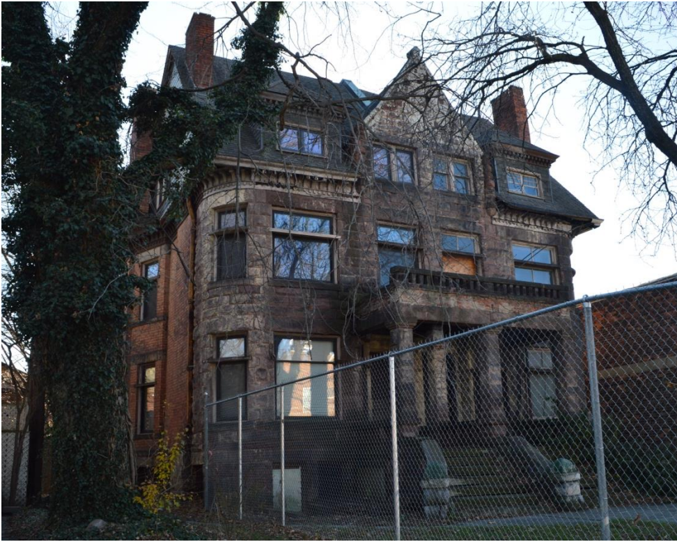
701 W. Canfield – Before (2017) and Current (work still in progress) photo of front elevation
