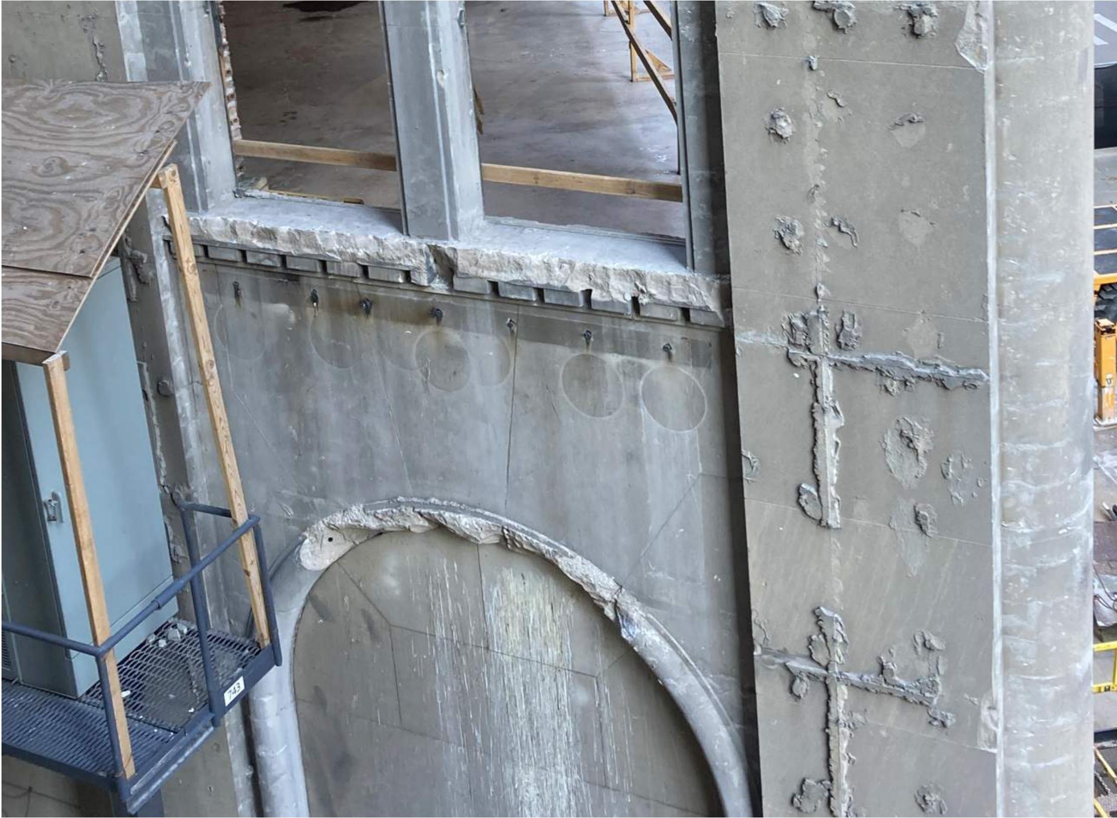
Alley facade at 3rd floor sill and dentils and 2nd floor arch
