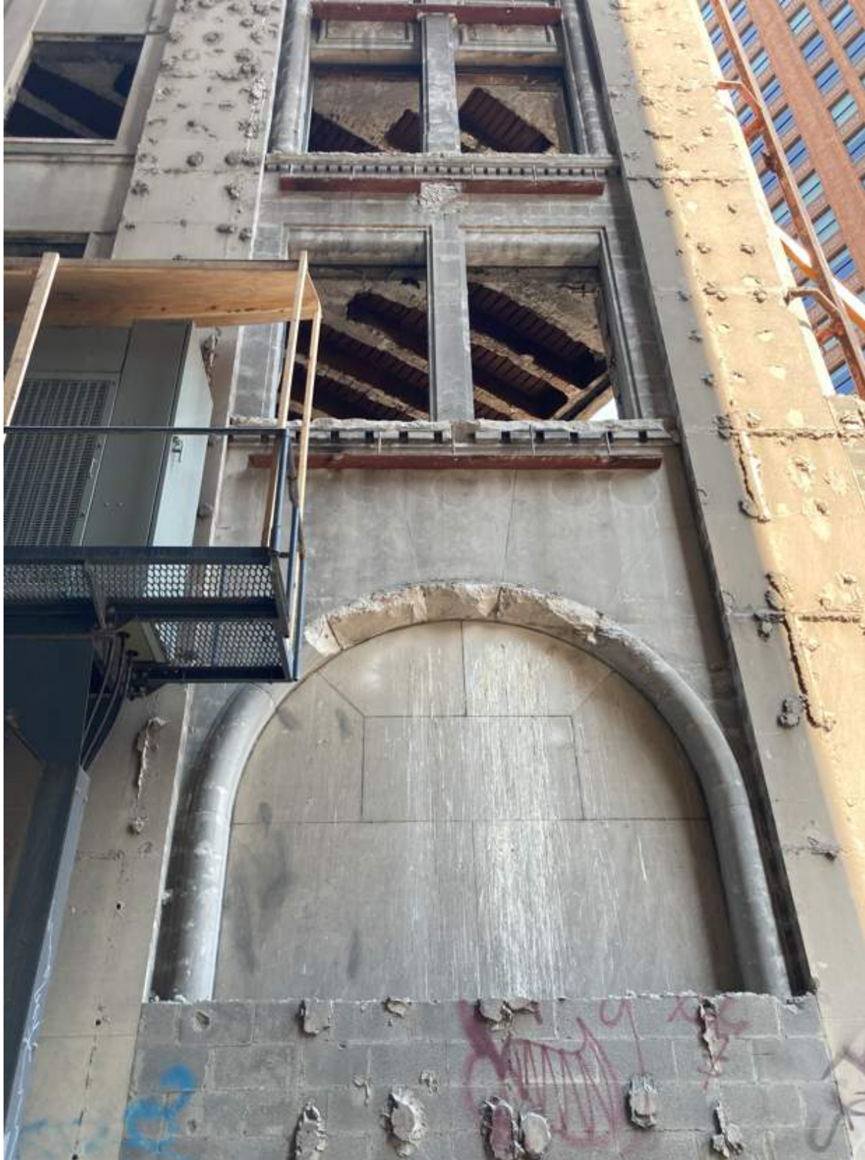
Alley facade after removal of CMU block, before removal of steel angles
