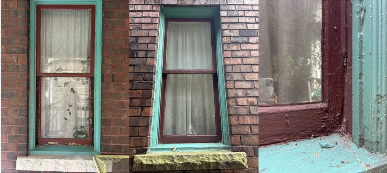
Window detail. First floor living room south (left); dining room left (center), dining room center (right); substantially damaged and inoperable
