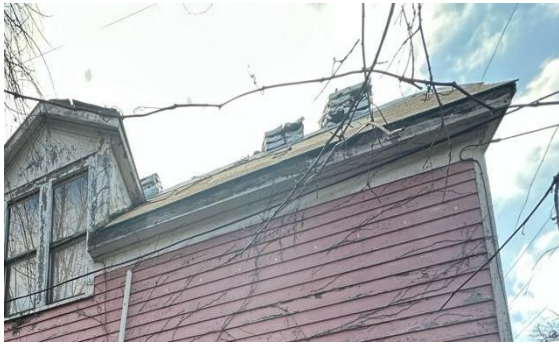
Old deteriorated and cracked former roof
