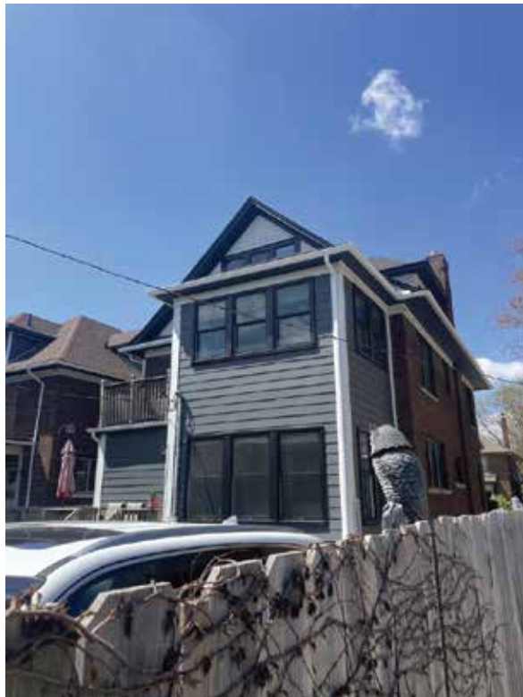
Finished Example of proposal repairs This photo was taken of the house next door 1659 Edison St
