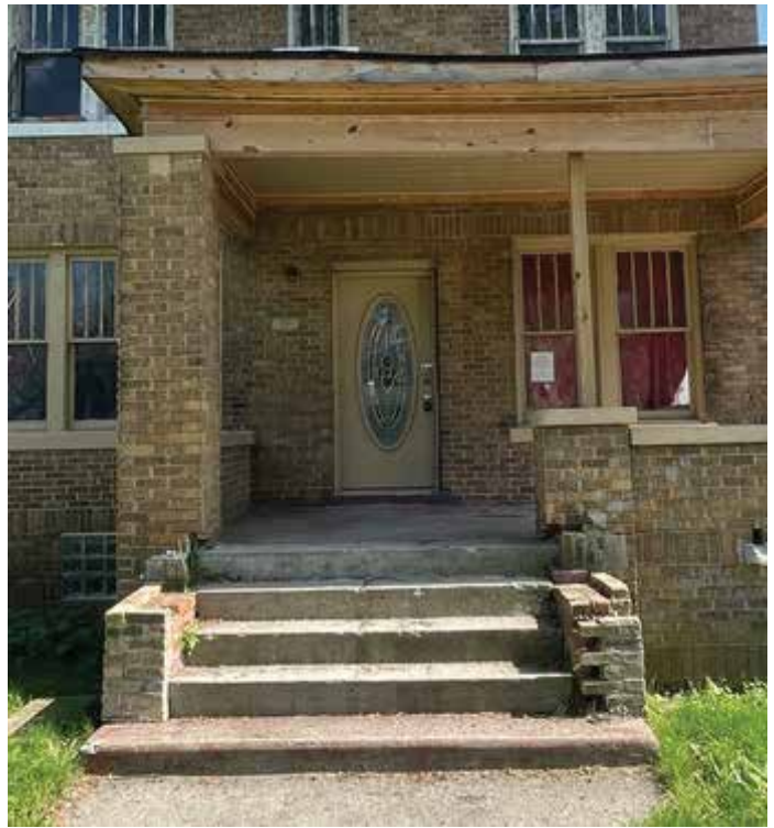
Replace missing bricks from front steps additional install missing caps on top of the bricks.
