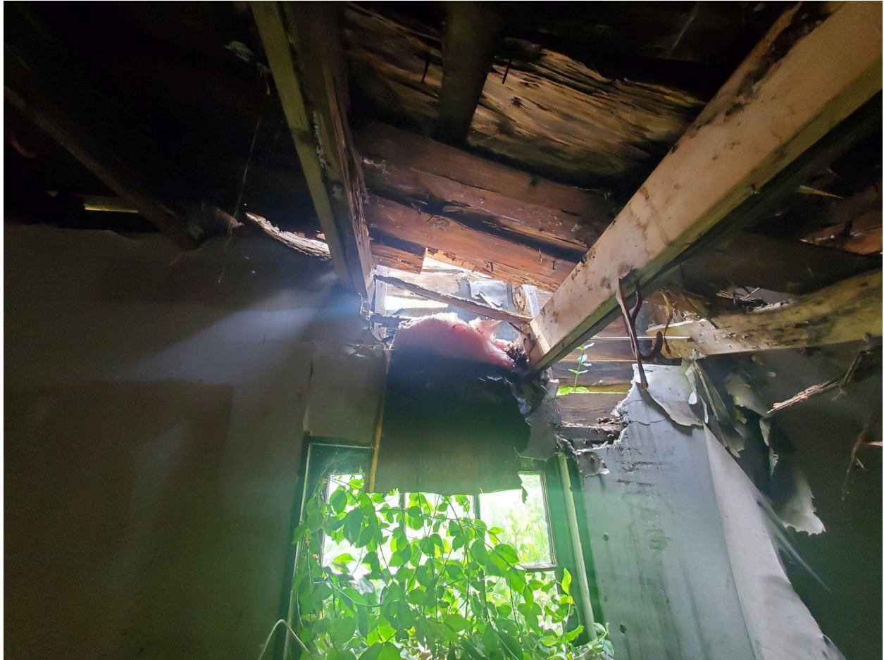
Typical Damage to Garage
