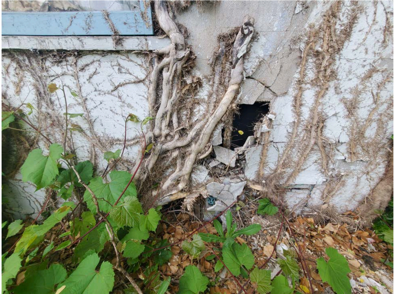
Typical Stucco Damage
