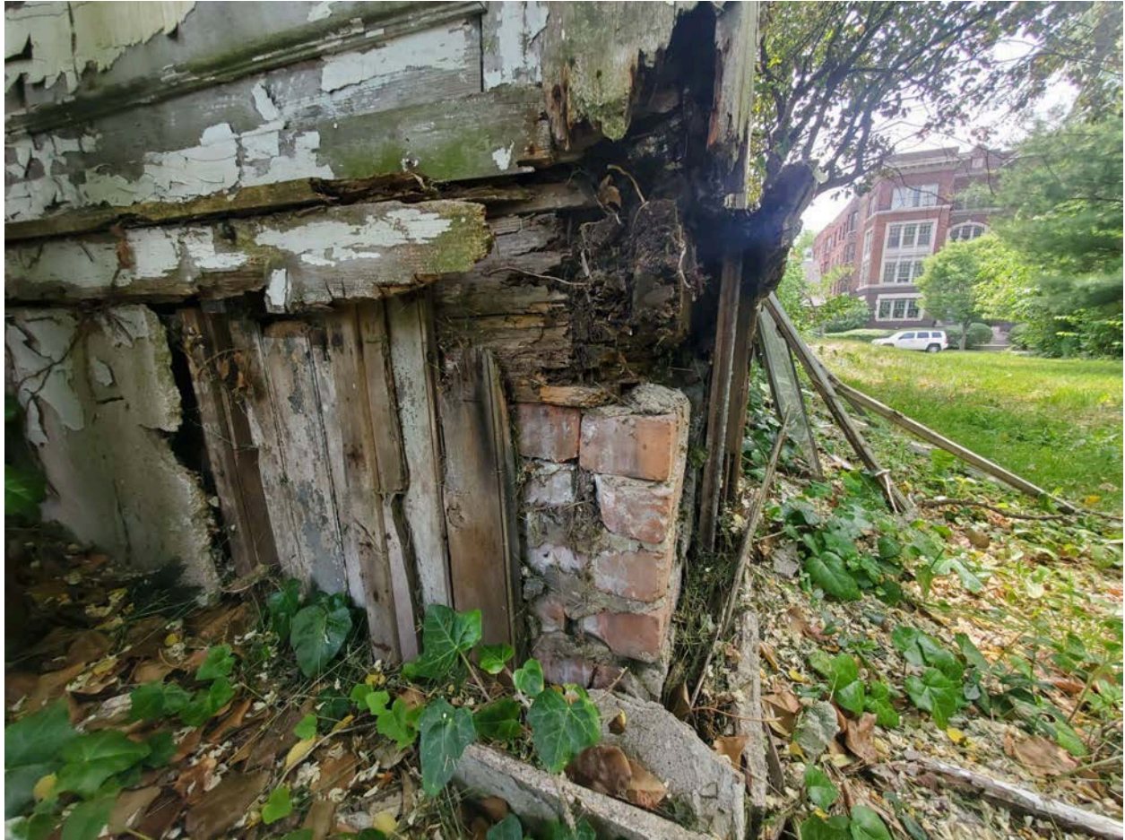
Typical Damage to Bay Window Footing
