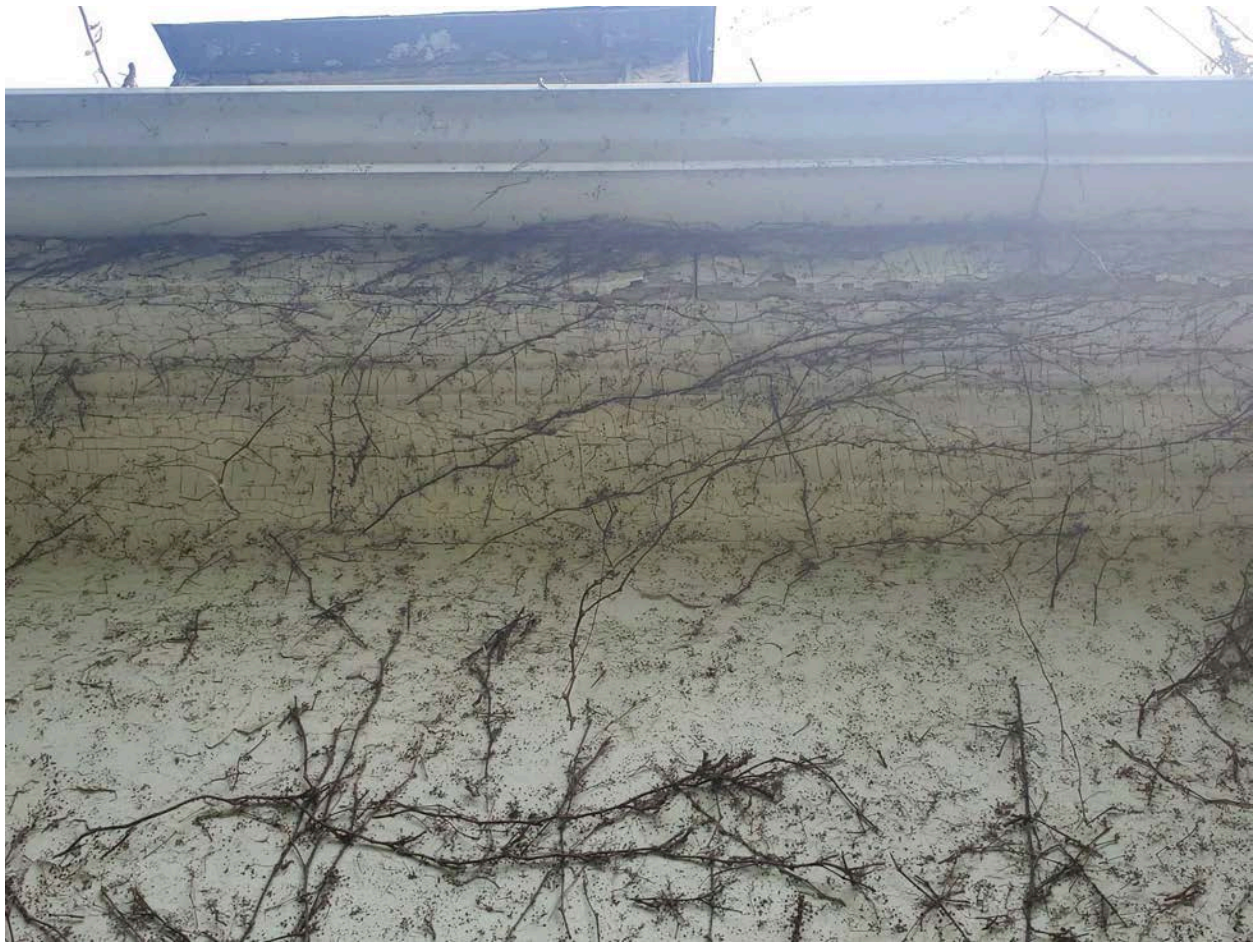
Typical Damage to Wood Detailing
