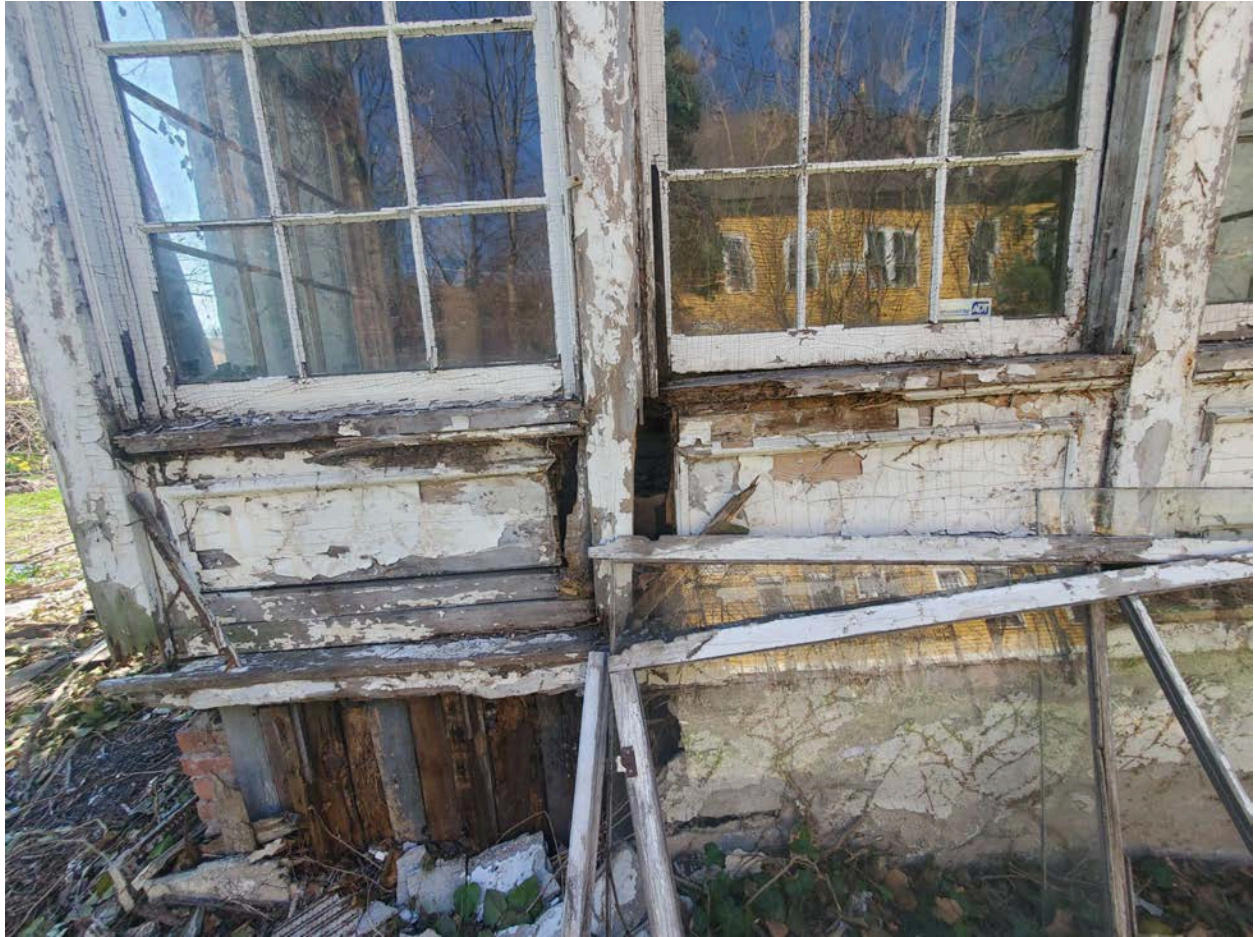
Typical Damage to Bay Window
