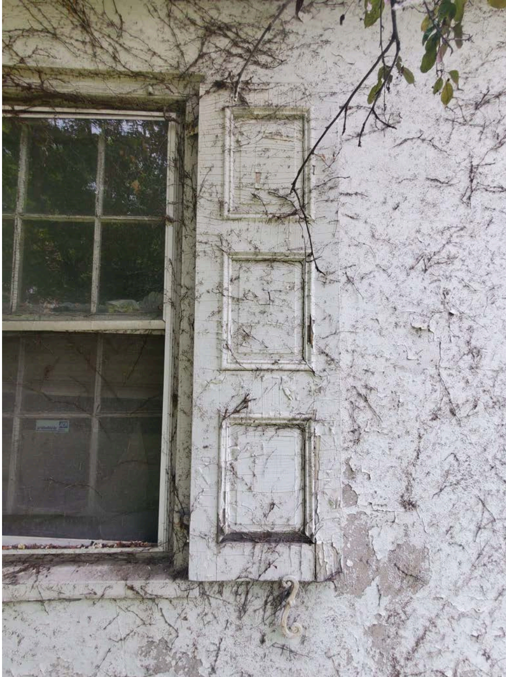
Typical Damage to Wood Shutter
