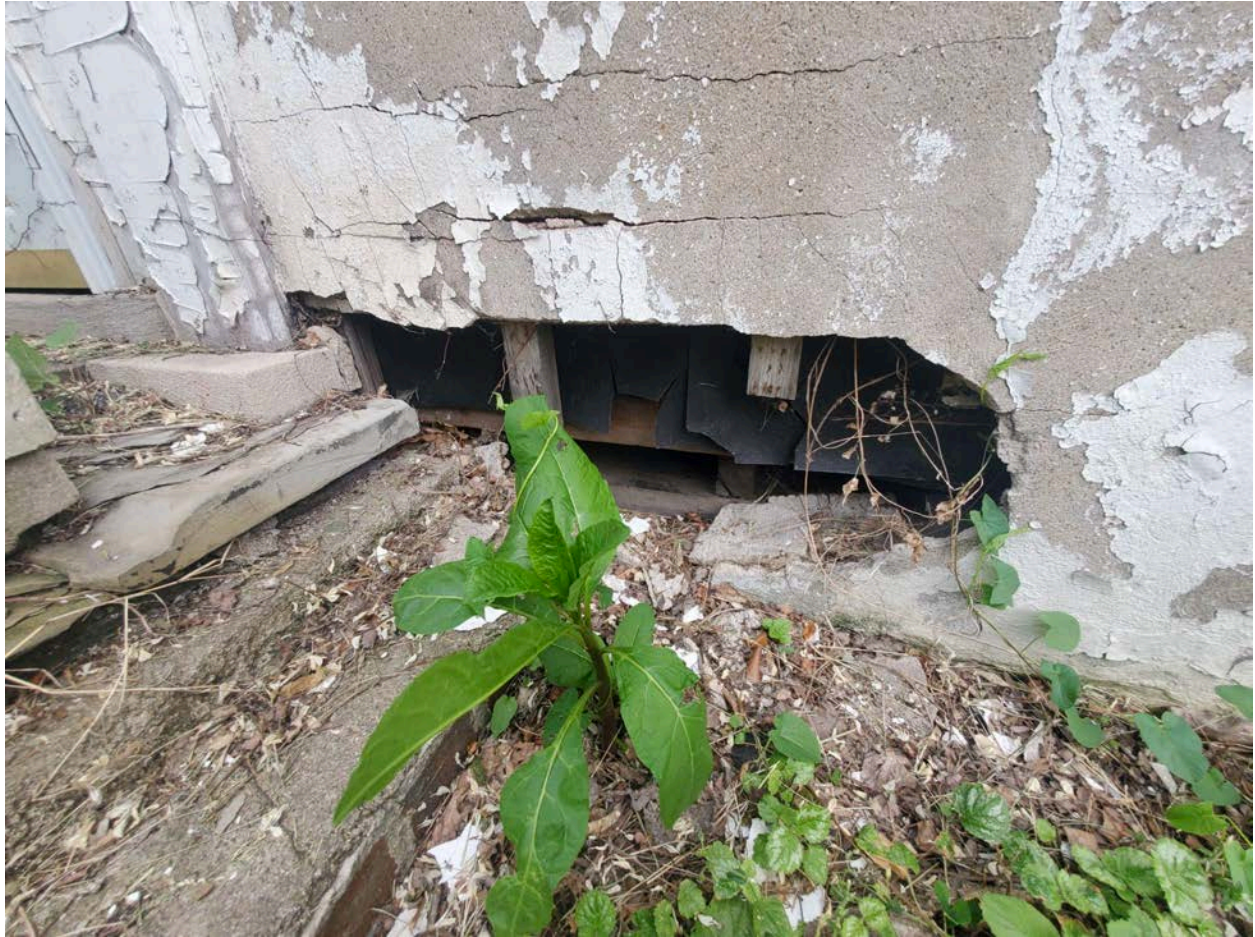
Typical Stucco Damage
