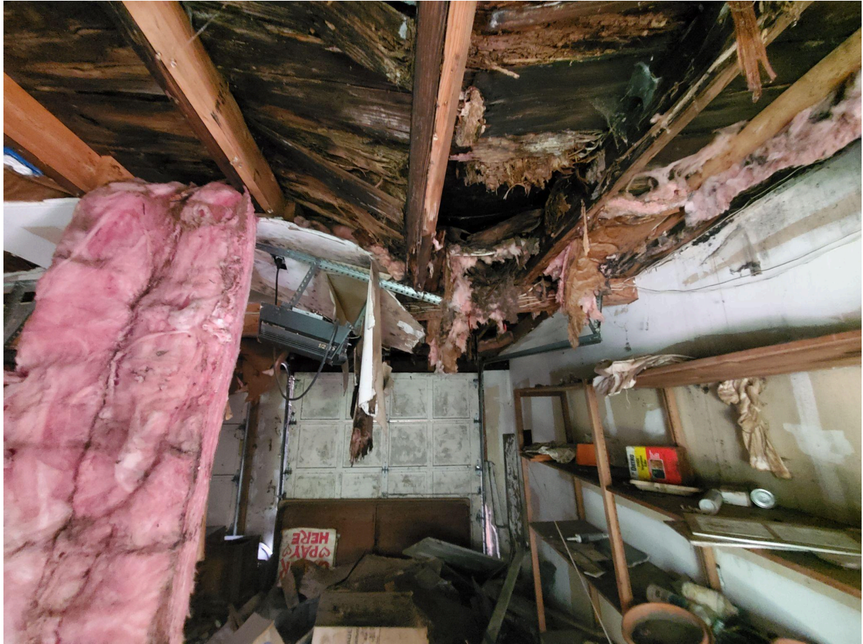
Typical Damage to Garage
