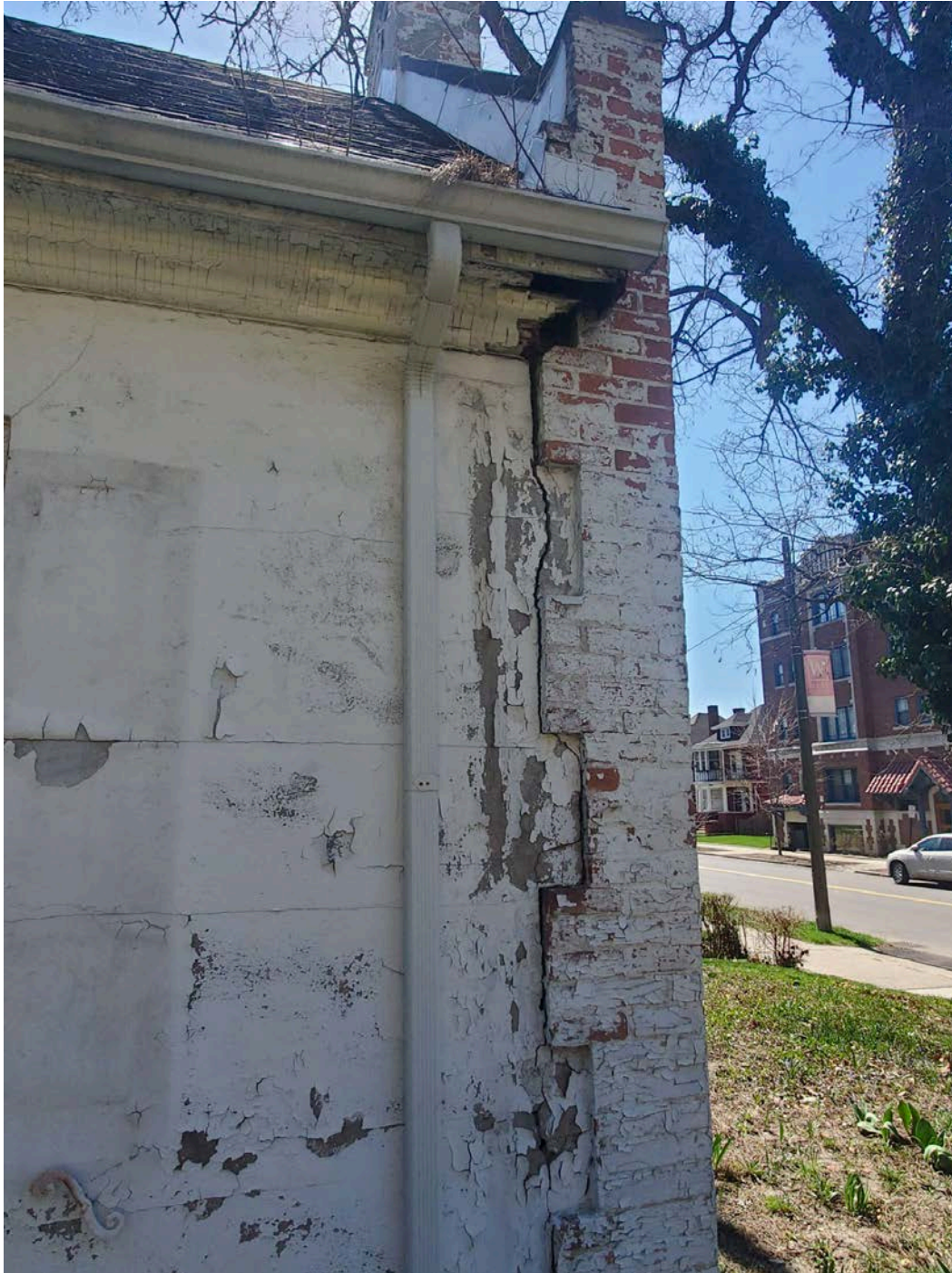
Typical Damage to Facade Detail
