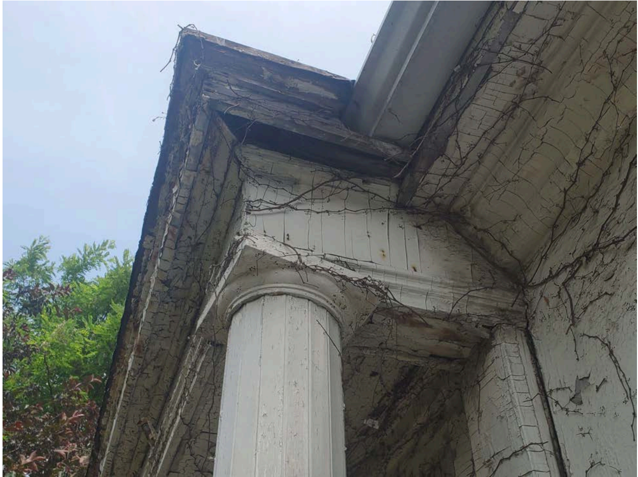
Existing Porch Canopy Typical Damage
