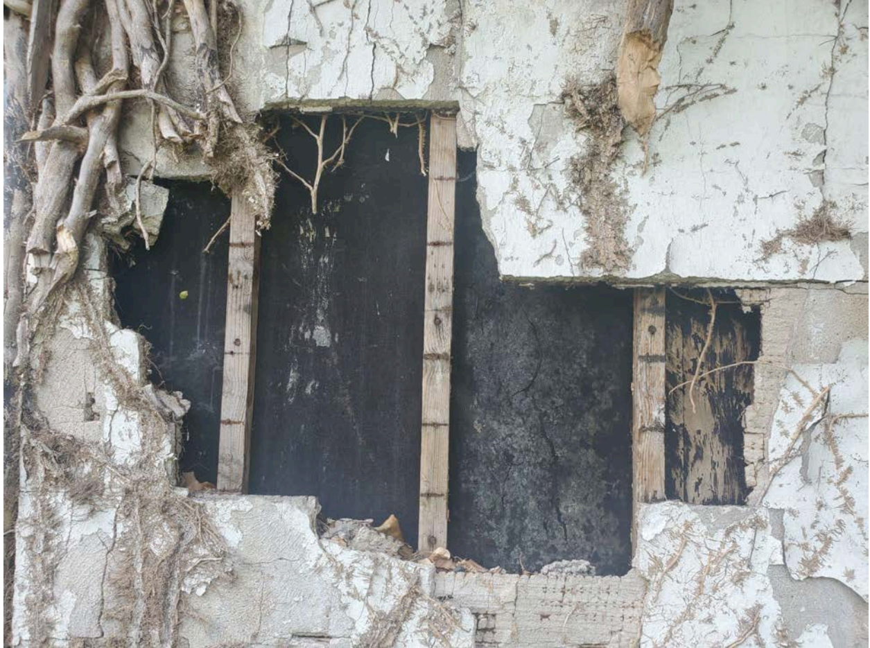
Typical Stucco Damage
