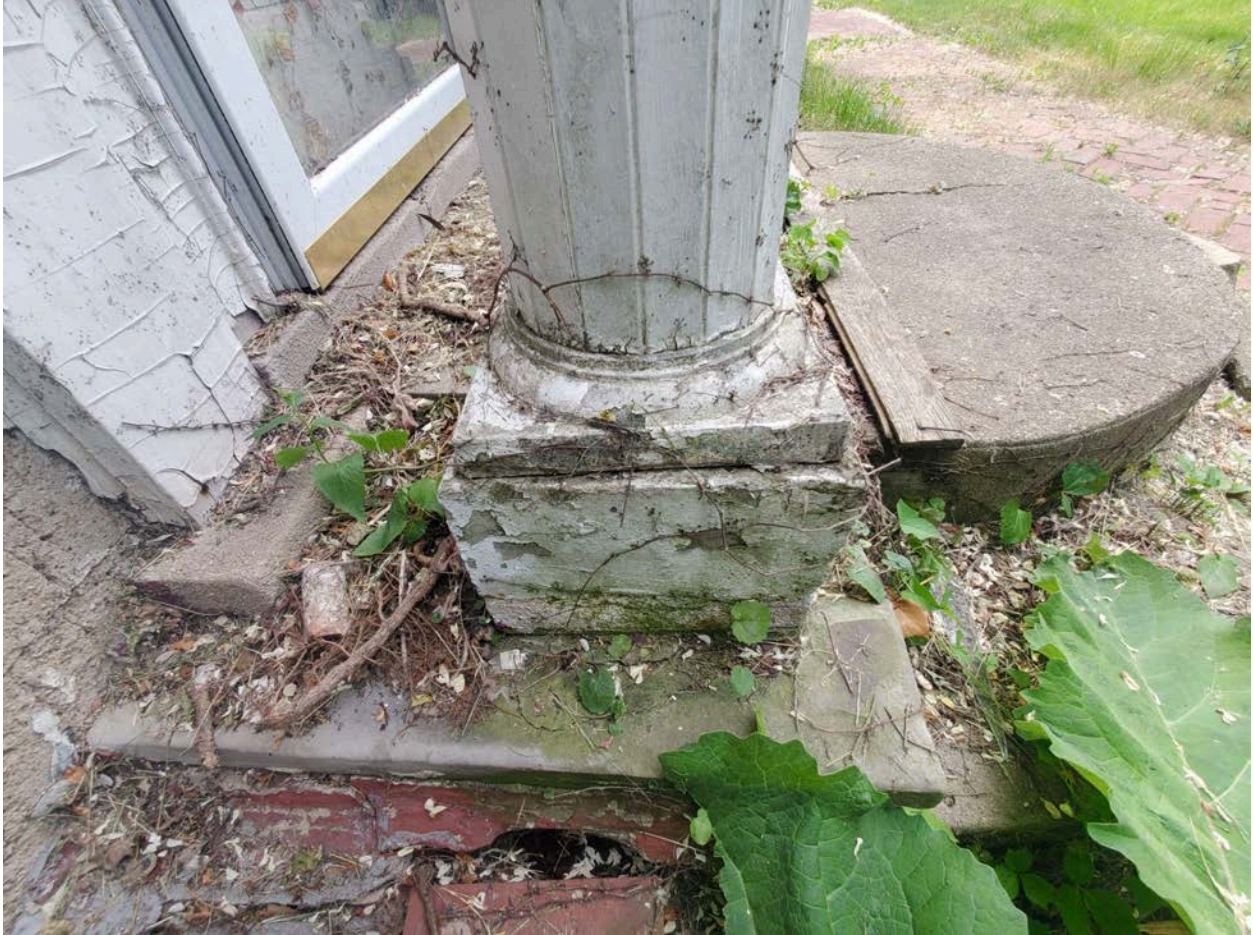
Existing Porch Loose Column Base
