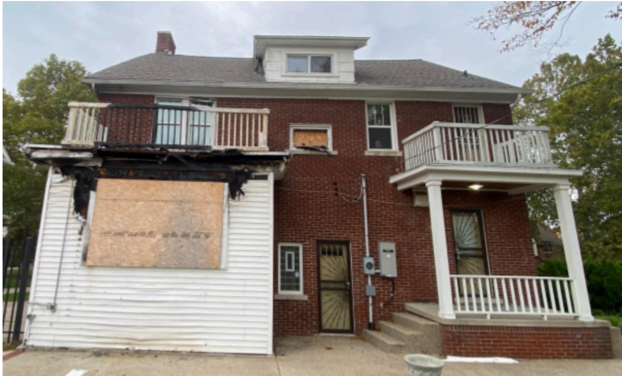
Fig. 13.0 - Rear of 570 Lodge. The rear “office” was severely damaged in a fire. Exterior vinyl siding was damaged, as well as windows and soffit assembly.
