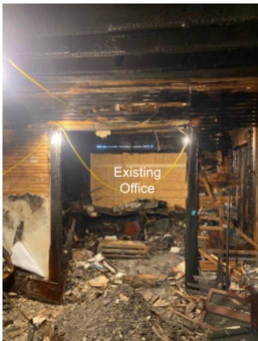
Fig. 14.0 - Fire severely damaged interior of “office”
