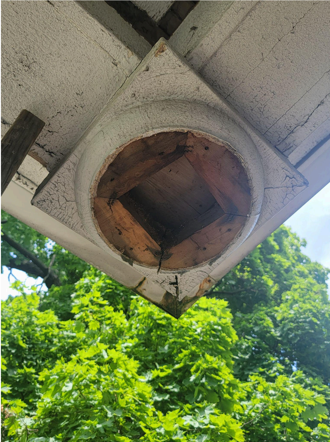
Missing Column Placement
