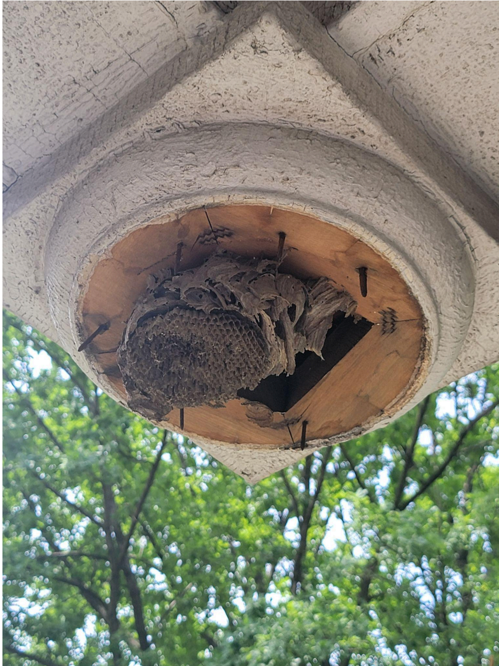
Missing Column Placement showing insect damage
