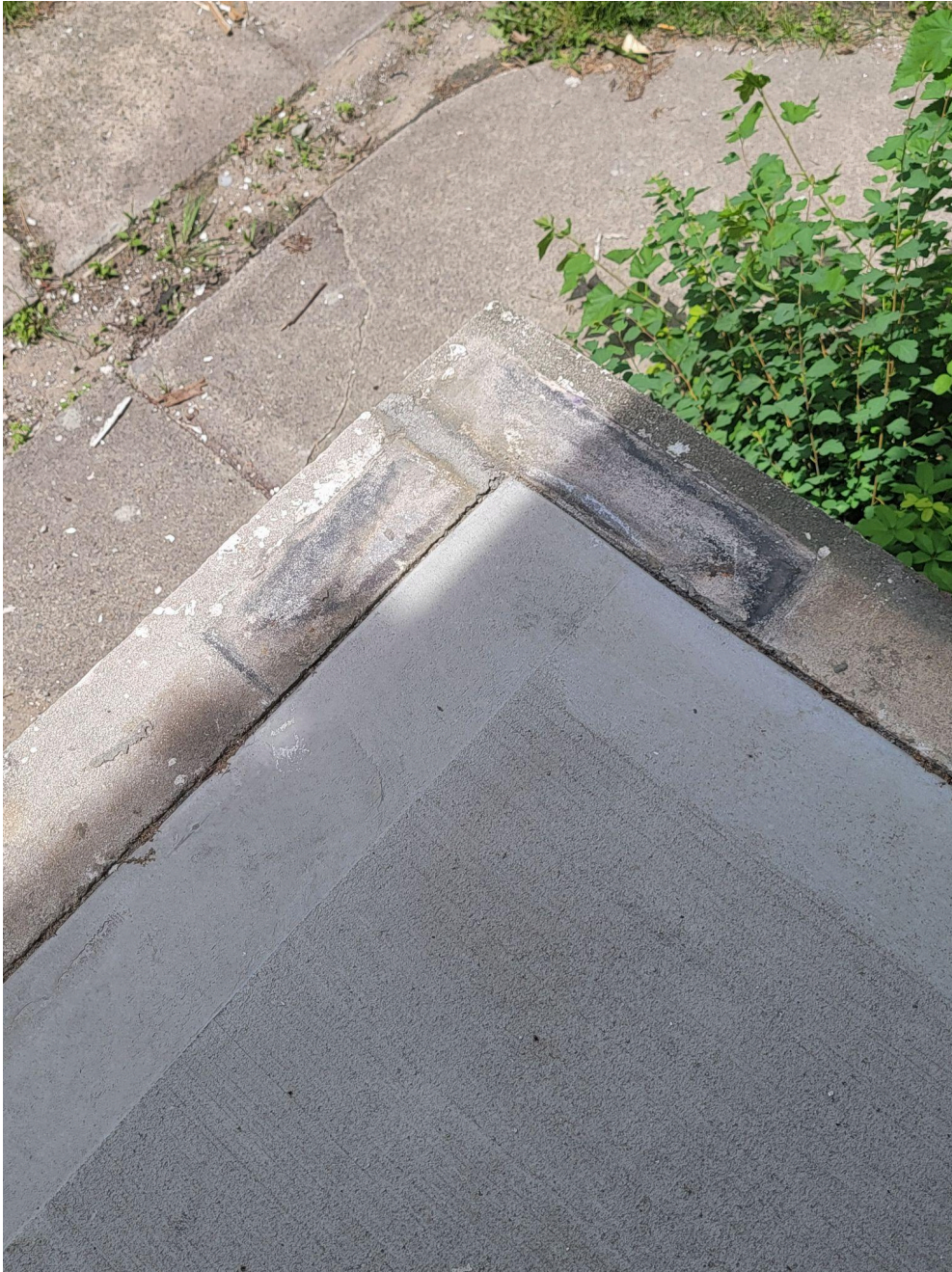
Missing Column Base at Porch (typical)
