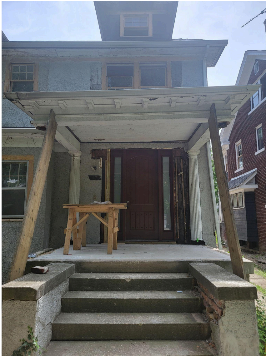
Front Porch Elevation
