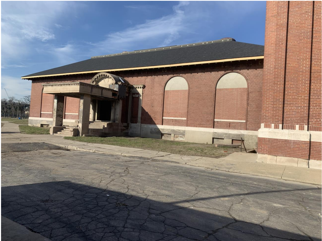
Existing Condition Photo 6: The canopy was added & decreased the height of the original entry. When the canopy was added, this metal flashing was also added. CDS proposes the added canopy, added door and added metal flashing be removed.
