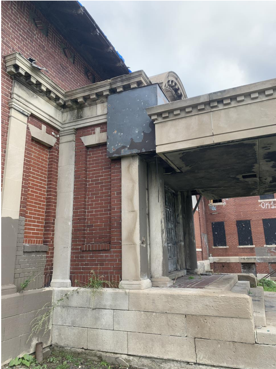
Existing Condition Photo 5: The canopy was added & decreased the height of the original entry. When the canopy was added, this metal flashing was also added. CDS proposes the added canopy, added door and added metal flashing be removed.
