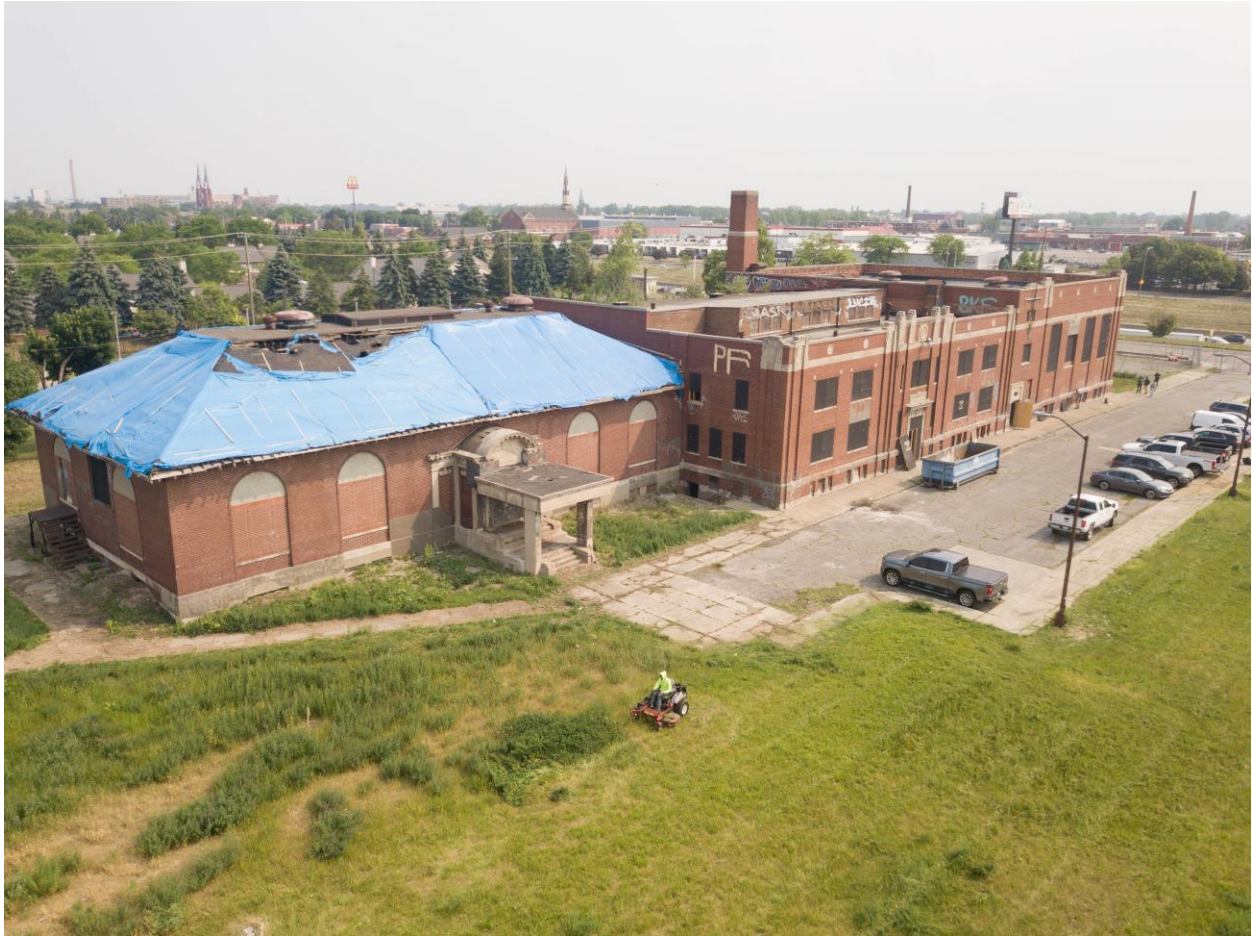
Existing Condition Photo 4: The canopy was added & decreased the height of the original entry.
