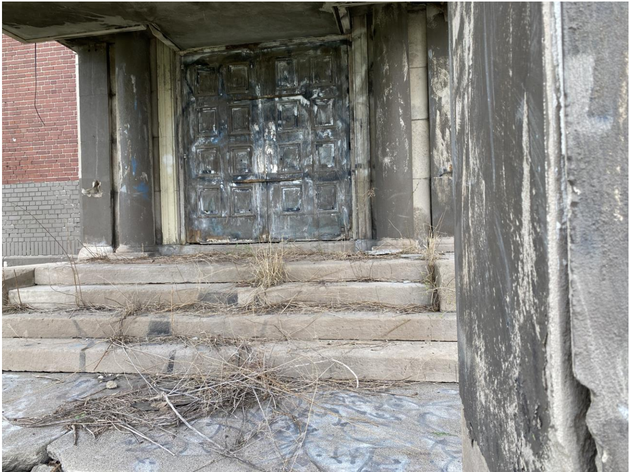
Existing Condition Photo 2: The existing door & frame were infilled in the original frame. The existing door has significant material loss through aging & weathering. With the removal of the canopy, the existing door in this photo (or a replica of this door) will not achieve a historically accurate façade.
