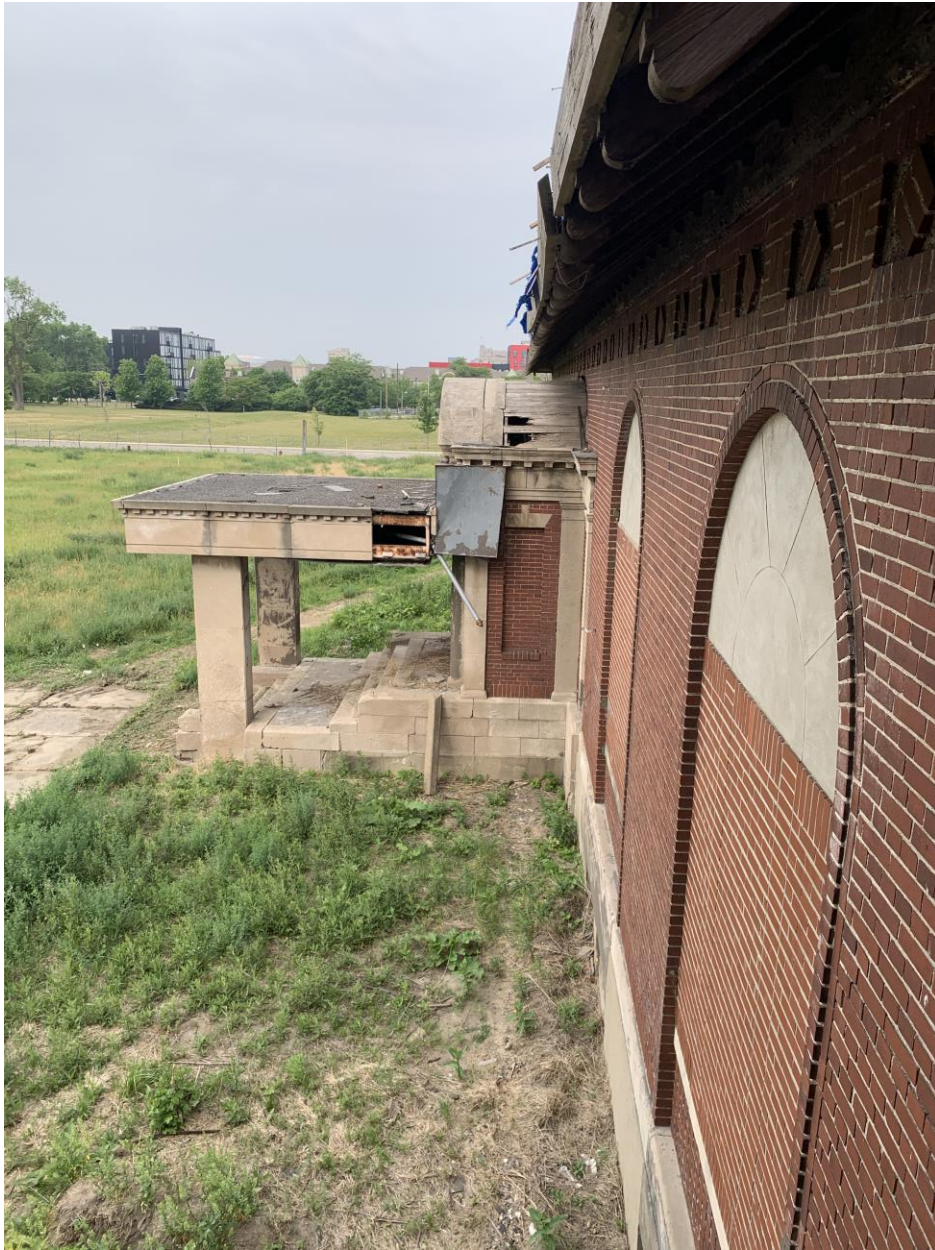
Existing Condition Photo 7: The canopy was added & decreased the height of the original entry. When the canopy was added, this metal flashing was also added. CDS proposes the added canopy, added door and added metal flashing be removed.
