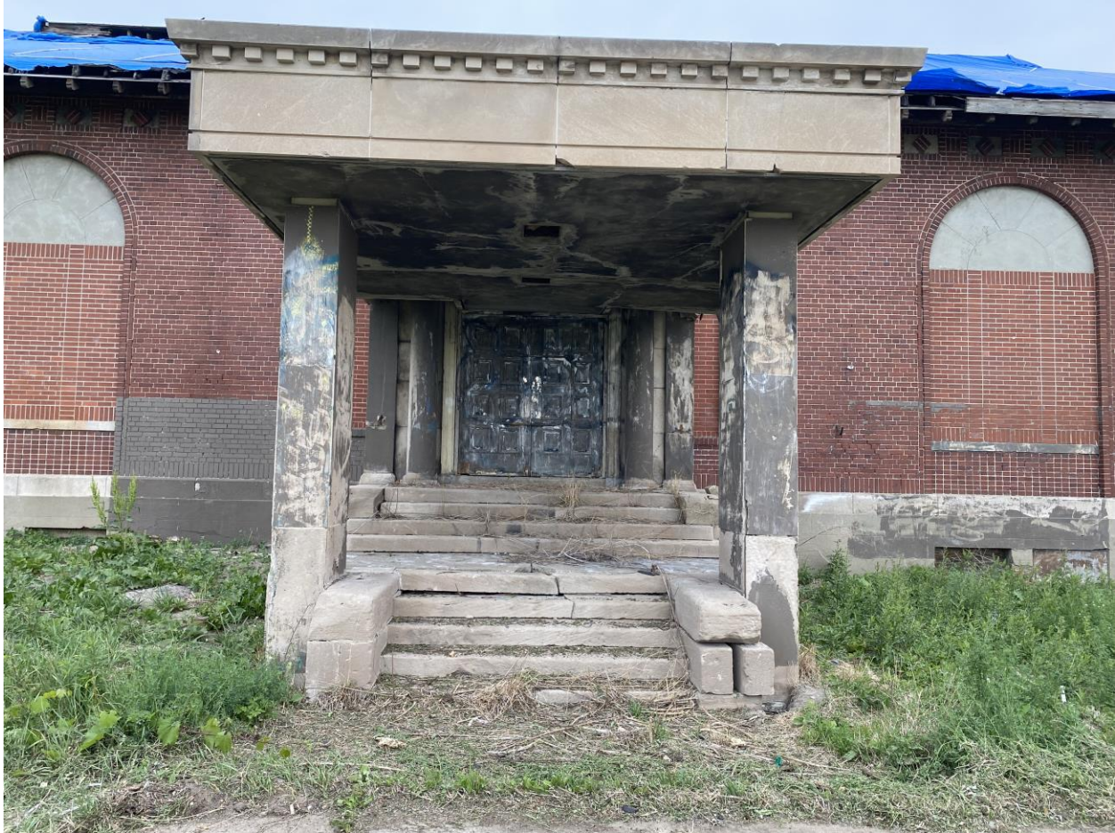
Existing Condition Photo 1: Original height of door & frame were lowered as a result of the existing canopy. A new door was also added in the existing frame to fit this reduced height.
