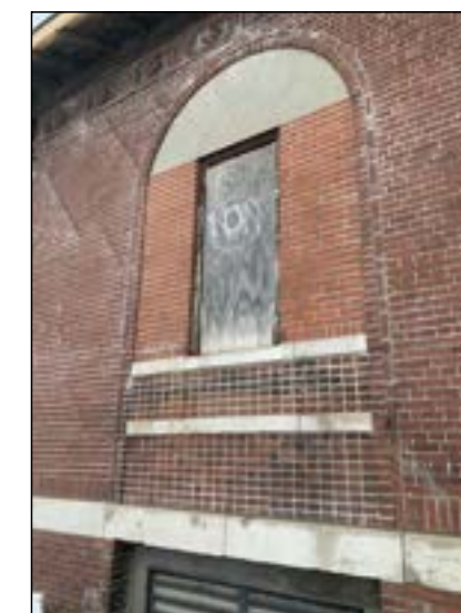
EXISTING H.M. DOOR FRAME W/ FLYWOOD INFILL
