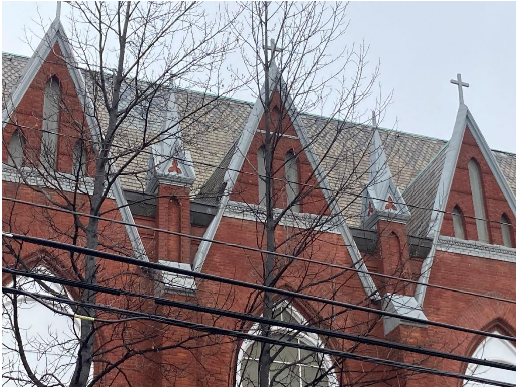
Current conditions, facing northeast, detail showing metal fascia with cross-shaped finials, metal spires with trefoil detailing, and copper gutters typical at roof. These elements will be removed in whole/throughout and will be replaced with new copper elements to match the existing. Staff photo taken 1/25/2024
