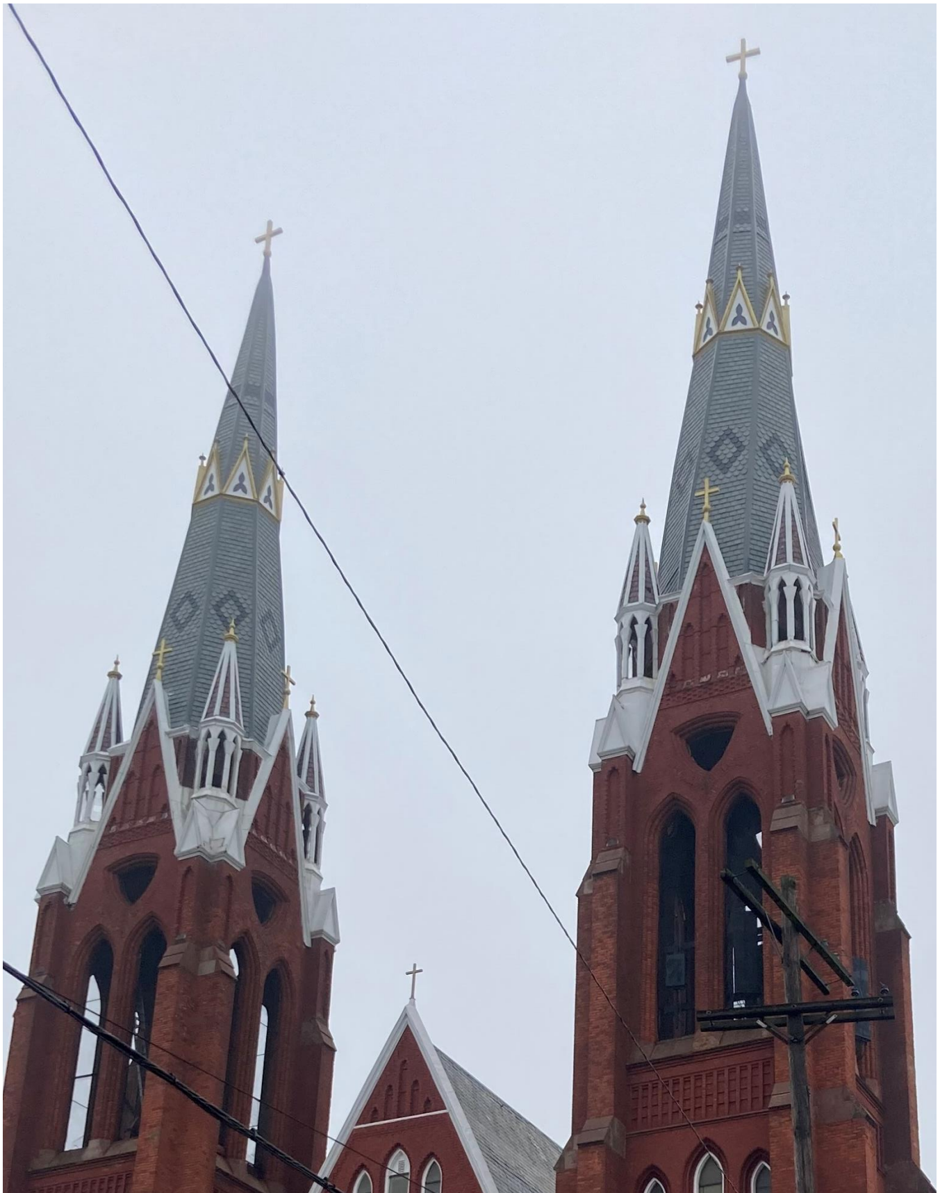
Detail of spires with recently installed Davinci synthetic slate roofing, current conditions, photo taken on 1/25/2024 by staff.
