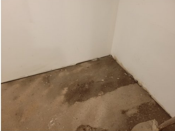
Photo 7 Moisture in basement
