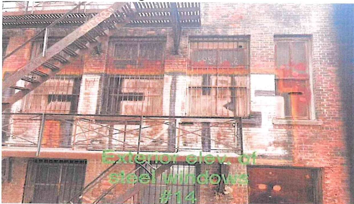
Exterior of typical steel windows exposed to elements and vandalism
