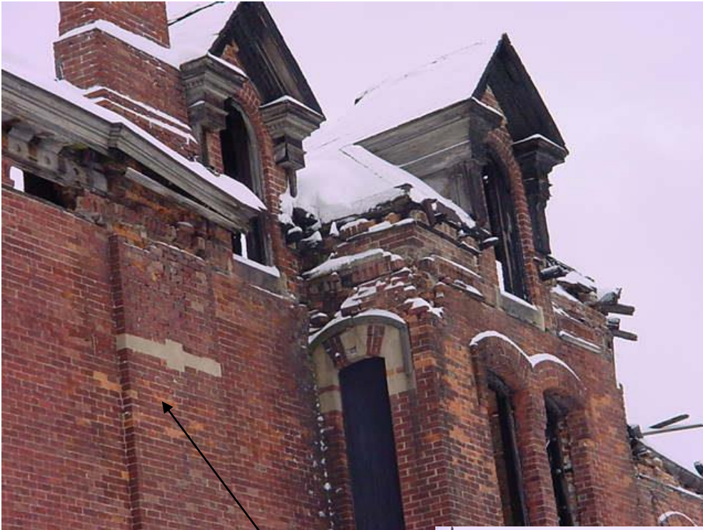
96-104 Edmund Place, second and third story detail of west elevation. Chimney (arrow) is proposed to be rebuilt.
