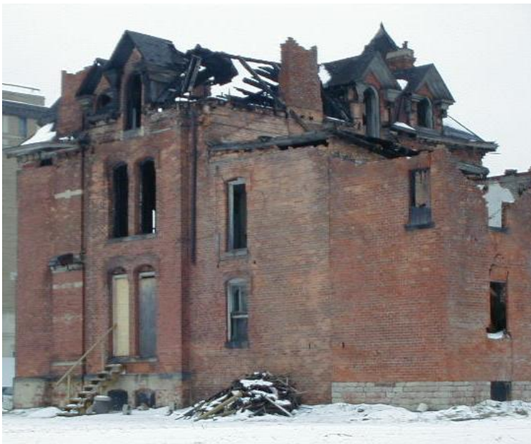
96-104 Edmund Place, side view of addition proposed to be rebuilt. Notice the brick line, the foundation change and lower eave line.
