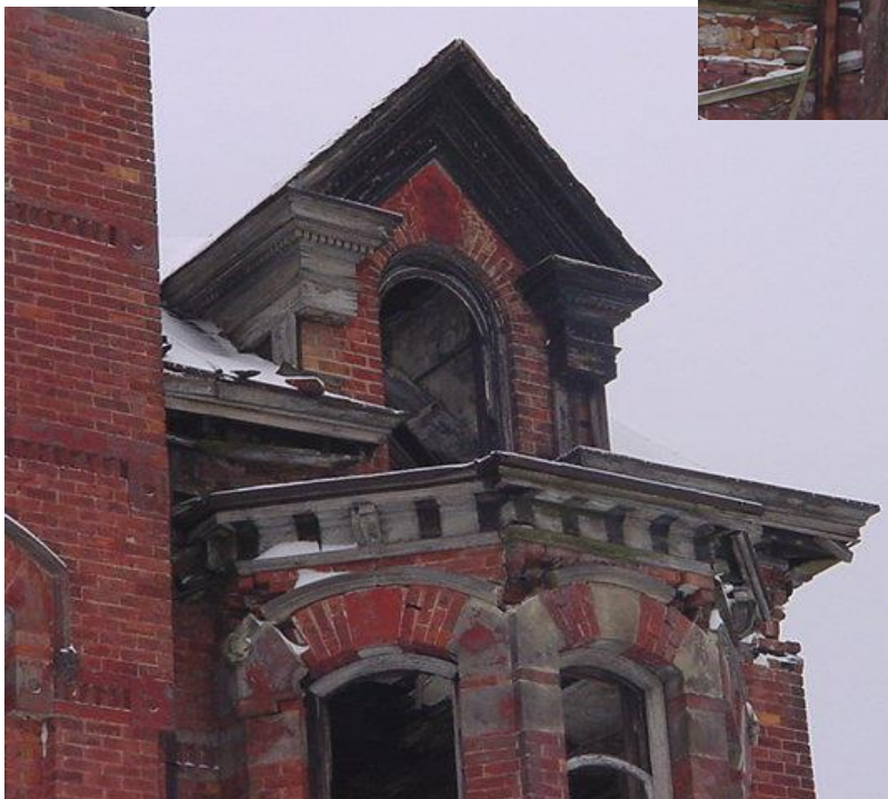
96-104 Edmund Place, detail of a side dormer with return cornice, arched window, bay window cornice and arched window lintel.
