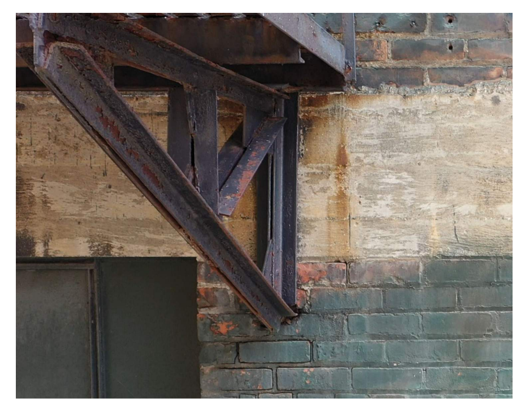
P-6 DETERIORATED BRICK AT EGRESS STAIR CONNECTIONS
