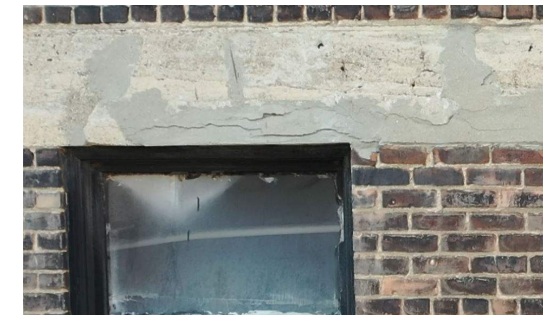
P-3 SPALLING CONCRETE AT CONCRETE BEAM ABOVE WINDOW
