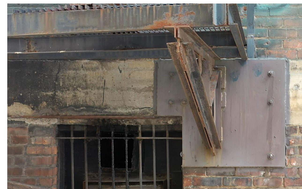
P-5 EXPOSED REINFORCEMENT ABOVE WINDOW AT STAIR CONNECTION
