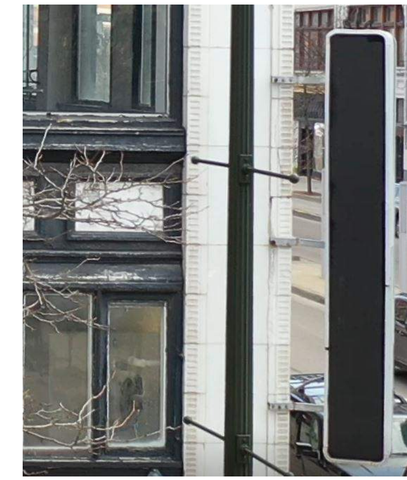
P-6 CRACKING IN BILLBOARD ATTACHMENT AT TC CORNER
