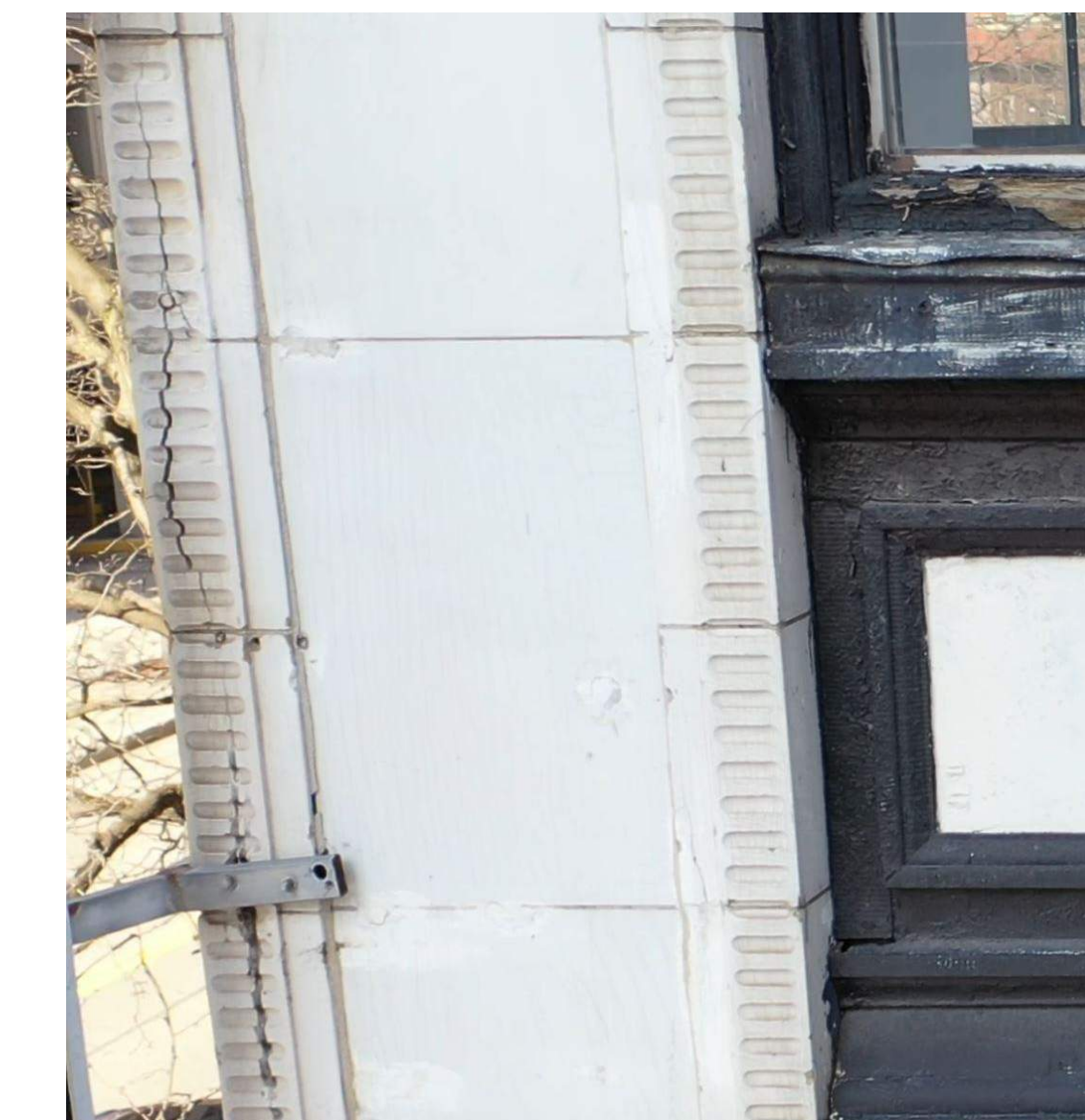
P-6 CRACKING IN BILBOARD ATTACHMENT AT TC CORNER
