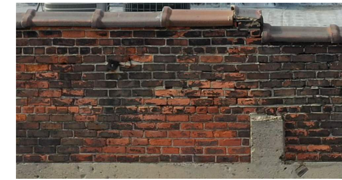
P-1 BROKEN AND DISPLACED COPING STONES AND BRICK DETERIORATION
