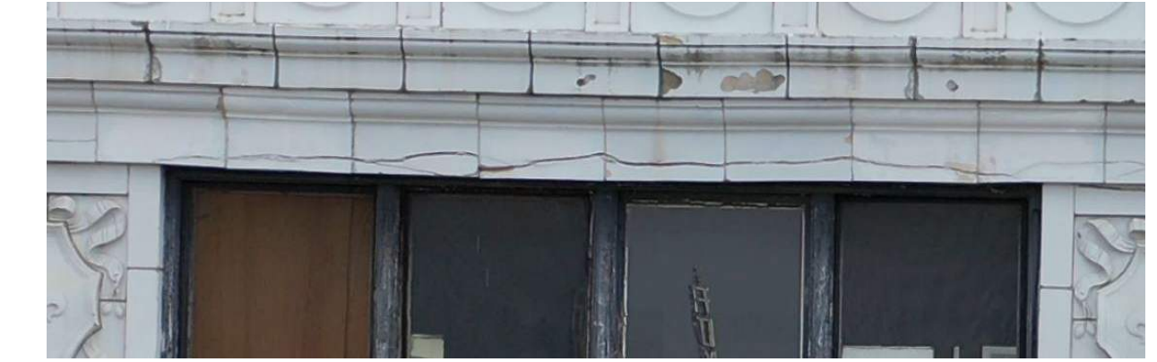
P-2 BROKEN TERRA COTTA ABOVE UPPER WINDOW OPENING
