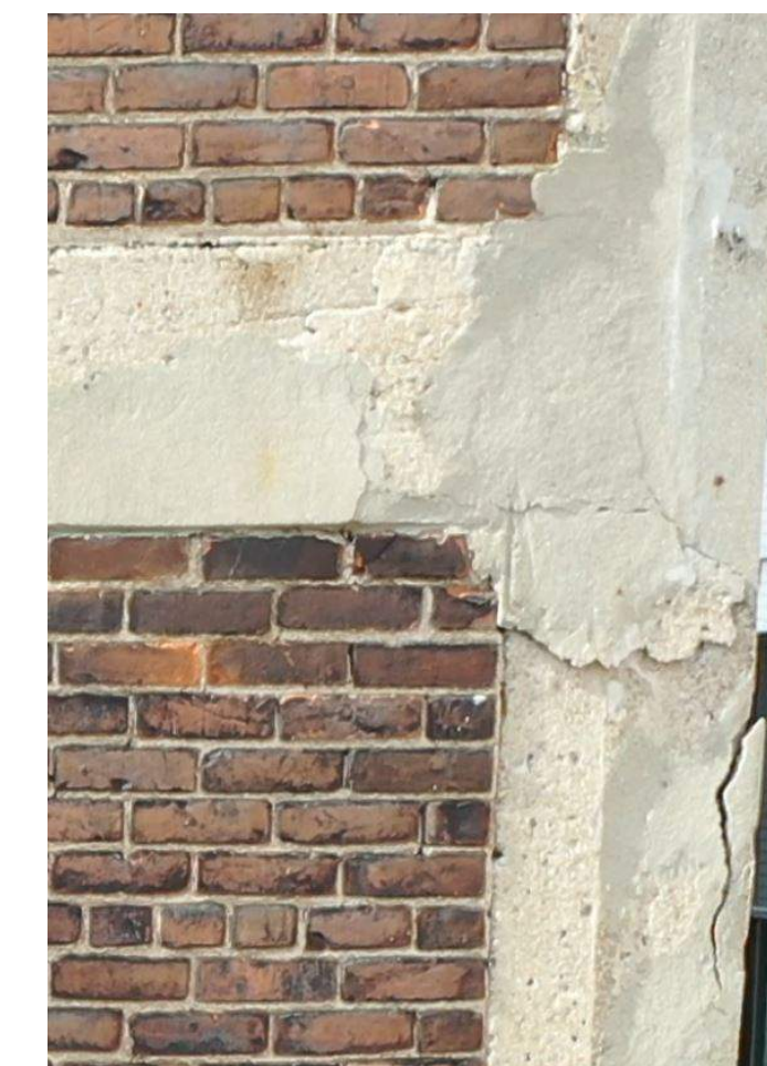
P-4 SPALLING CONCRETE AT CONCRETE COLUMN
