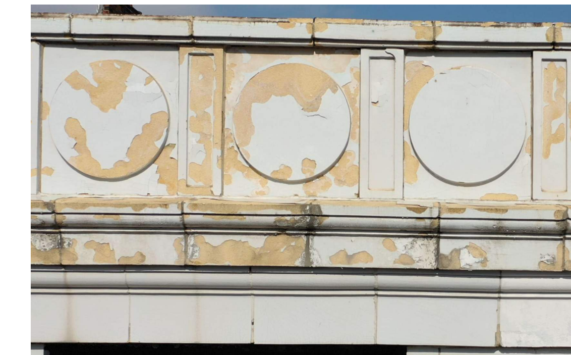
P-1 SPALLING TERRA COTTA UNDER PARAPET STONES
