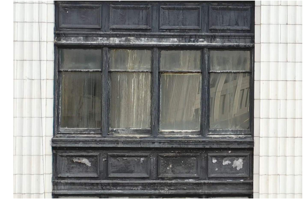
P-4 PEELING PAINT AT METAL PAN BETWEEN WINDOWS
