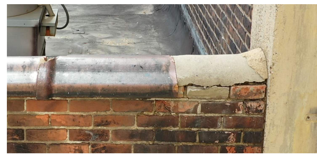
P-1 BROKEN AND MISSING COPING STONES AT LOWER PARAPET
