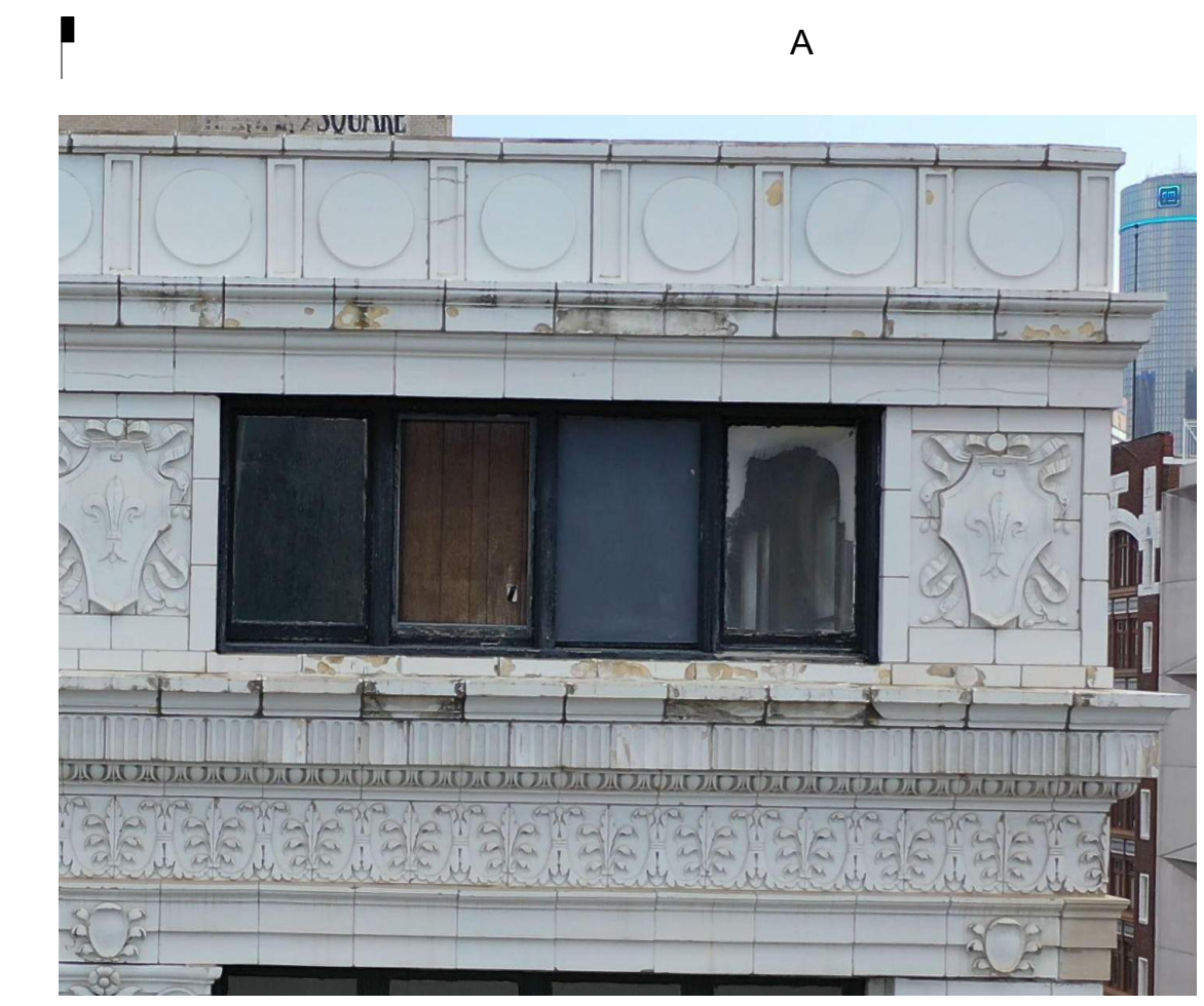
P-1 SPALLING TERRA COTTA AT UPPER WATER TABLE AND PARAPET
