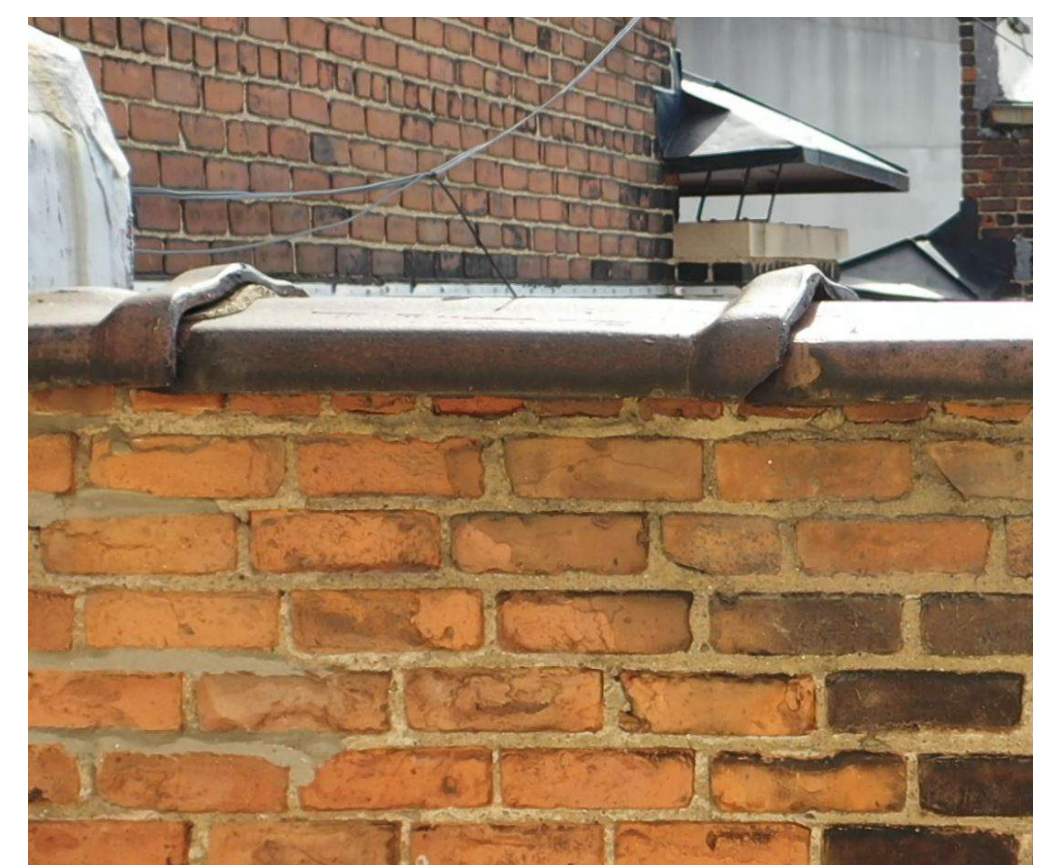
P-2 DISPLACED COPING STONES AND BRICK DETERIORATION
