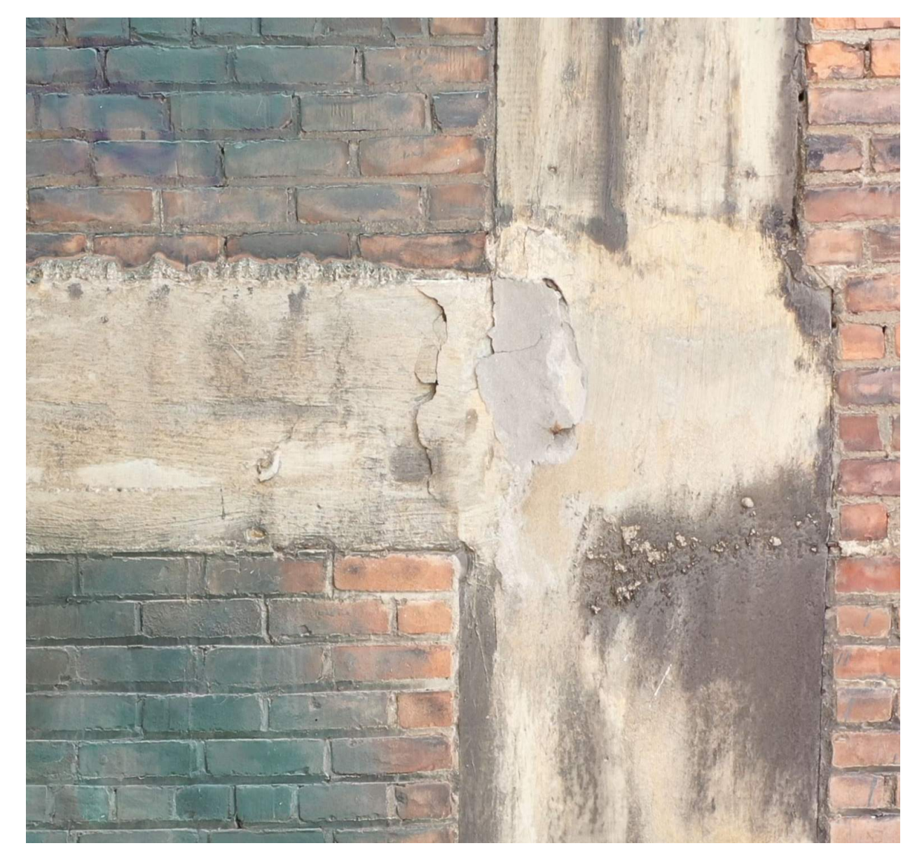
P-3 SPALLING CONCRETE AT COLUMN AND BEAMS
