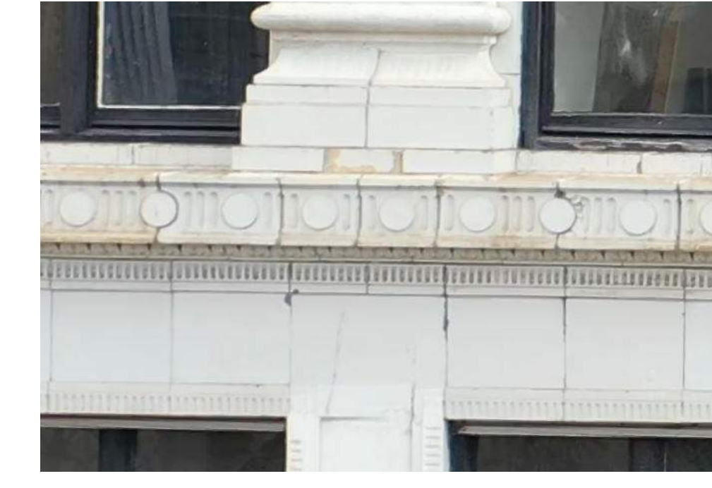
P-3 SPALLING TERRA COTTA AT LOWER WATER TABLE
