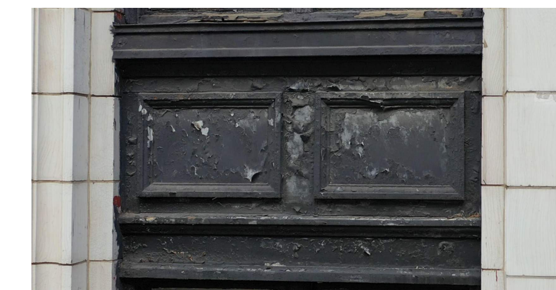
P-4 PEELING PAINT AT METAL PAN BETWEEN WINDOWS
