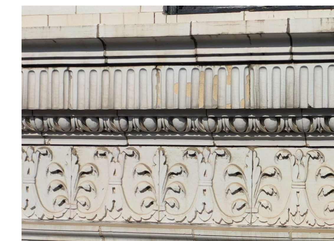
P-5 SPALLING TERRA COTTA AT LOWER WATER TABLE
