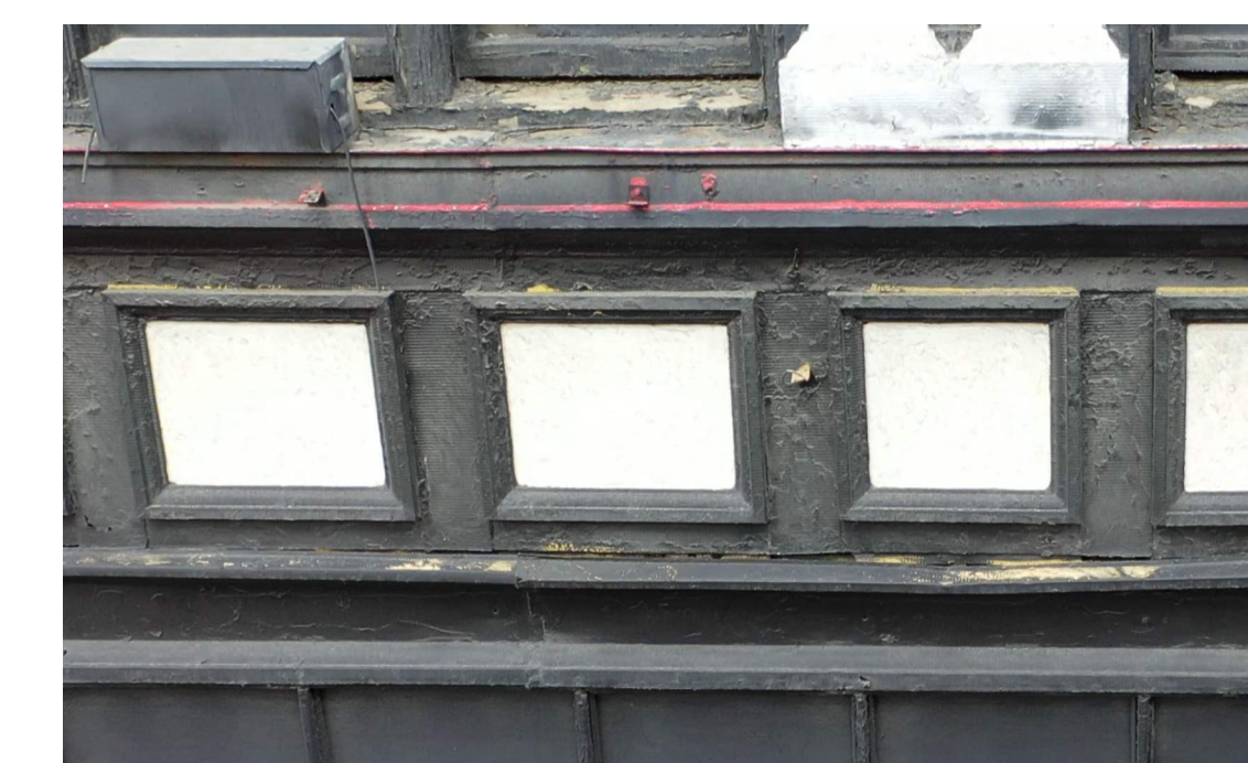
P-3 DISPLACEMENT AT STOREFRONT WINDOWS
