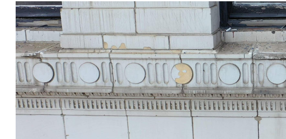
P-2 SPALLING TERRA COTTA AT UPPER WATER TABLE
