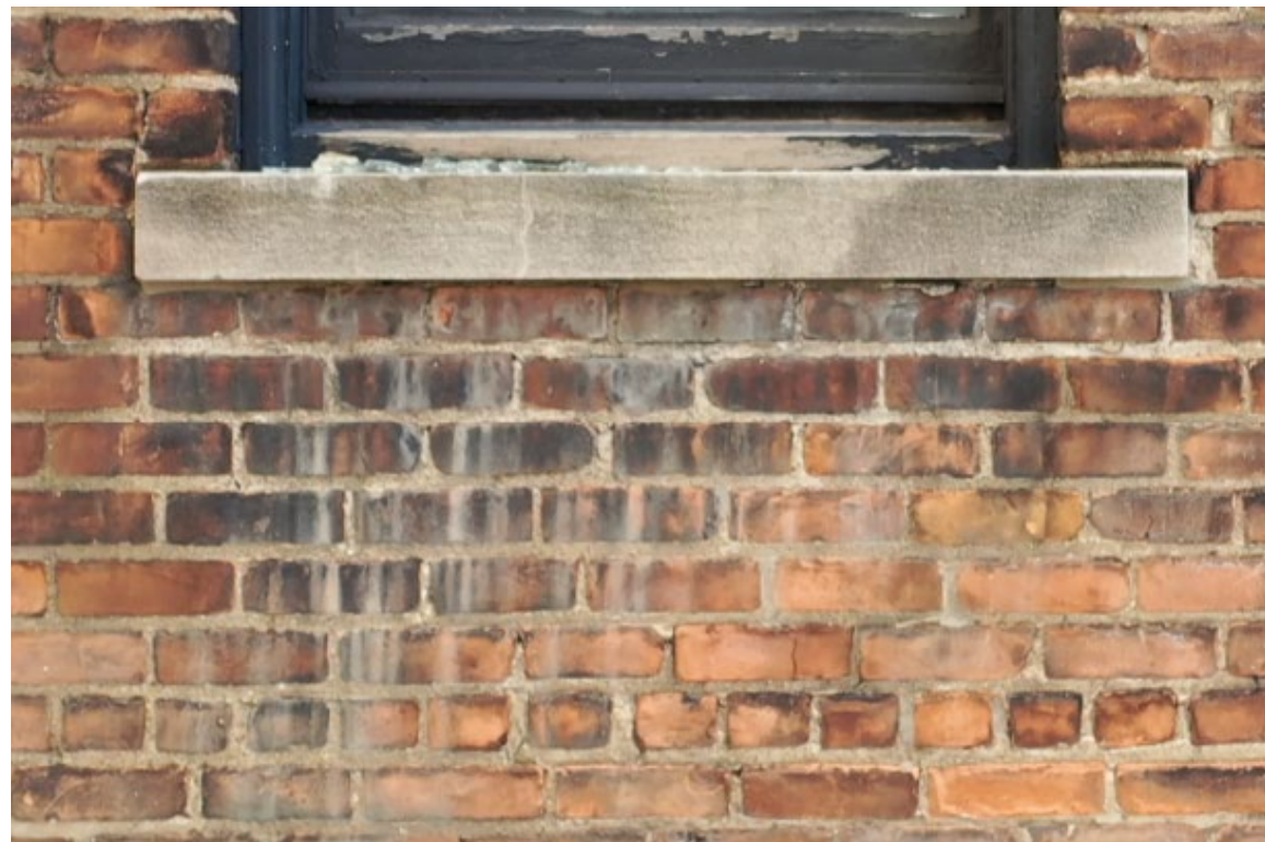
Example of typical brick efflorescence and deterioration, April 2023
