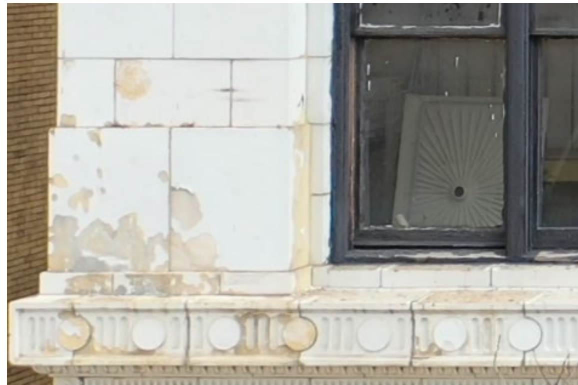
Example of typical terracotta delamination, April 2023
