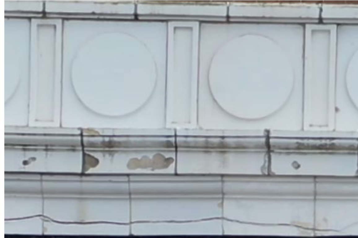
Example of terracotta cracking and delamination at water table, April 2023
