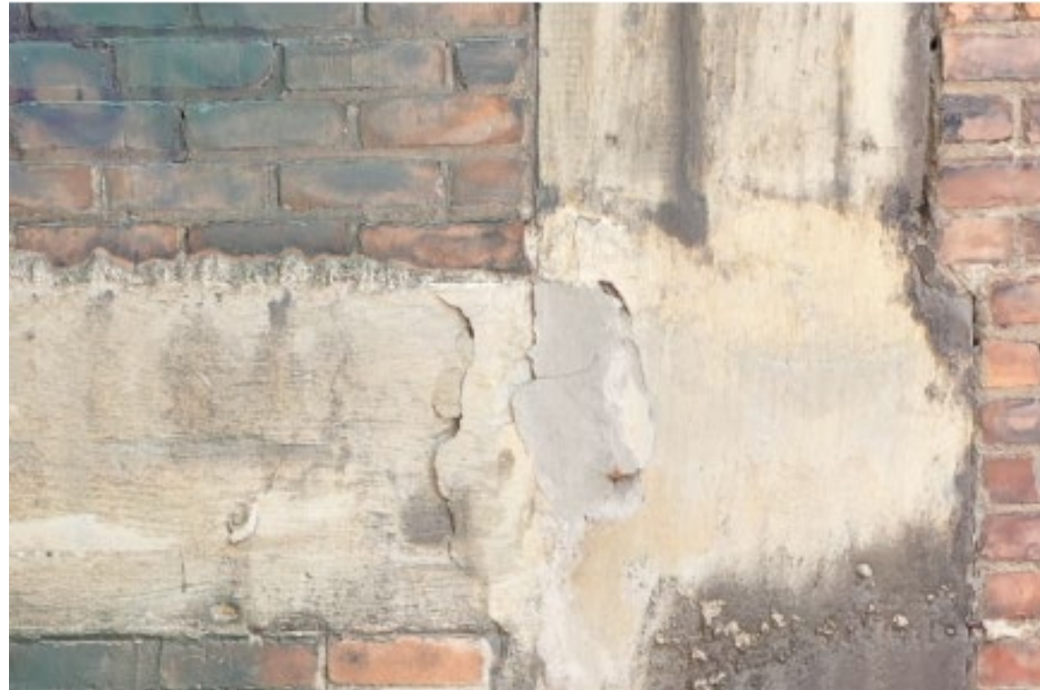
Example of exposed concrete structure spalling, April 2023
