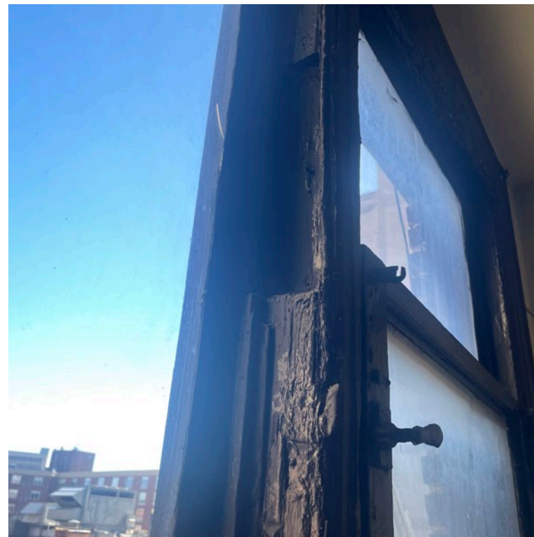
TYPICAL OVERALL WOOD CONDITION
