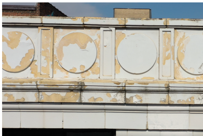
P-6 Spalling terra-cotta at parapet and upper water table
