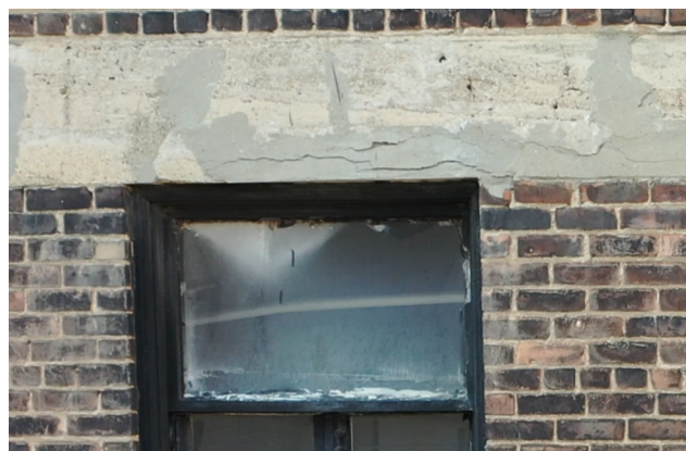
P-17 Spalling along patched concrete column
