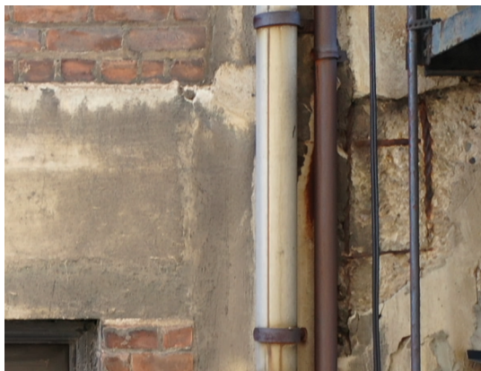
P-12 Spalled concrete at building joint between columns
