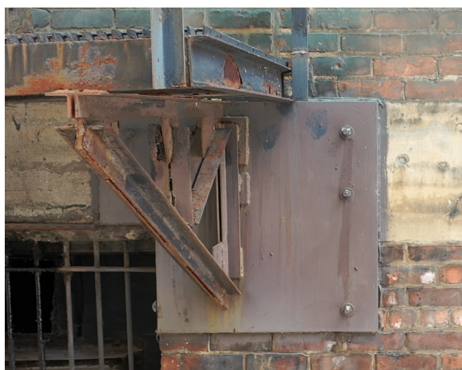
P-9 Corrosion at fire escape steel
