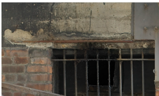
P-11 Reinforcement visible above window at spalled concrete
