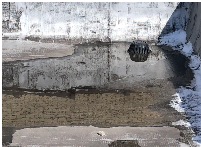
P-21 Poor drainage and ponding at roof
