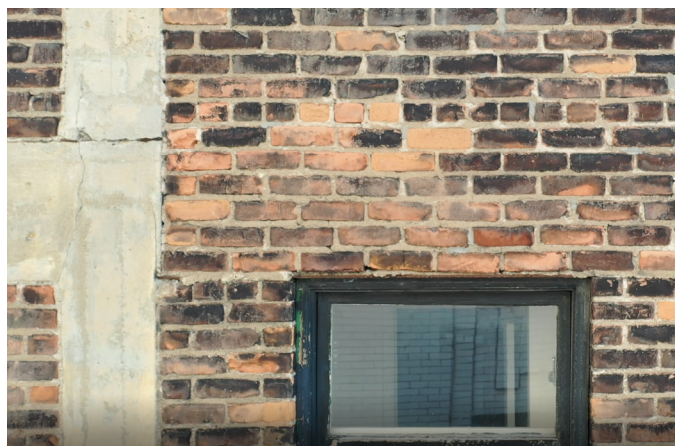
P-8 Rust jacking of brick above corroded steel lintels
