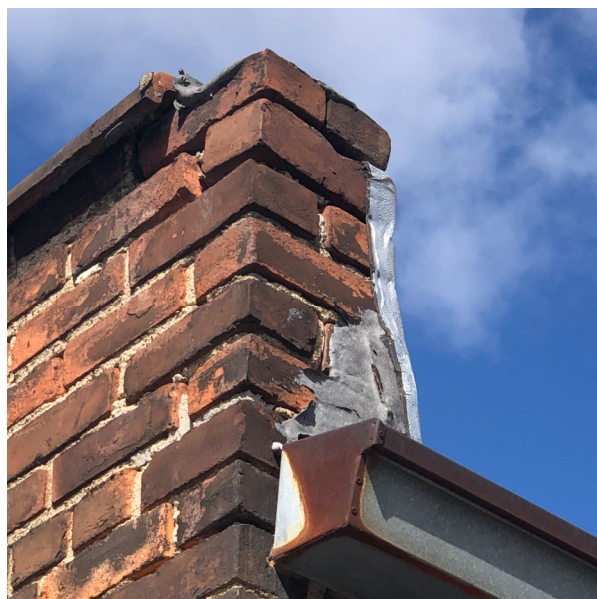
P-22 Broken coping stones and deteriorated mortar joints at elevator shaft
