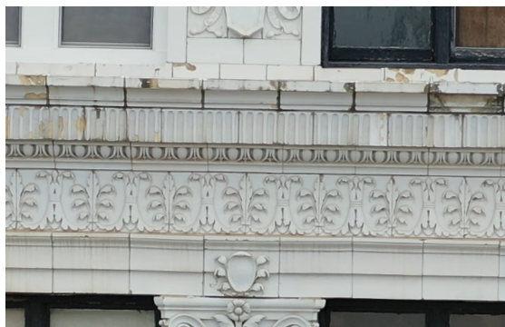
P-1 Spalling of terra-cotta below water table
