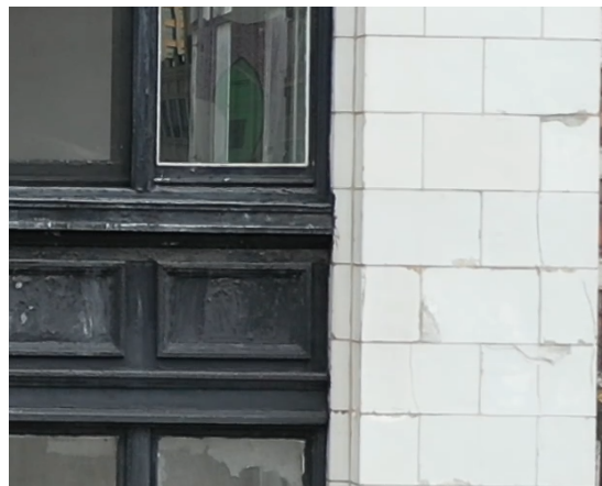
P-4 Cracks in corner terra-cotta due to corroded embedded steel
