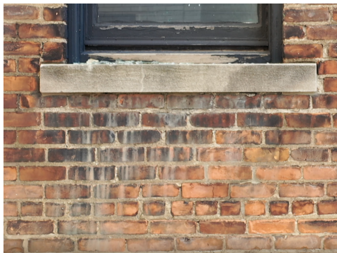
P-7 Efflorescence at brick below window sill
