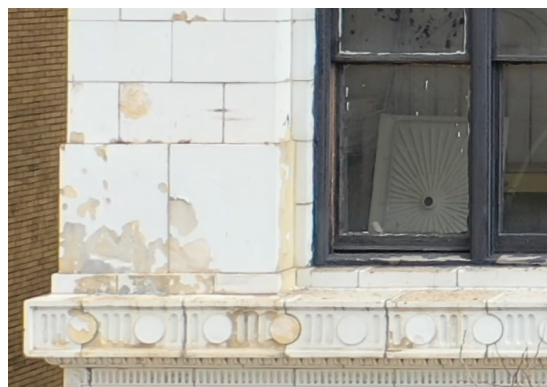
P-2 Delamination of terra-cotta around lower water tables
