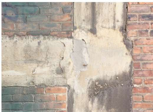
P-10 Spalling of exposed concrete frame
