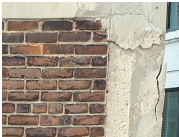
P-16 Spalling along patched concrete column
