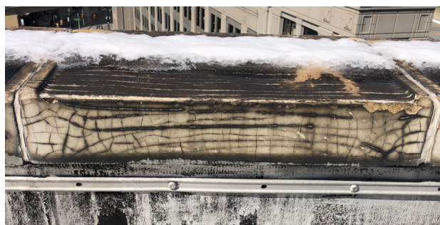
P-19 Delaminating coping stones and deteriorated joints
