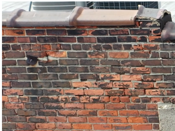
P-18 Broken and displaced coping stones at parapet
