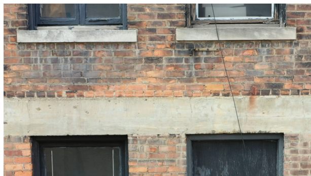
P-13 Brick and mortar deterioration around concrete frame
