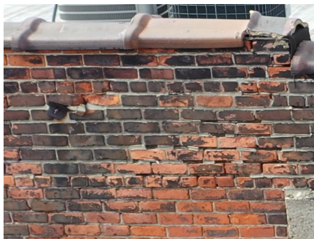
P-14 Brick and mortar deterioration below coping stones
