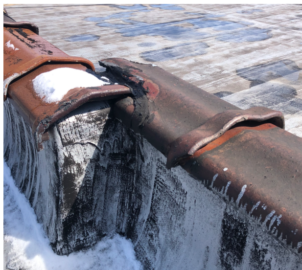
P-20 Displaced coping stones overtop flashing at building joint parapet
