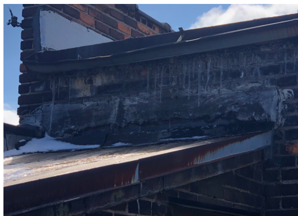
P-23 Broken gutters and deteriorated flashing below elevator roof
