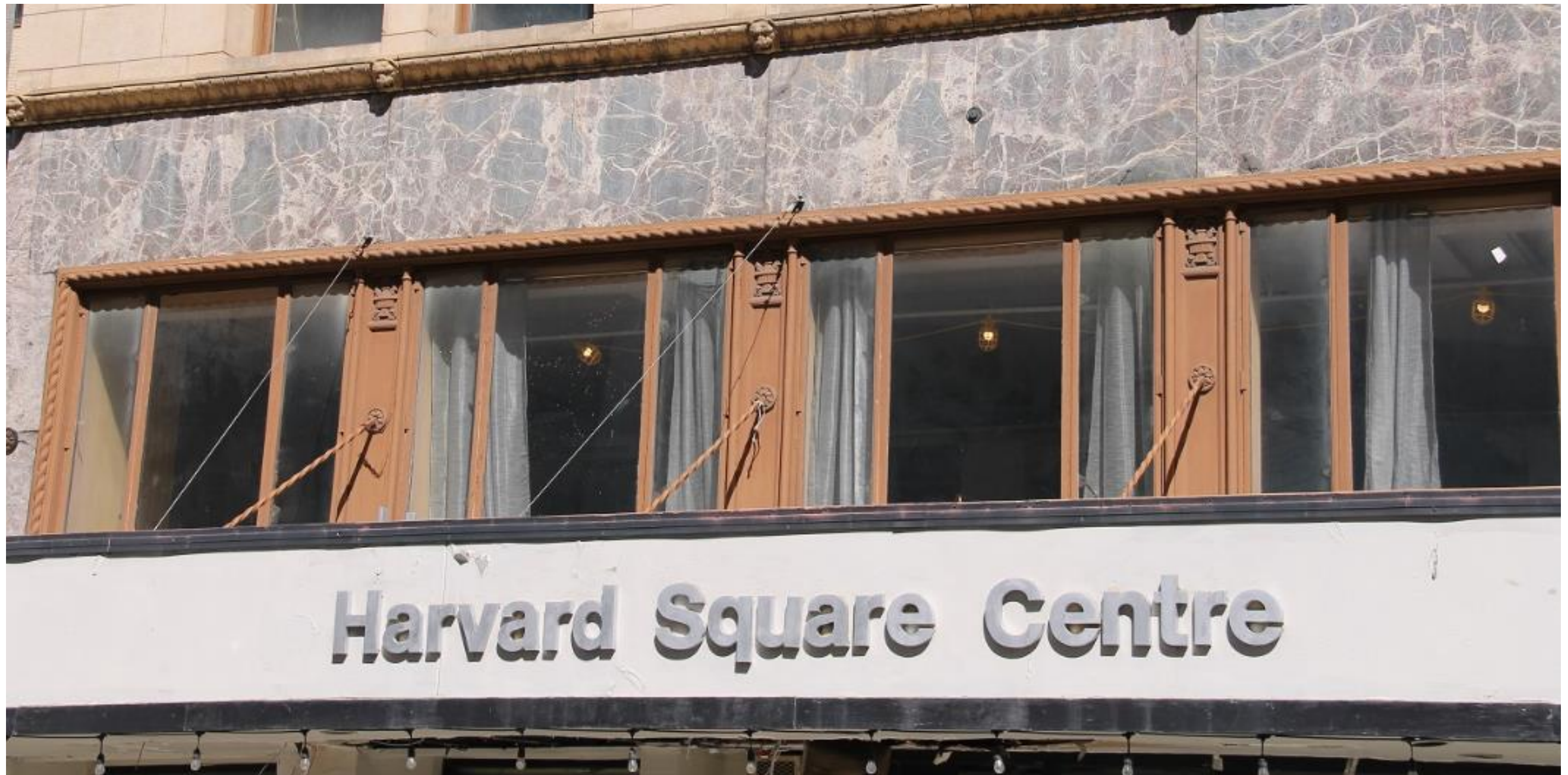
Hot rolled steel casement and fixed frames and sashes with cast iron surround, to be restored
