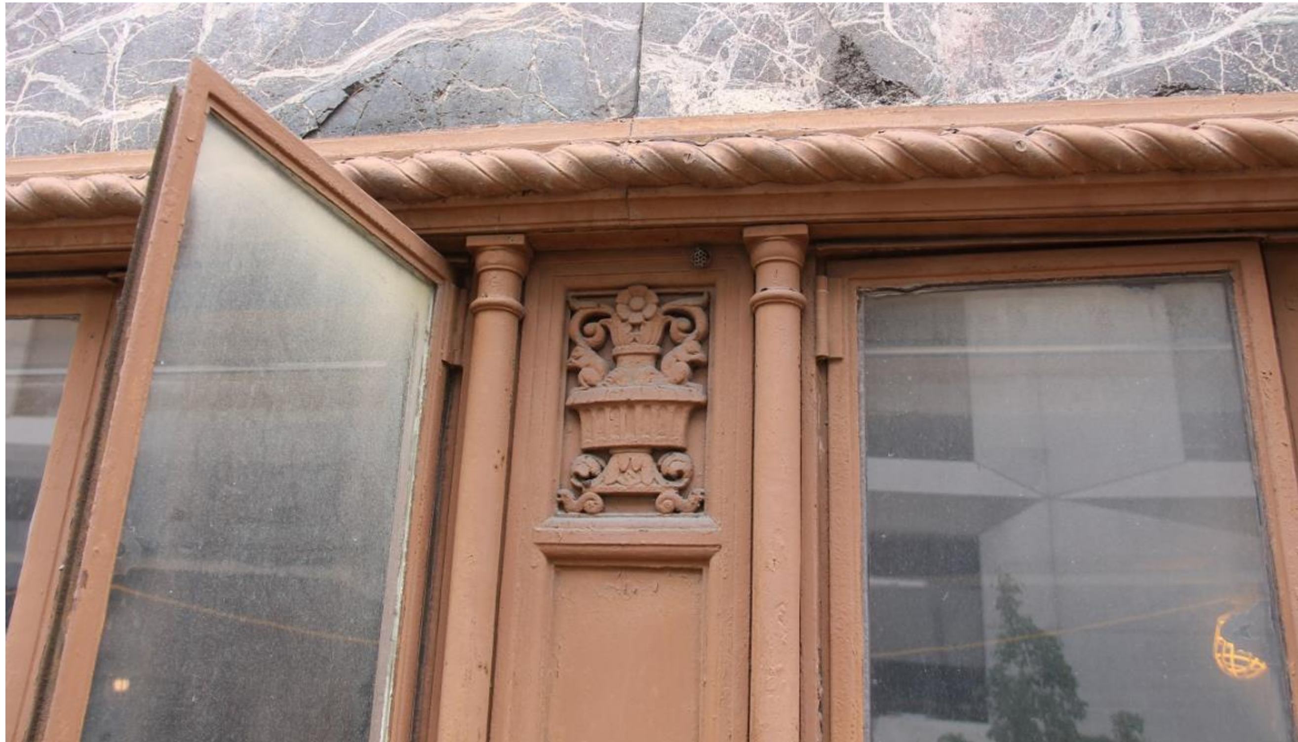
Hot rolled steel casement and fixed frames and sashes with cast iron surround, to be restored
