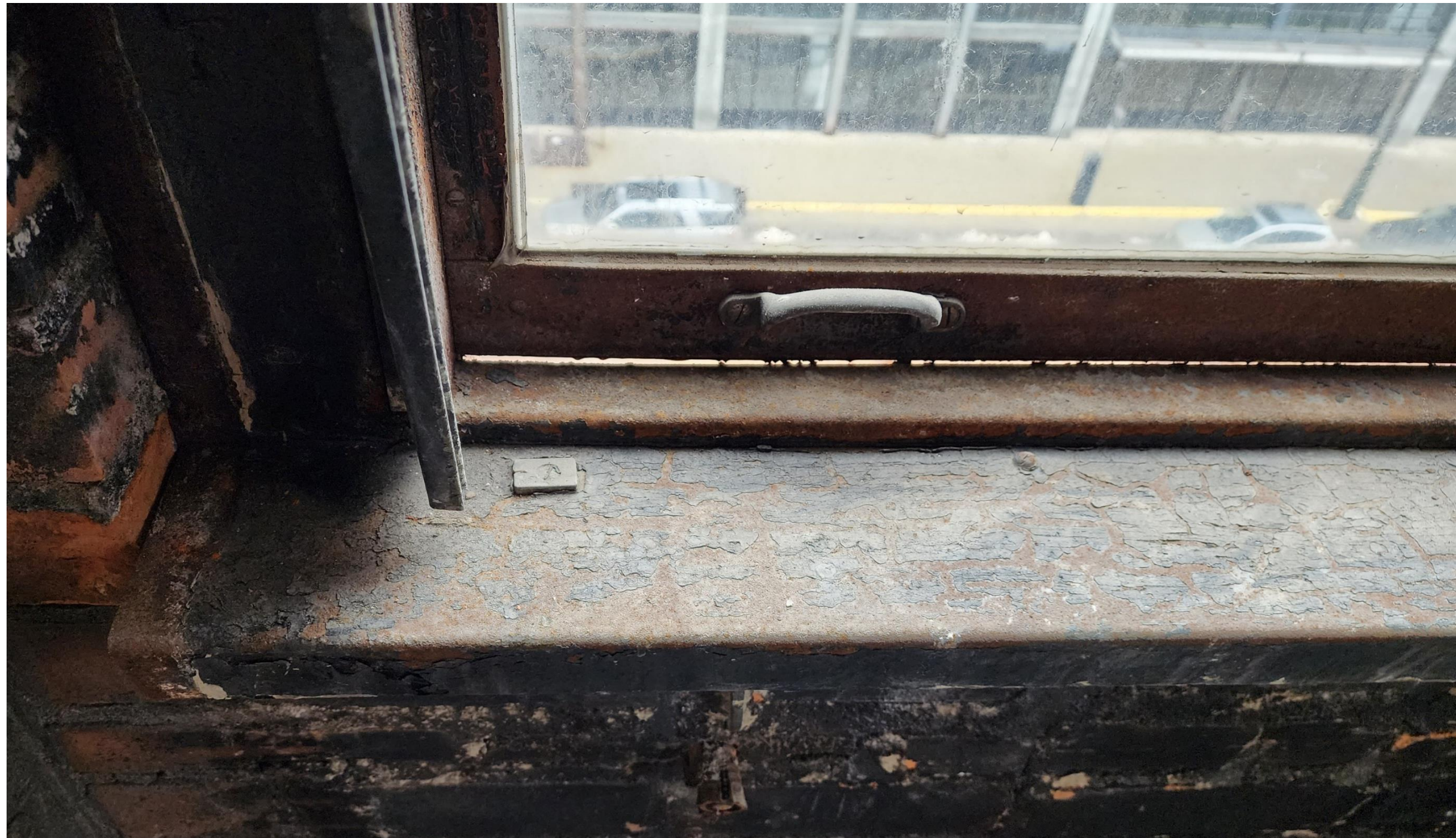
Interior view of typical cold rolled steel double-hung frame and sash, to be replaced
