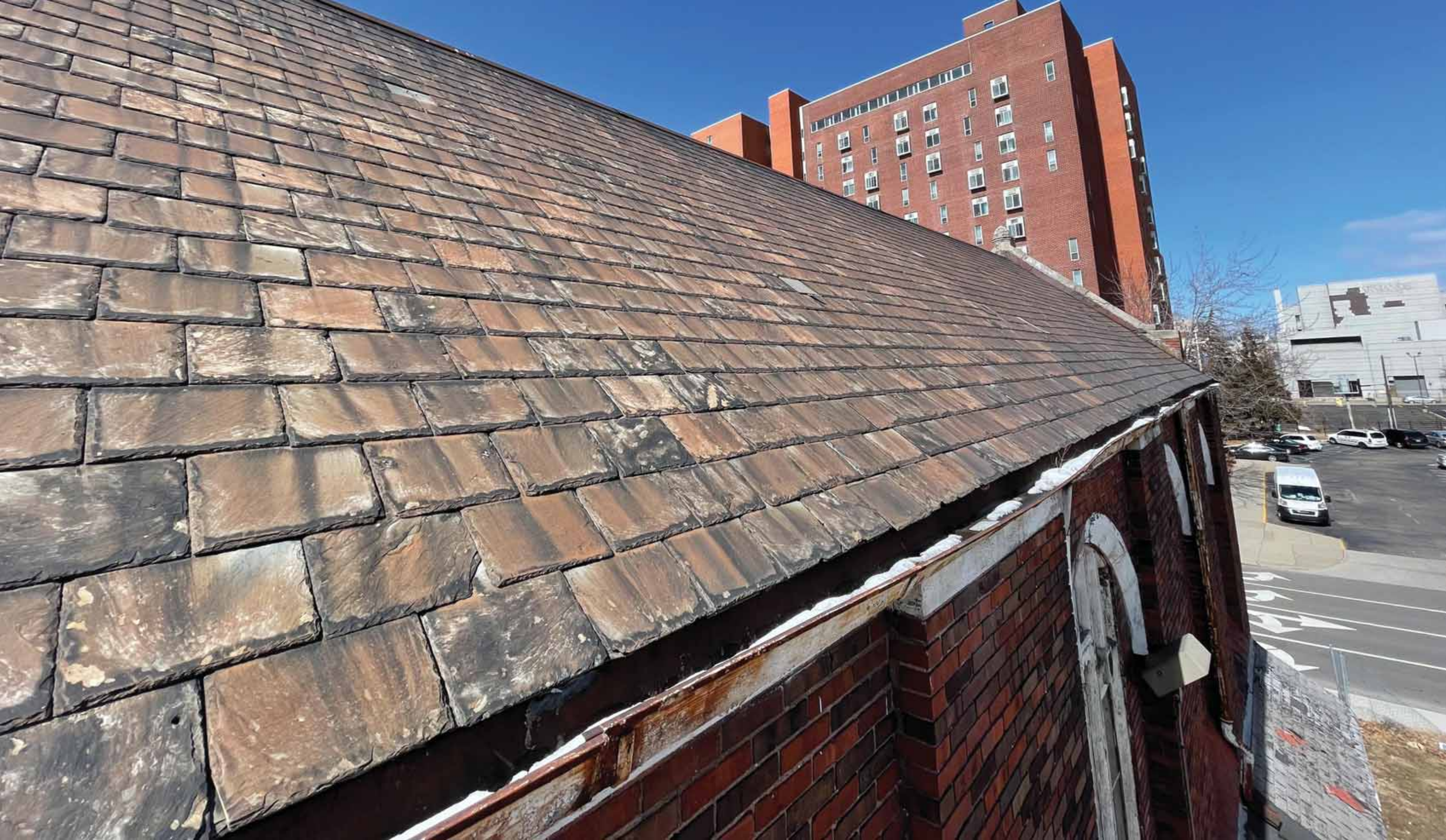
Existing Conditions, Slate is 1/6 of standard slate thickness, with delamination and sheering of tiles.
