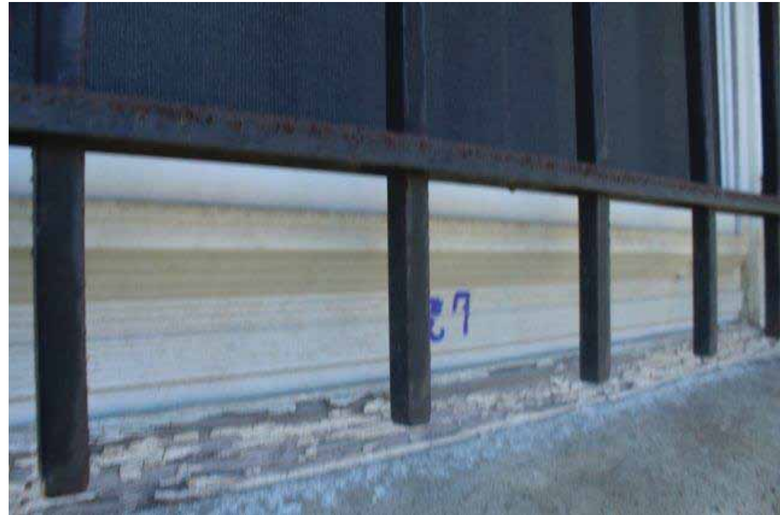
Image of window 27, vinyl replacement on wood sill. The sill is deteriorating and beginning to fail.
