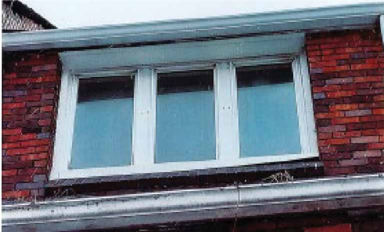
Image of window FW1, vinyl replacement in brick surround and center addition.
