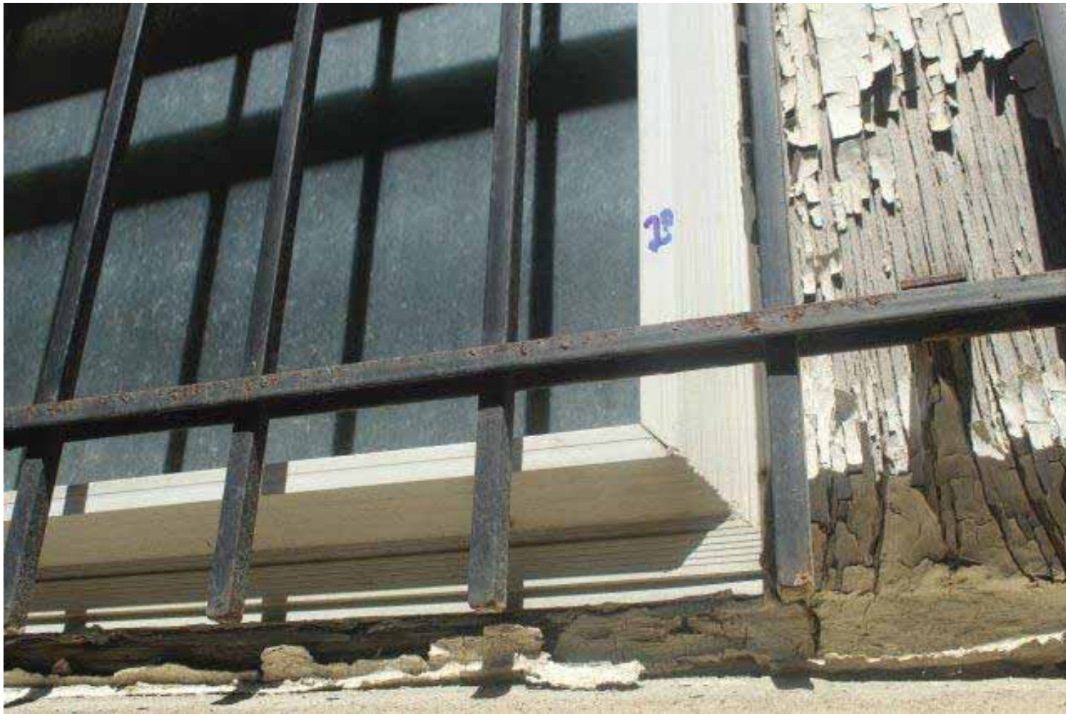
Image of window 28, vinyl replacement in wood trim. The trim is deteriorating and beginning to fail.
