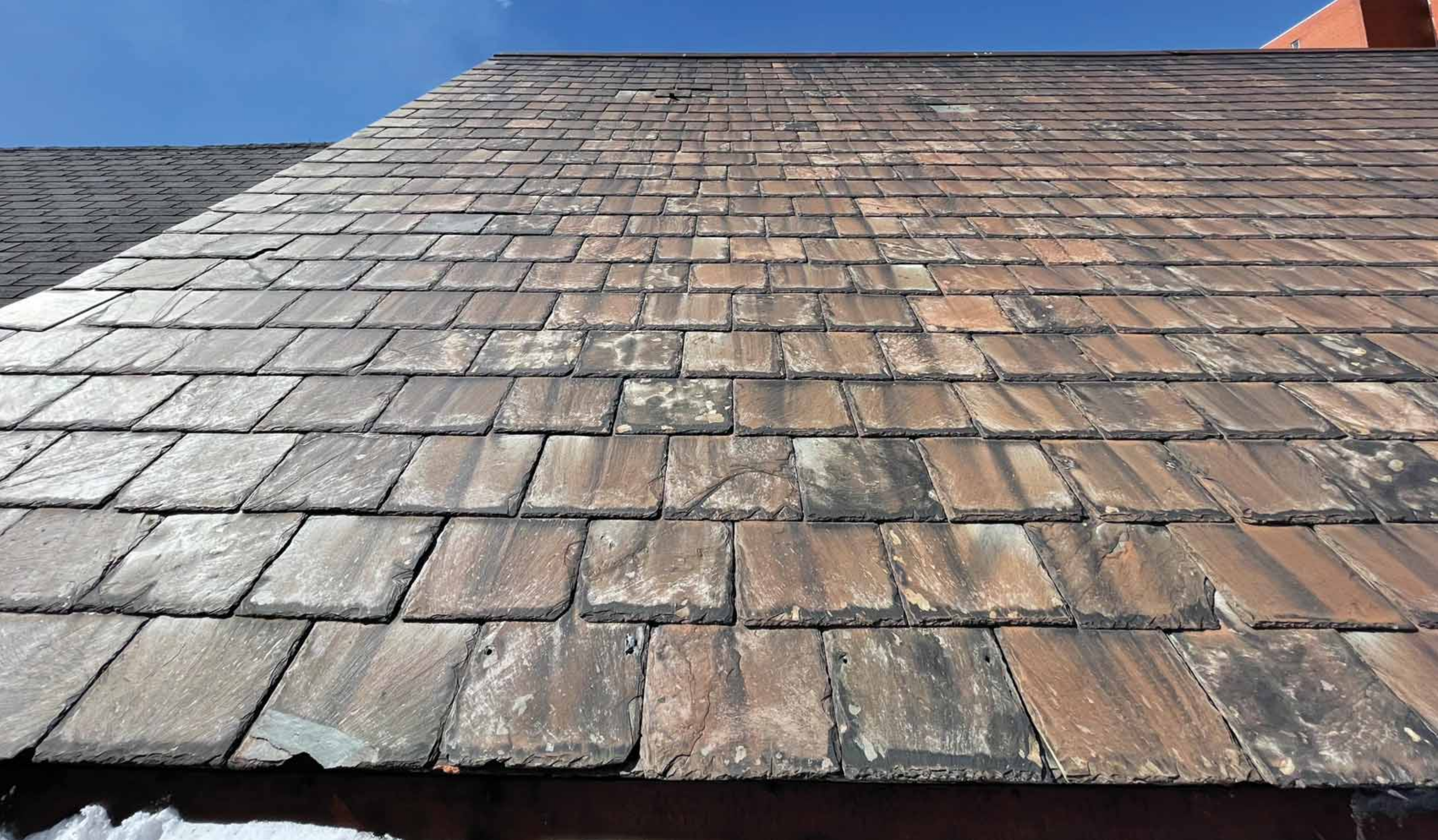
Existing Conditions : Slate is 1/6 standard thickness with visible delamination and sheering of tiles.
