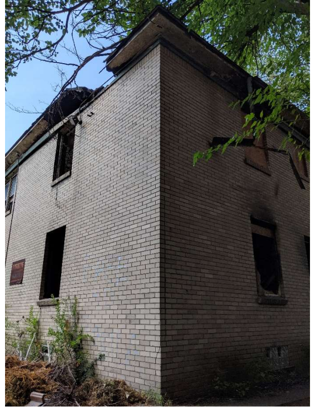
Photo 23: Exterior masonry at fire damaged wall
