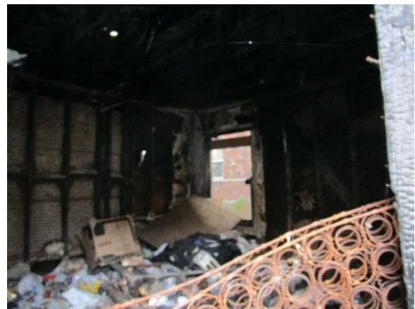
Photo 24: Interior studs at fire damaged wall
