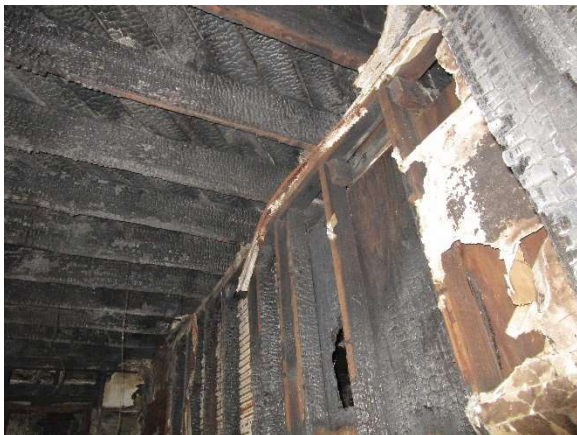
Photo 22: Interior studs and joists at fire damaged wall
