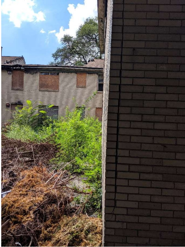
Photo 21: Bowed and separating brick cladding at fire damaged wall
