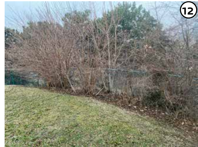
Remove all invasive shrubs here. Reset landscape edging, add topsoil, mulch, and new shrubs along fence
