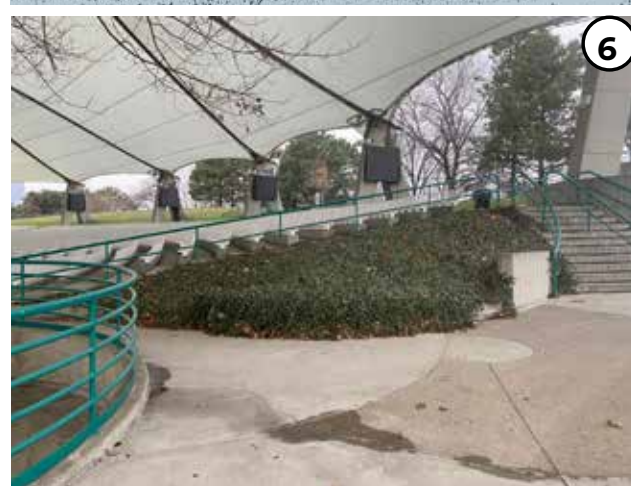
6 English Ivy is overgrown, prune back to reveal seatwall
