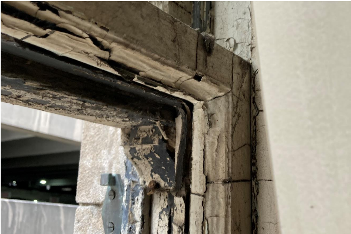
Figure #19: Interior, Alley Window Condition. 8/4/22
