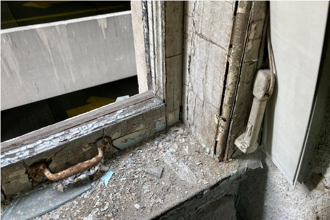
Figure #18: Interior, Alley Window condition. 8/4/22
