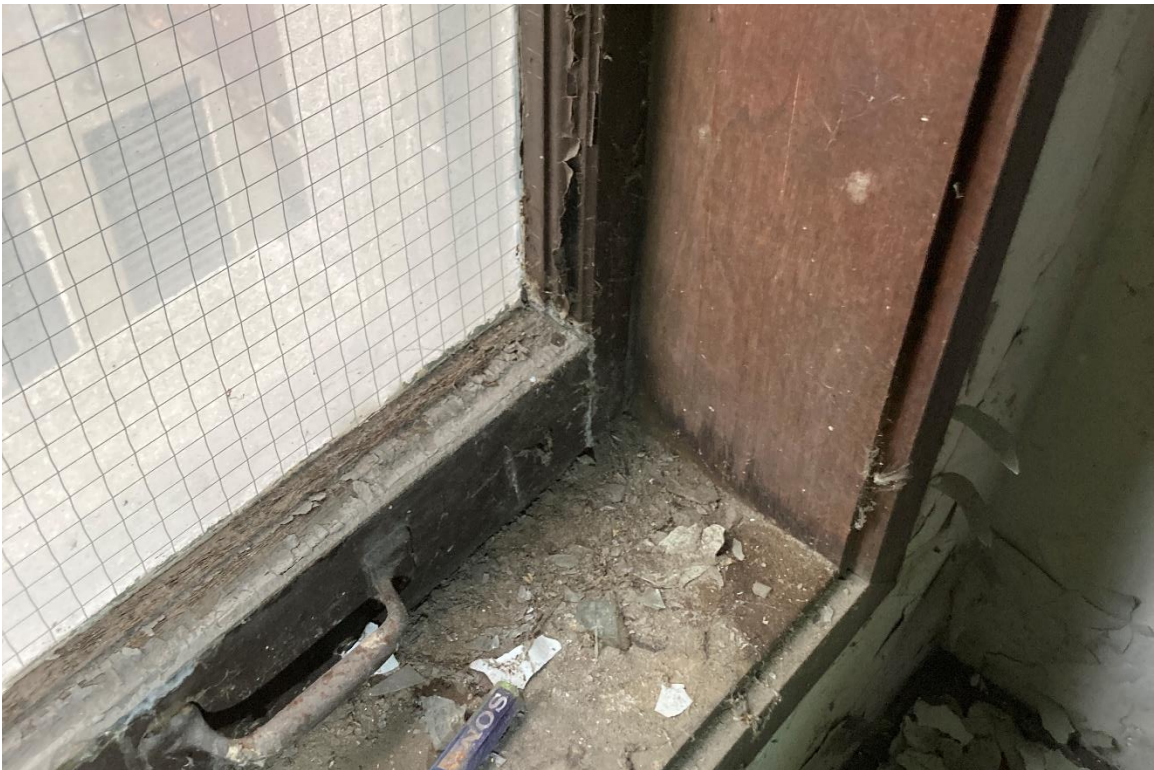
Figure #21: Interior, Alley Window Condition. 8/4/22
