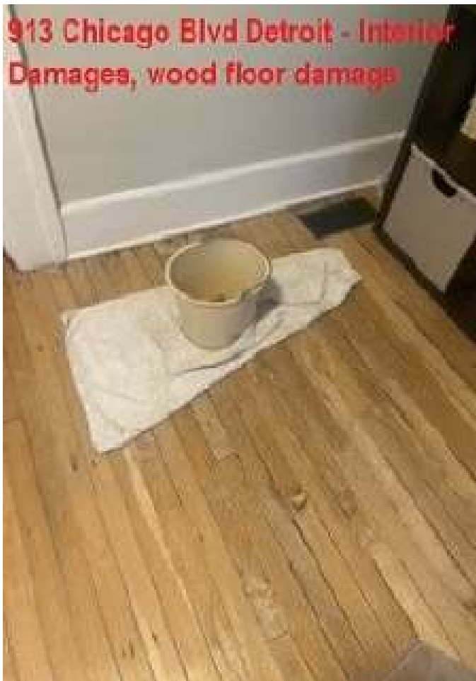
913 Chicago Blvd Detroit - Interior Damages
