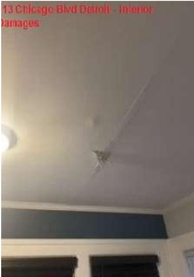
13 Chicago Blvd Detroit - Interior Damages
