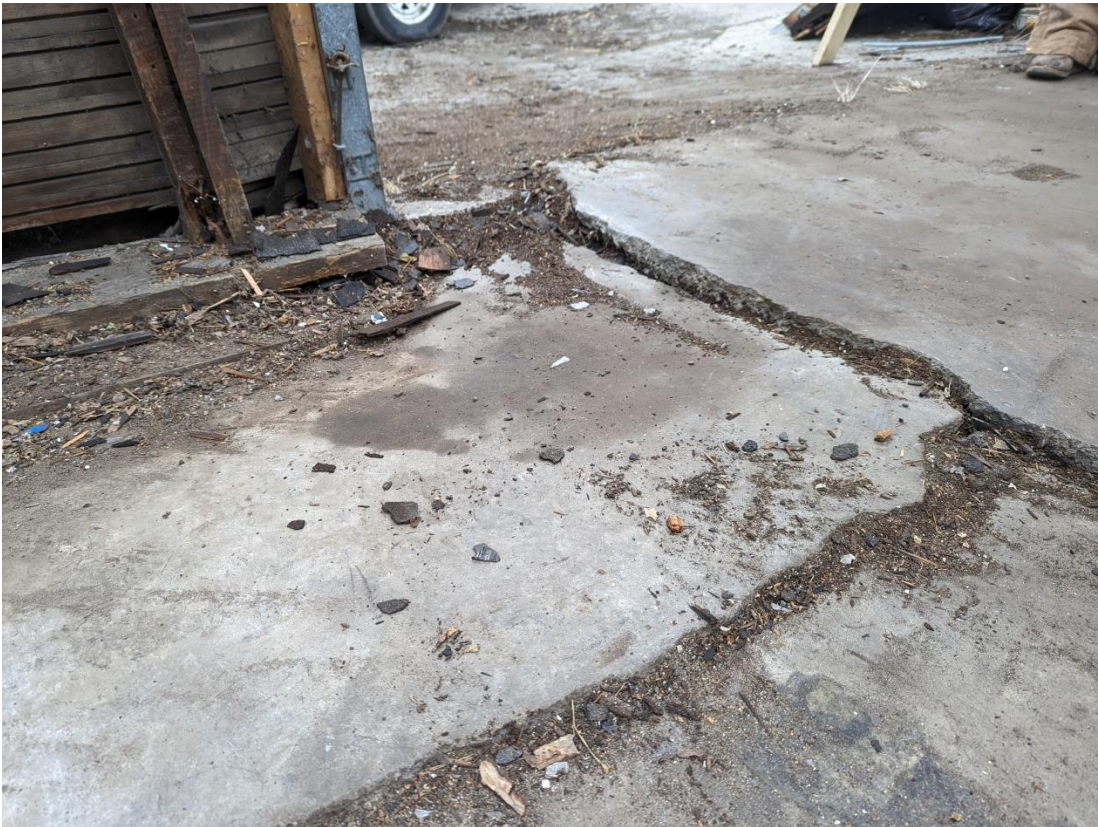
Figure 10 - Post Demolition, uneven concrete slab
