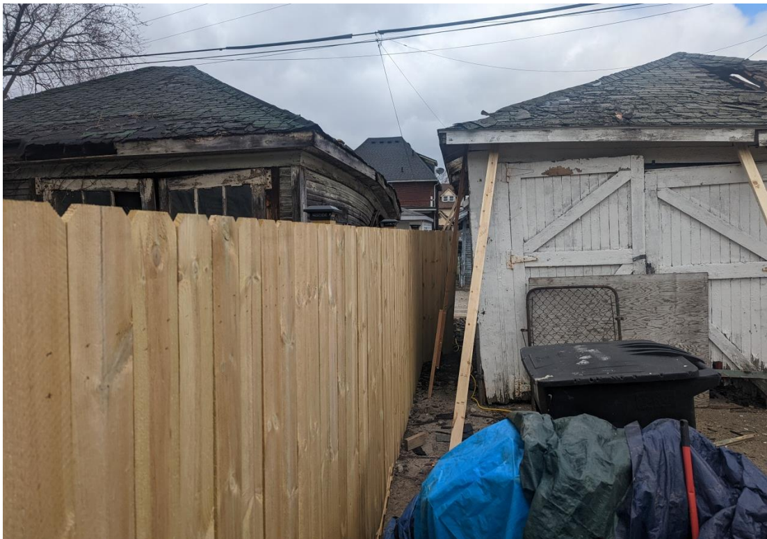
Figure 8 - Left side, near fence, of damaged garage
