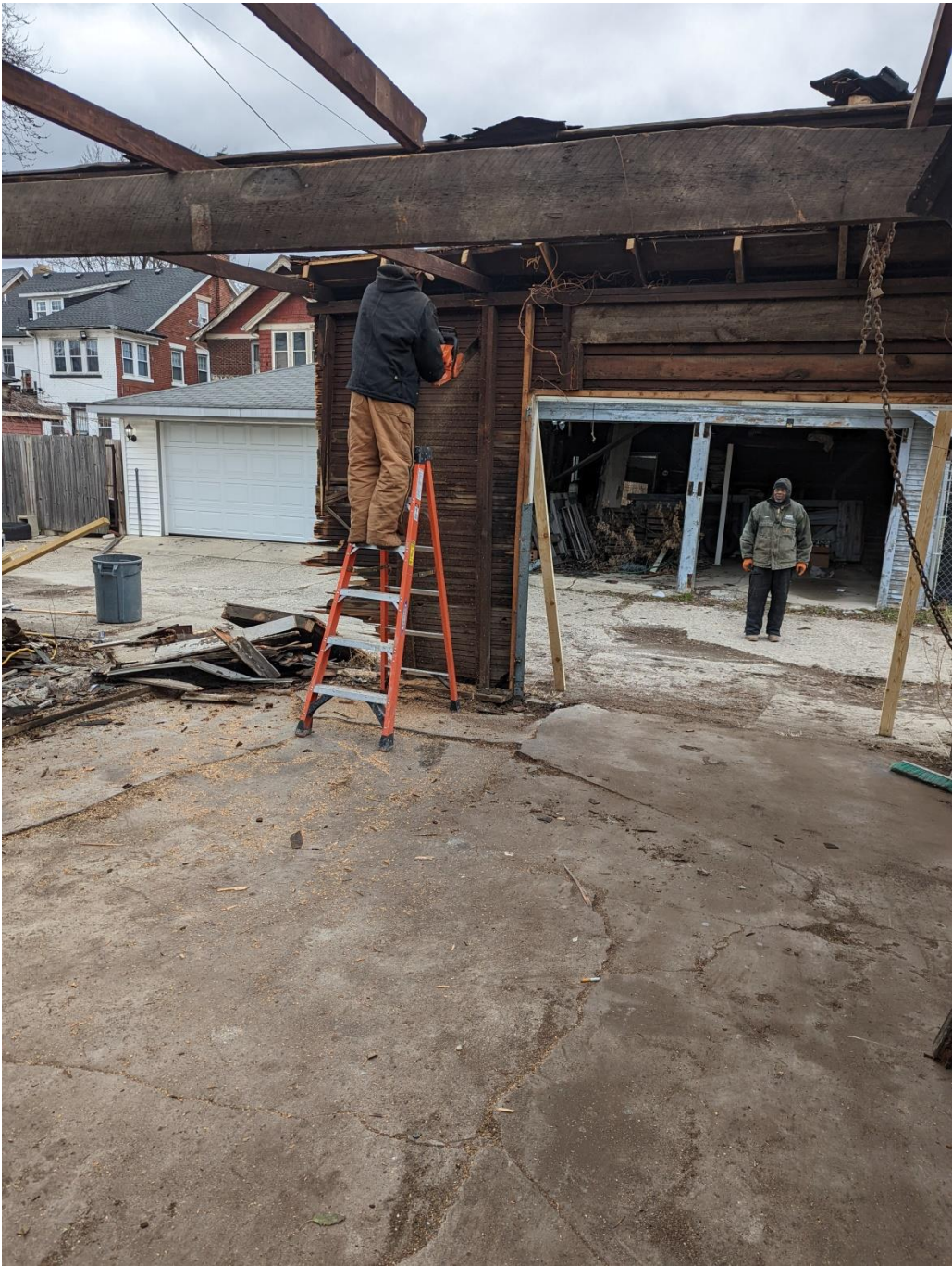
Figure 13 - Replacement garage to be erected as structure was a safety hazard and needed to be demolished
