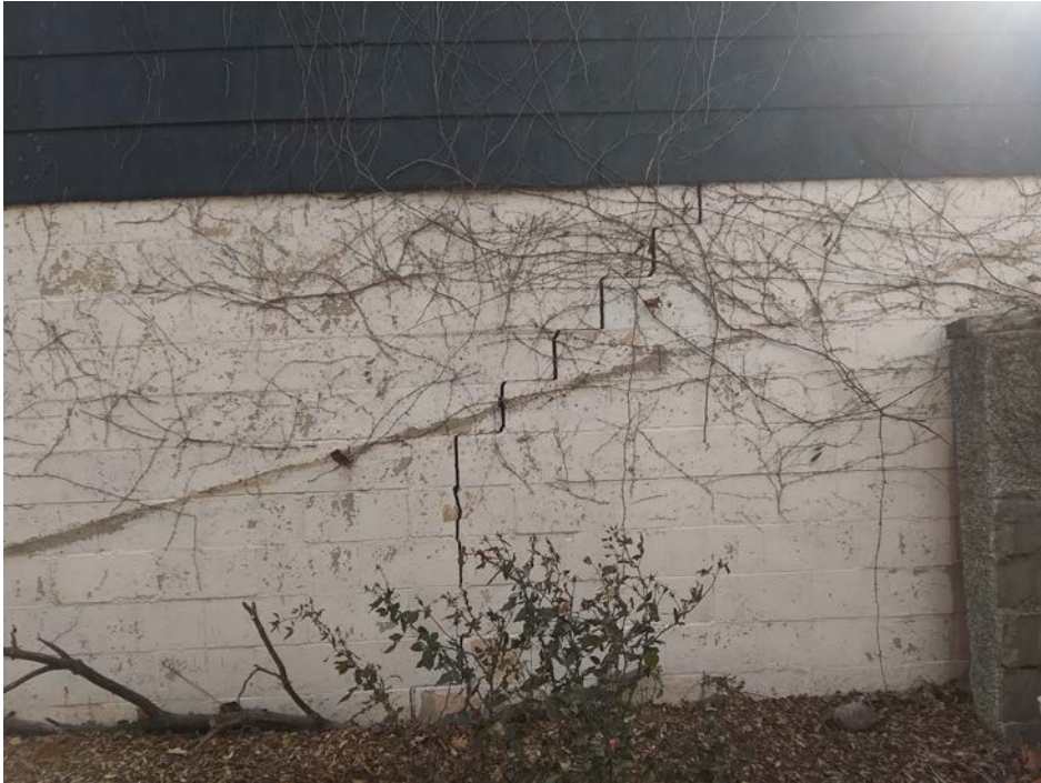
CRACKED MASONRY AT NORTH ELEVATION
