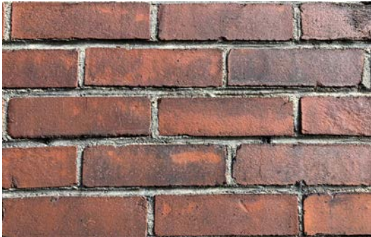
EXISTING HOUSE BRICK TO BE USED AS BASIS FOR GARAGE CMU DECORATIVE PAINT SCHEME
