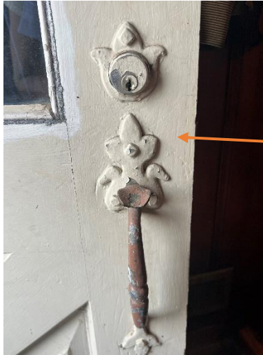
Lower lock does not work from exterior
