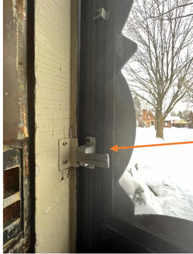
Screen door doesn't lock
