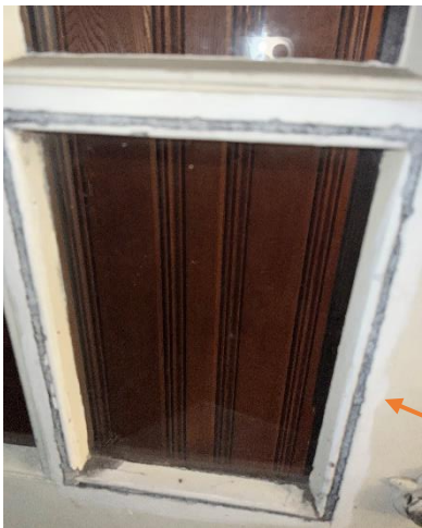
Mold growing around window pane that was replaced
