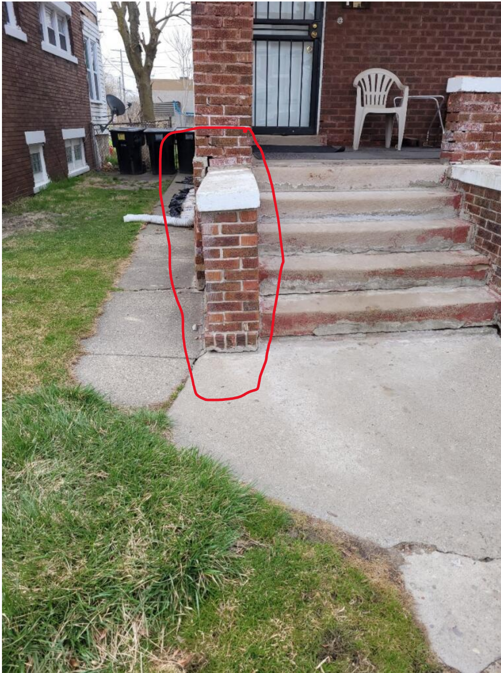
A: The wing wall is leaning to the left due to improper footing.
