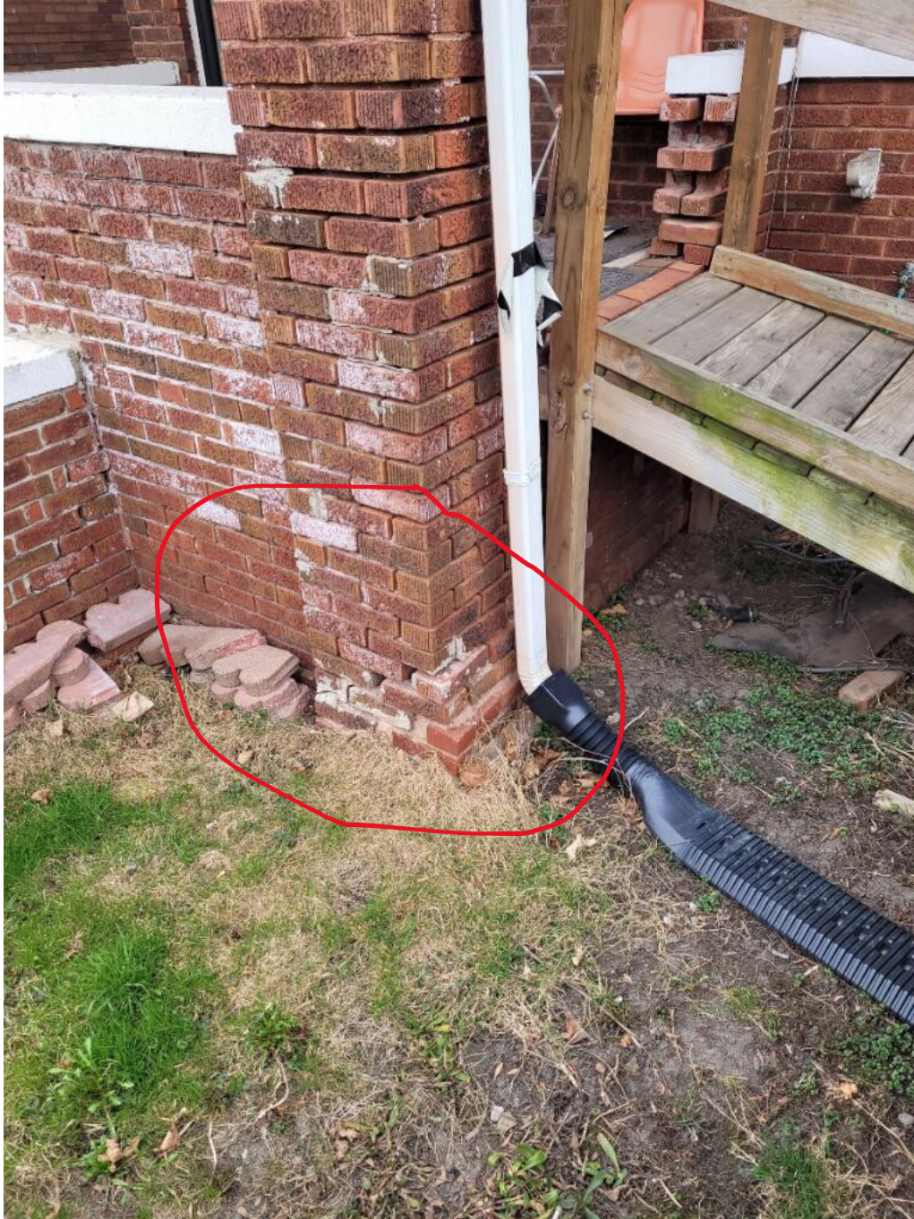
D: The brick column twisted and moved due to footing shifting. Step Crack
