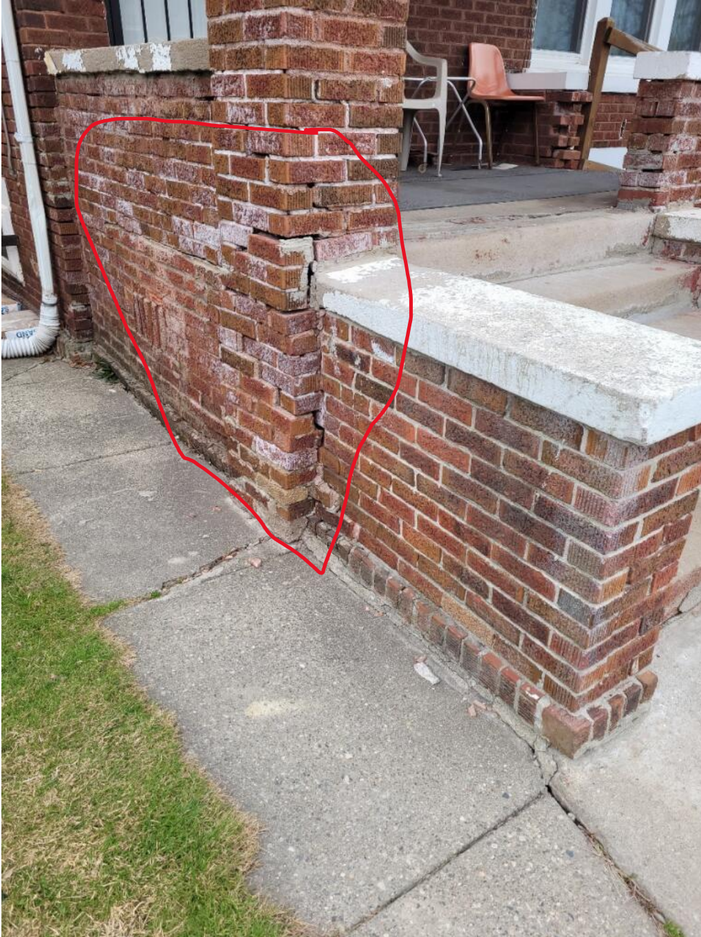
B: Column and wing wall are separating and shifting due to improper footing.
