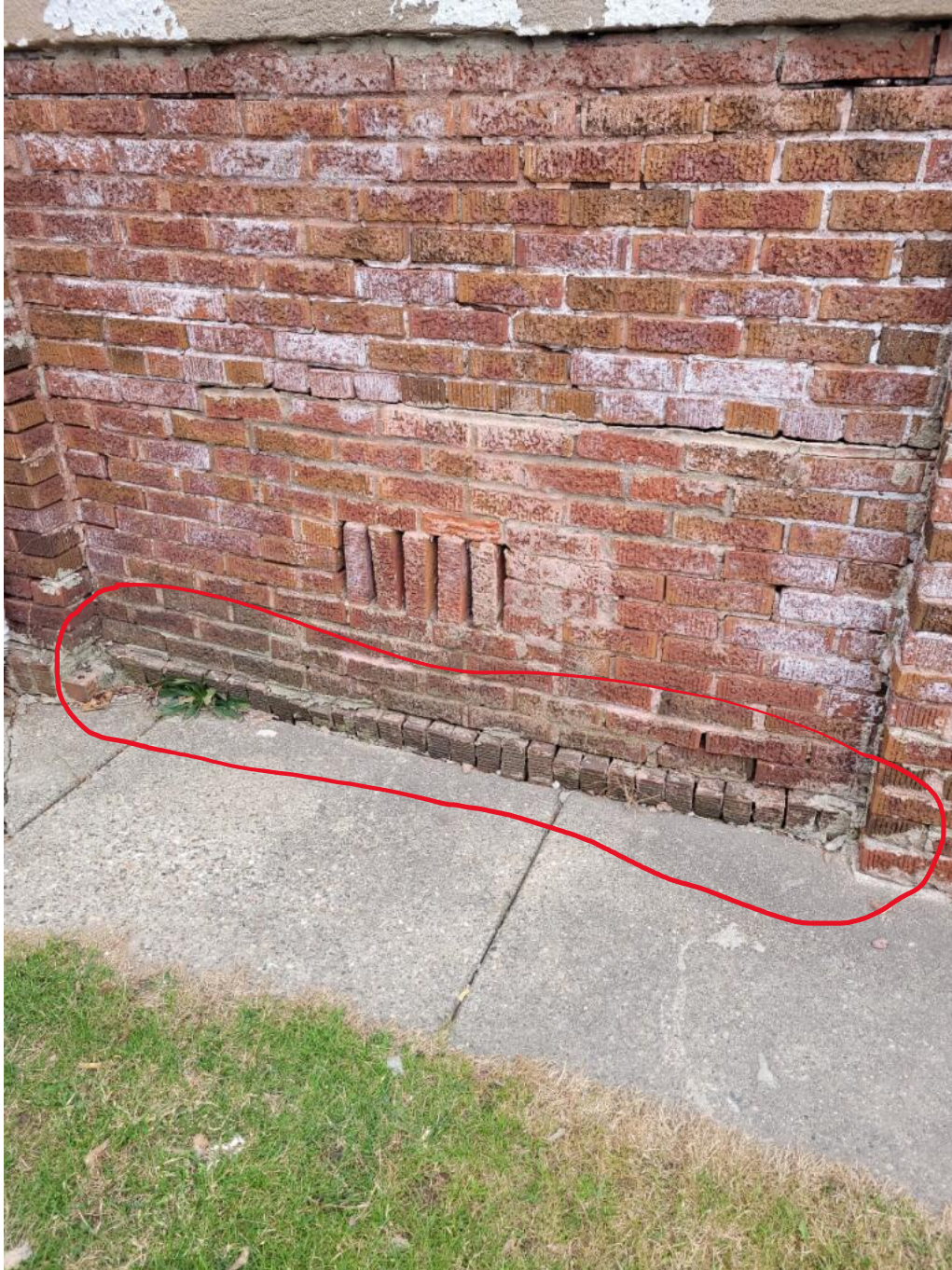
C: The porch wall has dropped down due to footing movement.
