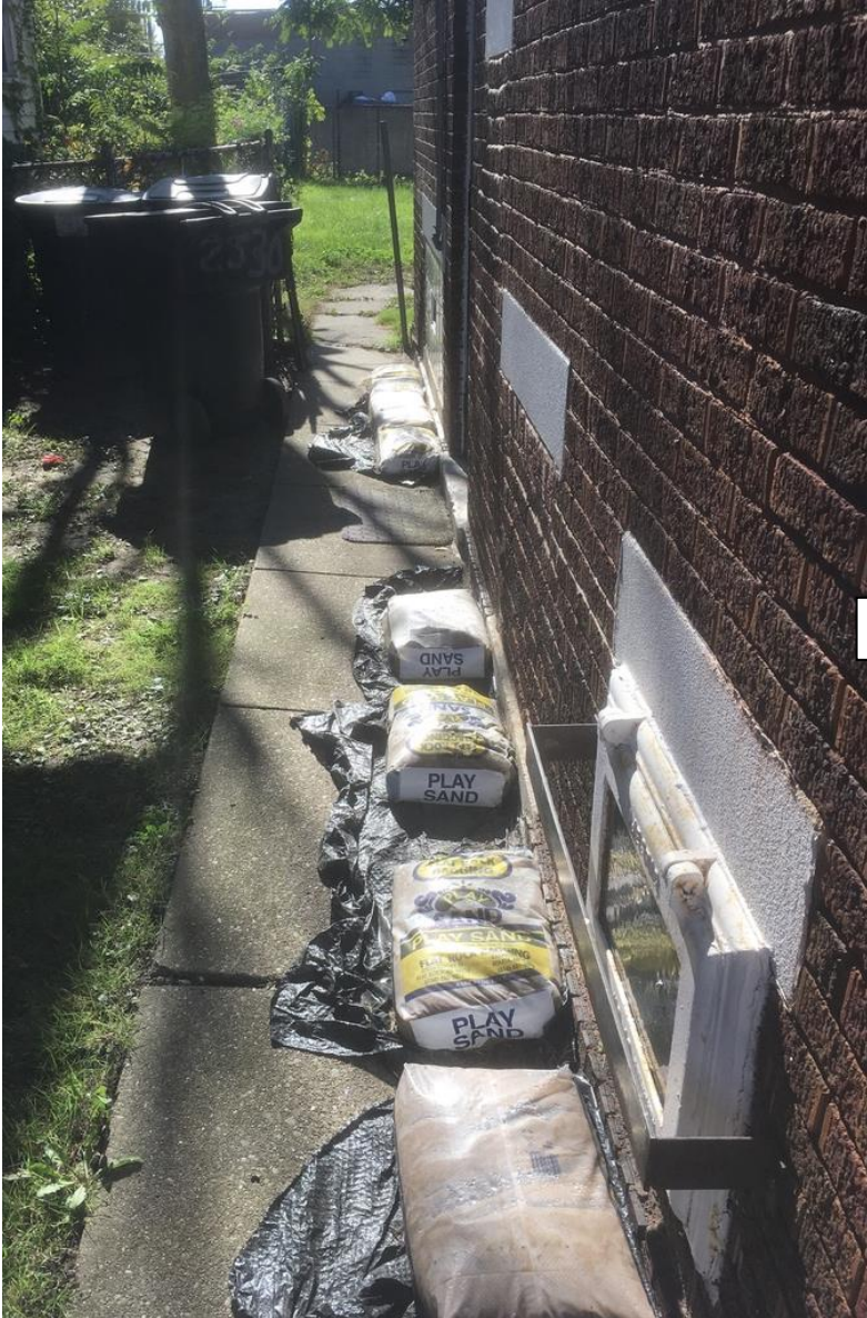
Service Walk – Damp Proofing (left)
